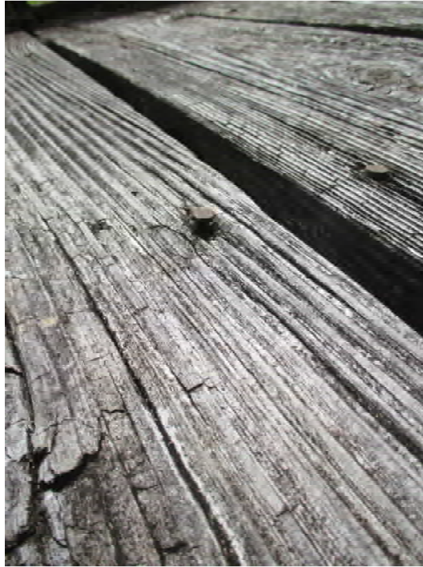
Photograph 5 Raised Nail Heads
