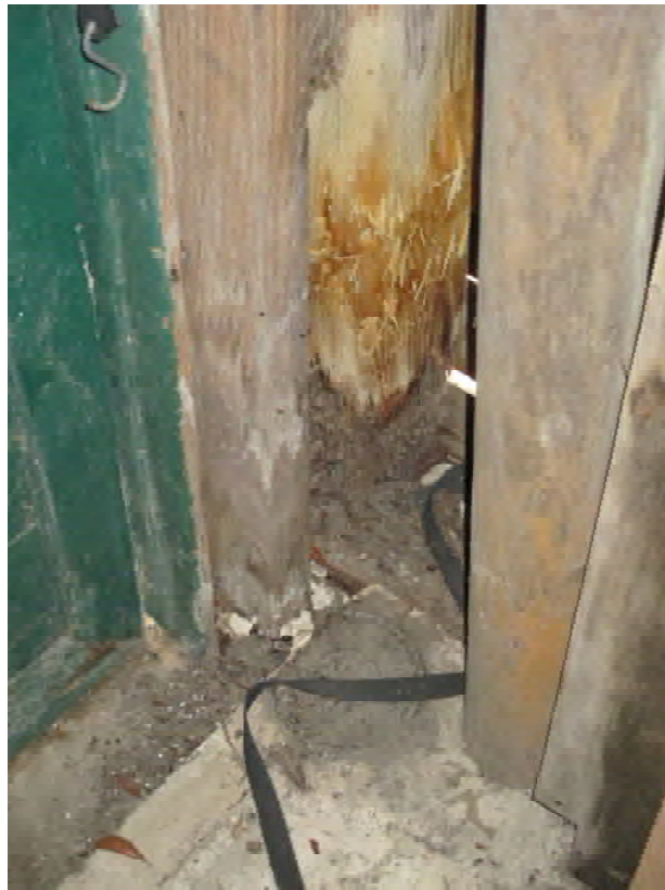
Photograph 5 Deteriorated Corner Column
