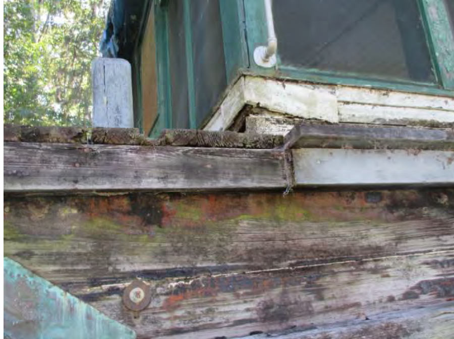
Photograph 11 Decking and Trim Deteriorated with Corroded Fasteners
