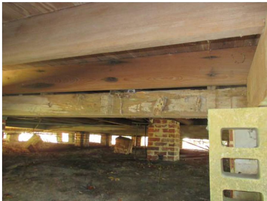
Photograph 15 Rotated and Settled Foundation Piers
