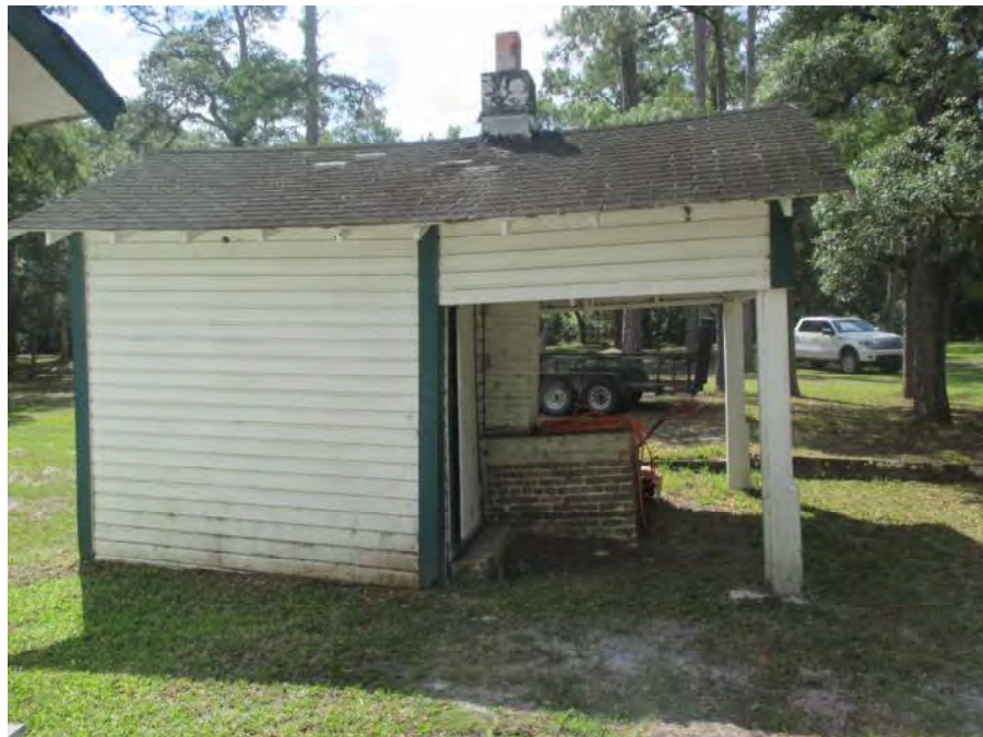
Photograph 2 Settled and Hinging Structural Framing
