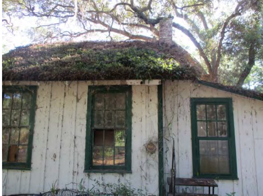
Photograph 2 Biological Growth on the Roof
