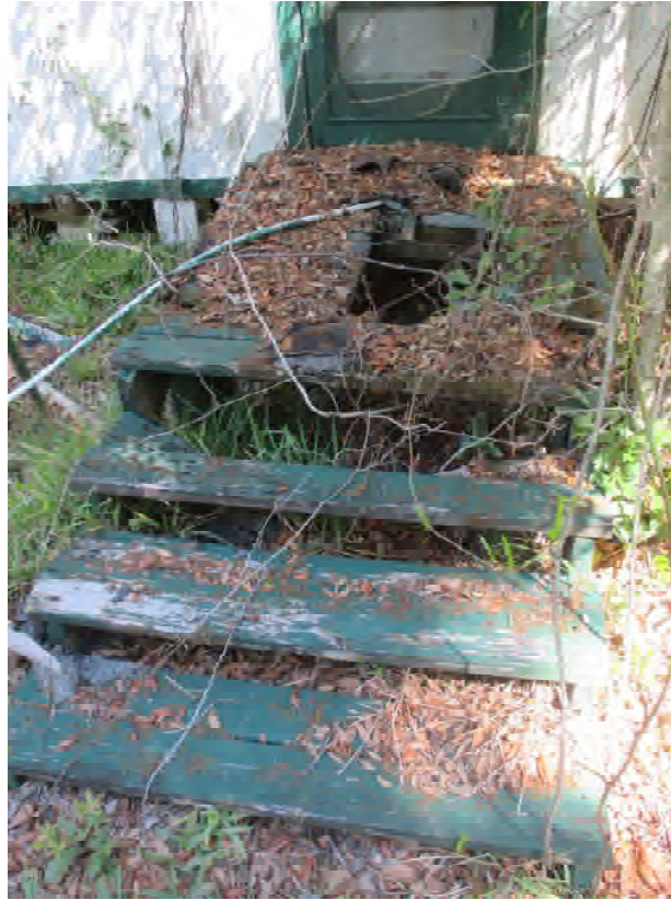
Photograph 14 Failed Rear Porch Entry Steps
