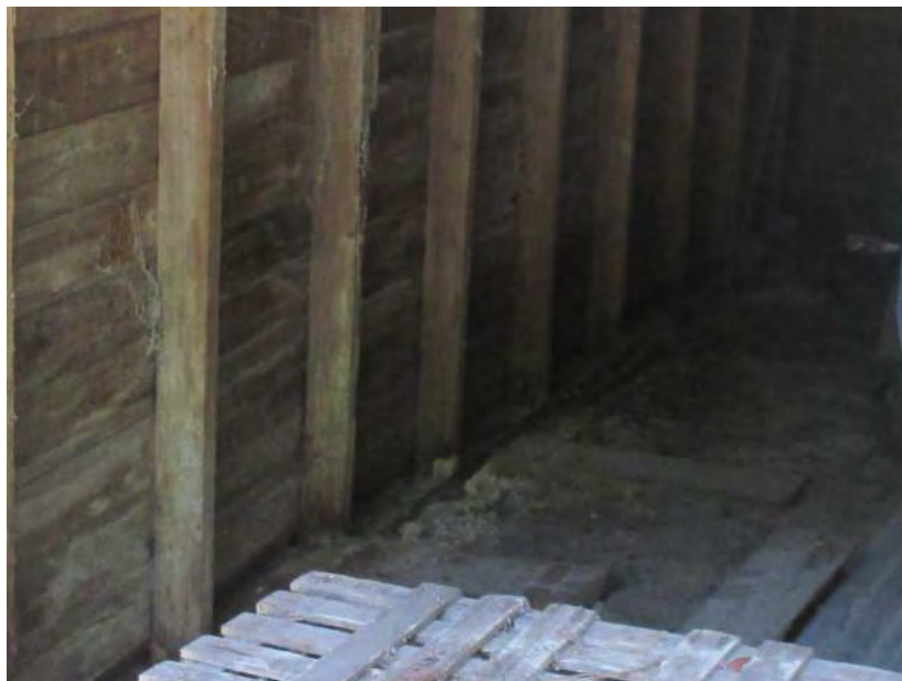
Photograph 10 Base of Wall Studs Deteriorated
