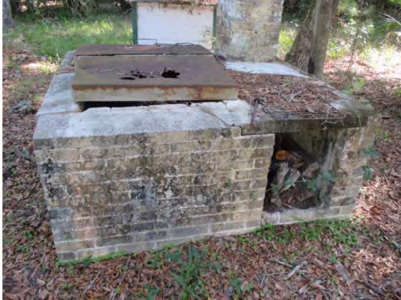
Photograph 4 Settling of Northwest Corner
