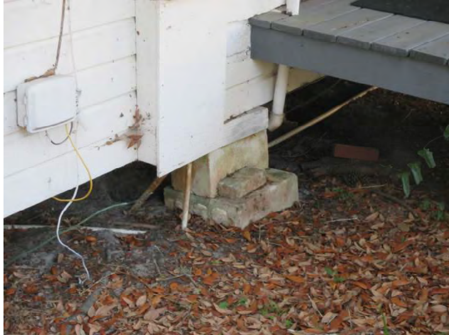
Photograph 18 Dry-Stacked and Unstable CMU Pier
