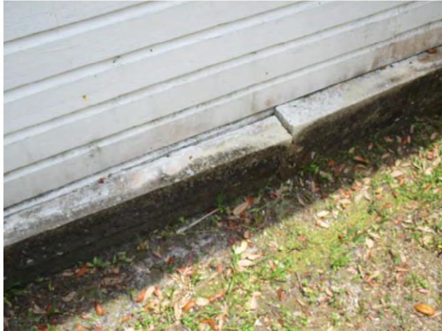
Photograph 6 Vertical and Horizontal Foundation Displacement
