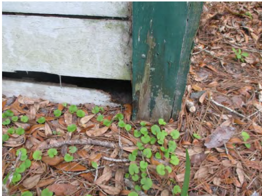
Photograph 4 Deteriorated Trim and Siding
