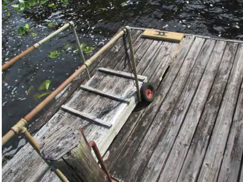
Photograph 9 Deteriorated Decking at Pivot Ramp
