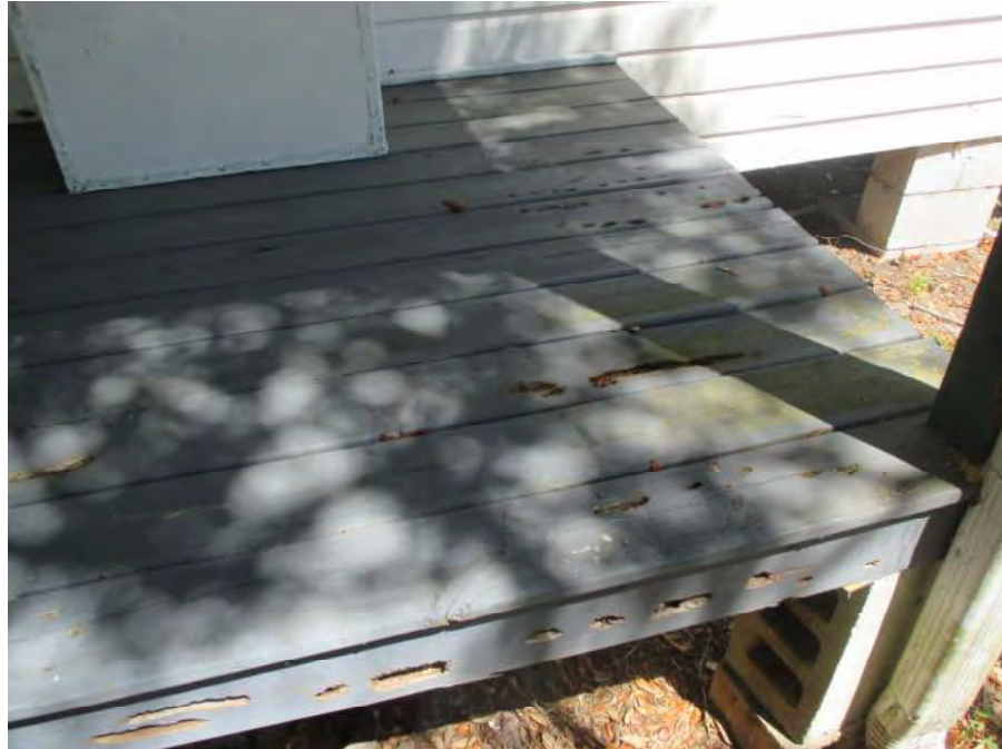
Photograph 12 Termite Damaged Floor Decking of Rear Porch Entry
