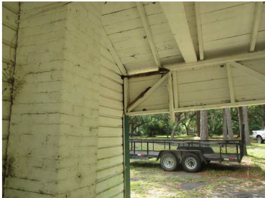
Photograph 14 Deteriorated Porch Framing
