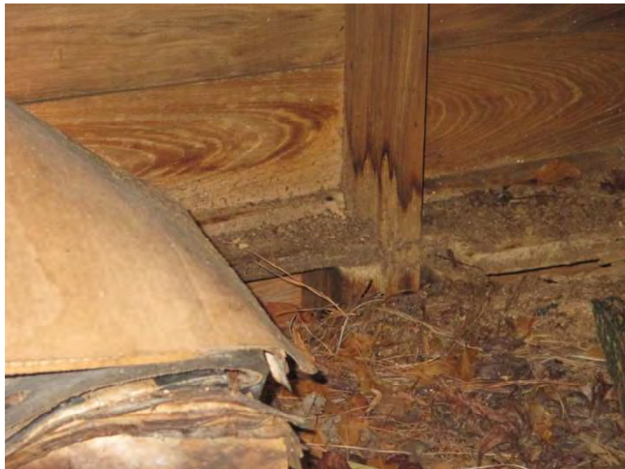
Photograph 6 Deteriorated Wall to Second-Floor Intersection
