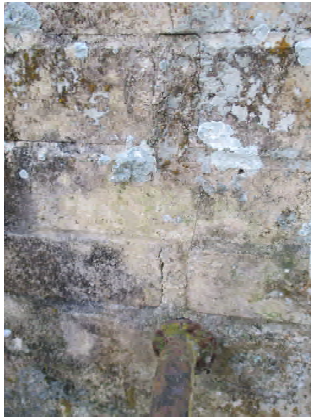
Photograph 3 Vertical Crack in Clay Brick
