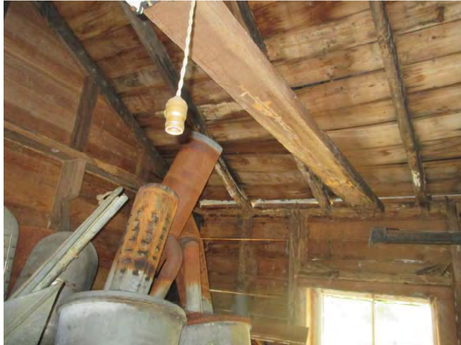
Photograph 5 Severely Deteriorated Wall and Roof Framing
