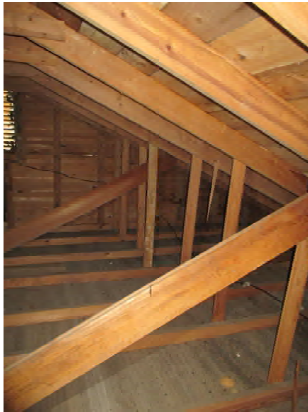
Photograph 5 Missing Diagonals within Attic
