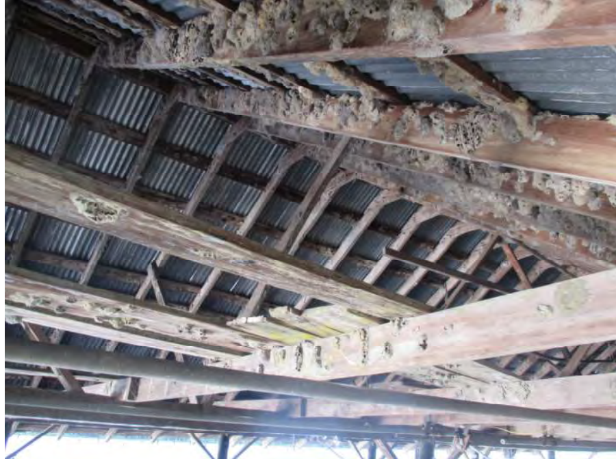
Photograph 5 Roof Rafters Covered in Mud Dauber Nests
