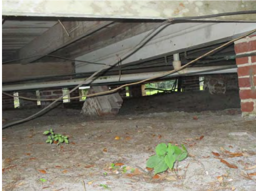
Photograph 16 Rotated and Settled Foundation Piers
