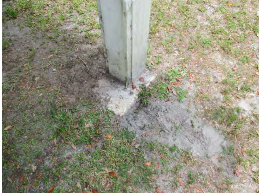
Photograph 15 Settled Column Foundation
