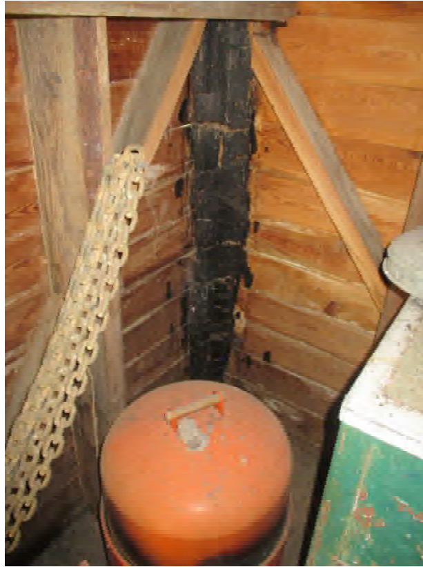
Photograph 9 Charred and Termite Damaged Column
