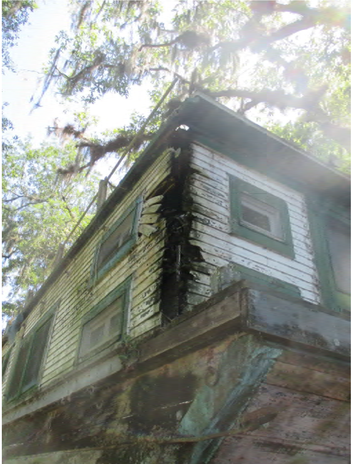
Photograph 3 Northwest Corner Severely Deteriorated
