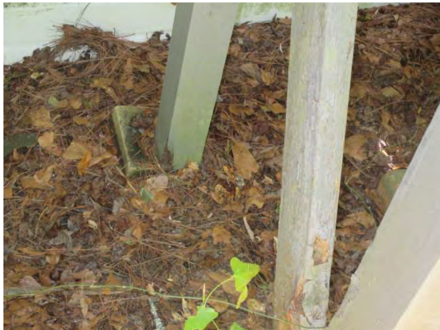
Photograph 14 Stair Column Not on Stable Foundation
