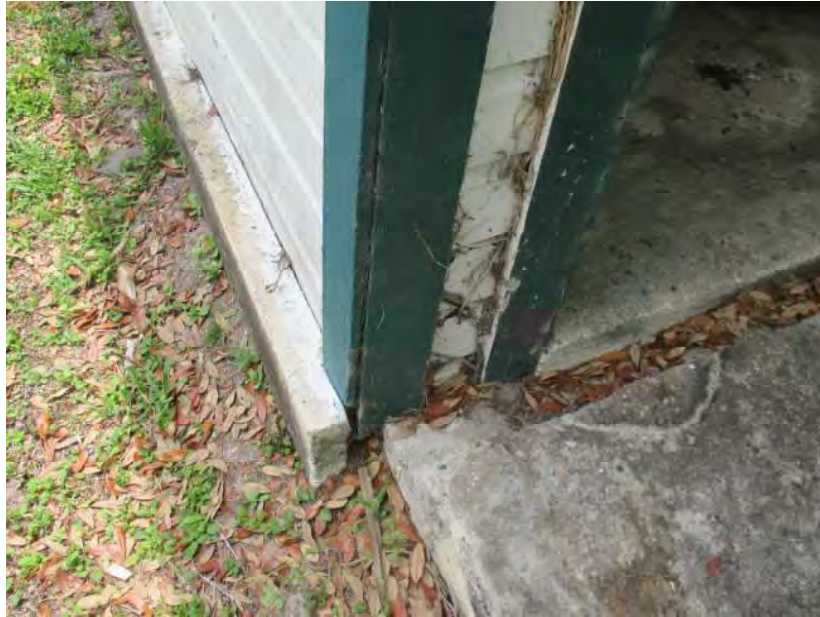
Photograph 8 Hinged Concrete Entry Ramp to Interior Slab
