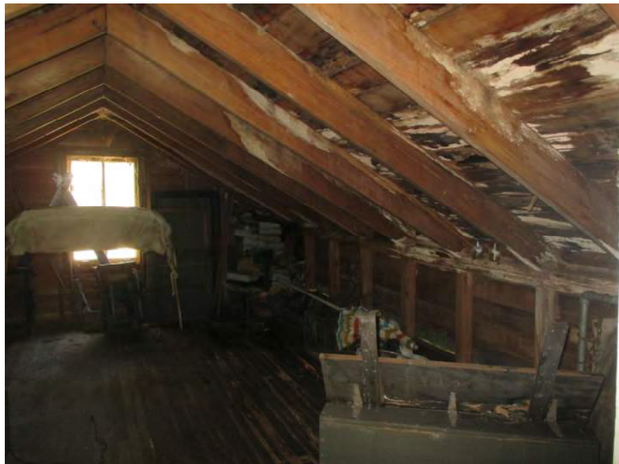
Photograph 2 Deteriorated Roof and Wall Framing
