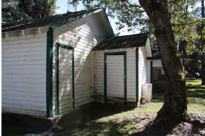
Rear of the Double Garage with deterioration on the rear addition.
