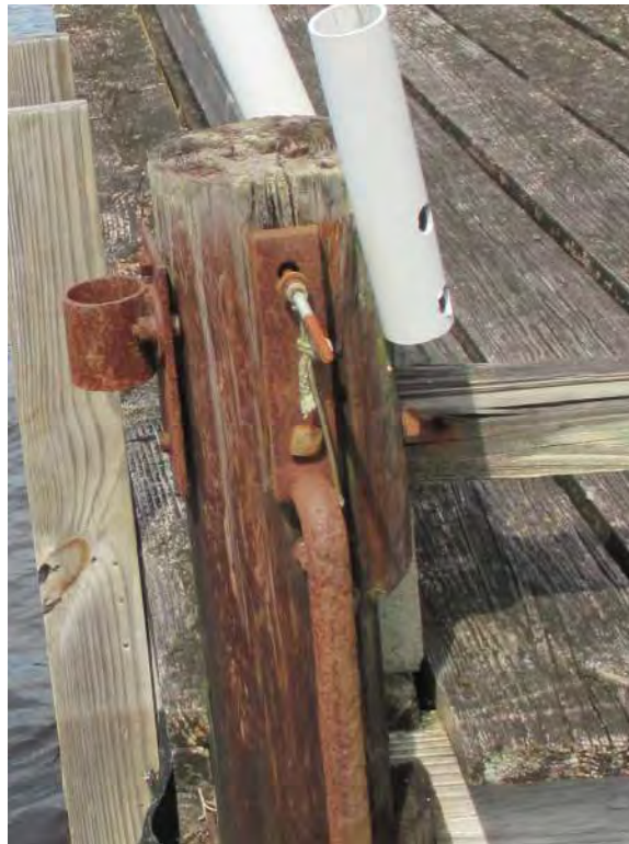
Photograph 10 Corroded and Missing Hardware
