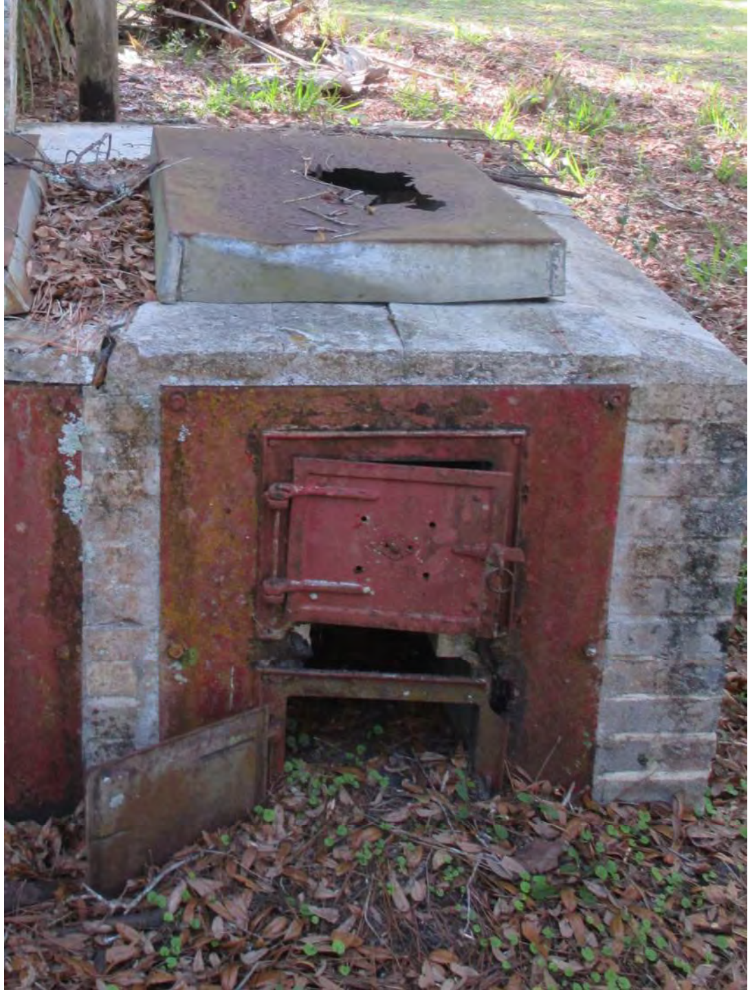
Photograph 6 Deteriorated Access Doors and Settled Corner
