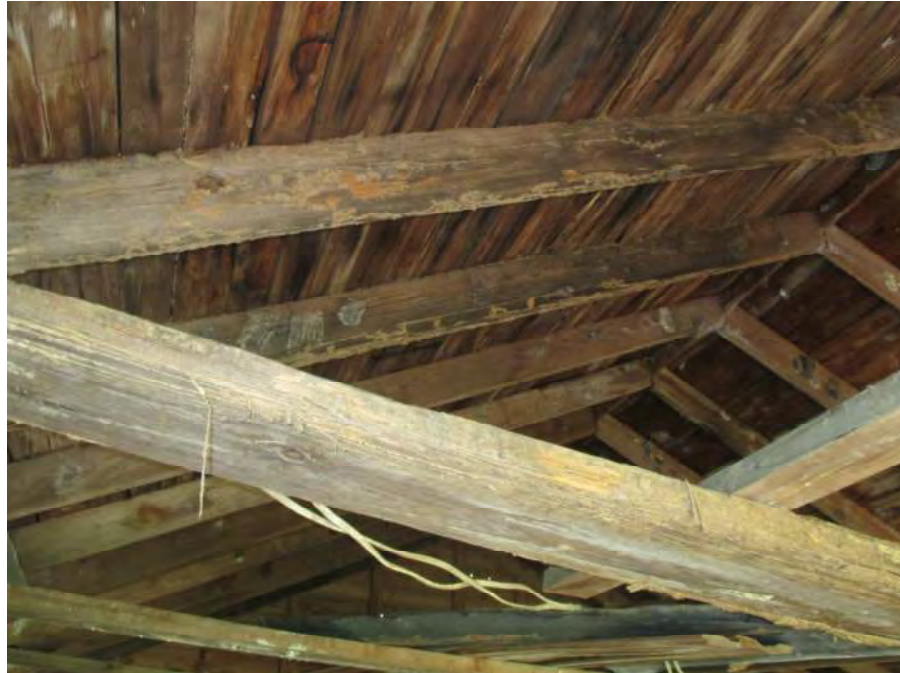
Photograph 2 Deteriorated Roof Rafters
