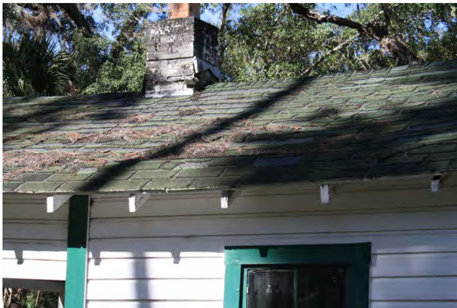
Fryer Shed chimney. Deteriorated and needs restoration.
