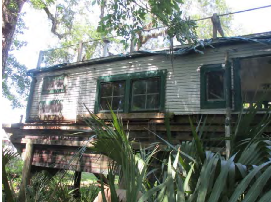
Photograph 13 Missing and Severely Deteriorated Siding
