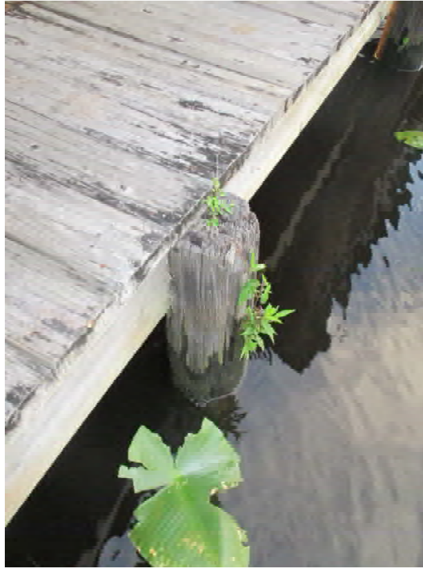
Photograph 11 Deterioration at Top of Timber Pile
