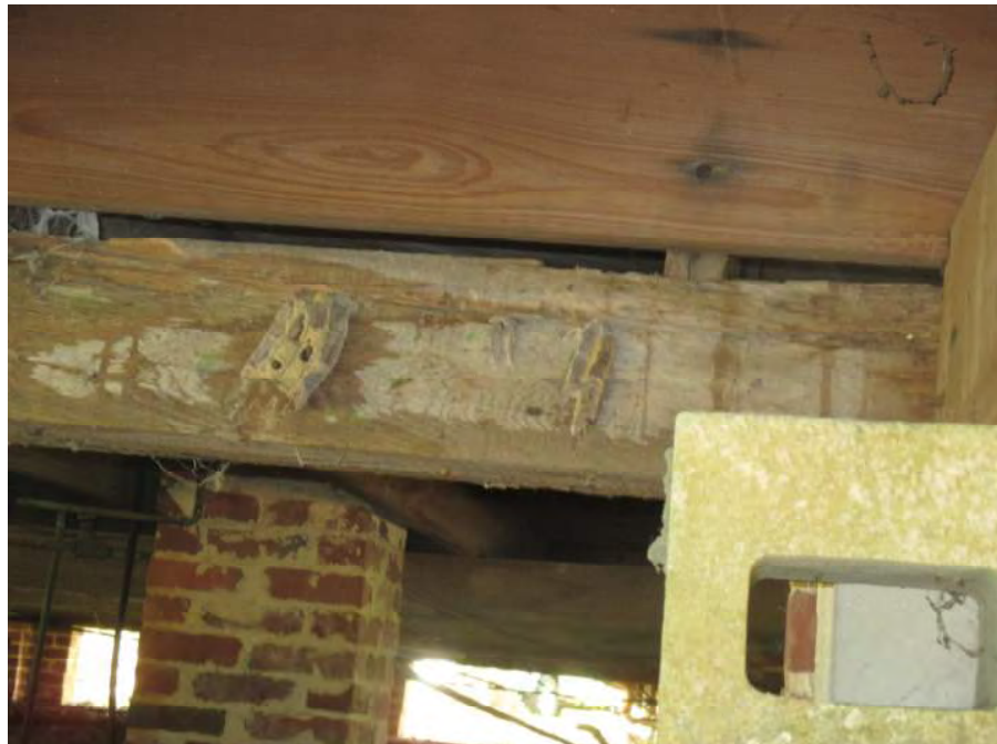
Photograph 11 Weathered Floor Framing
