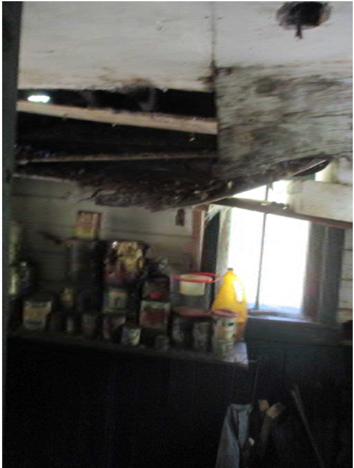
Photograph 6 Collapsed Roof Framing and Ceiling Due to Moisture
