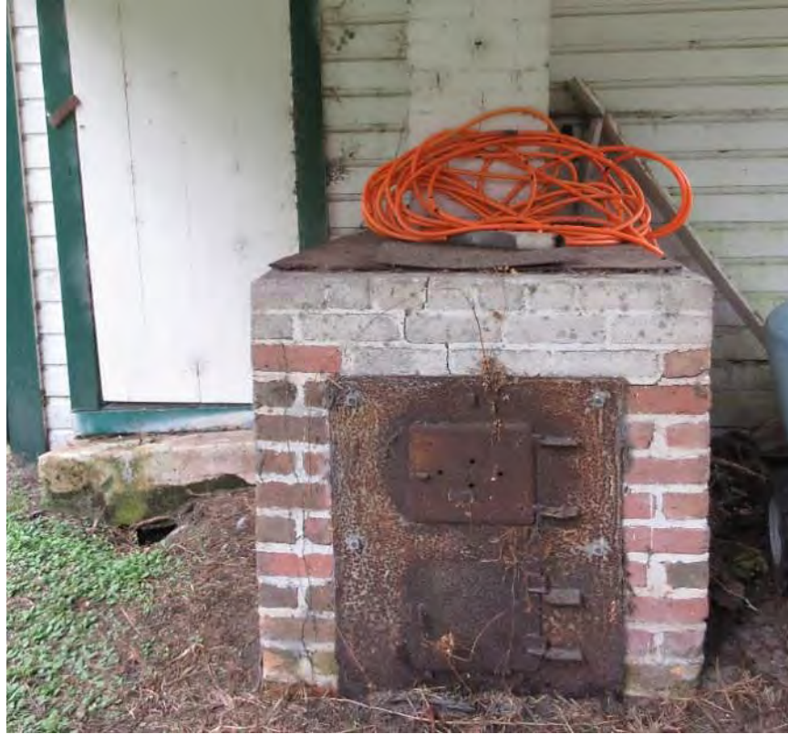
Detail of the fryer stove.
