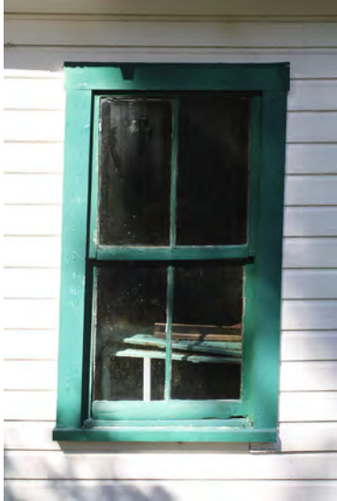
Fryer Shed window with deterioration.
