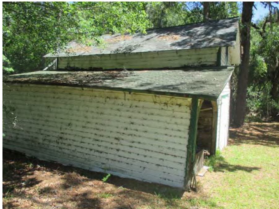
Photograph 12 Corner Racked and Settled
