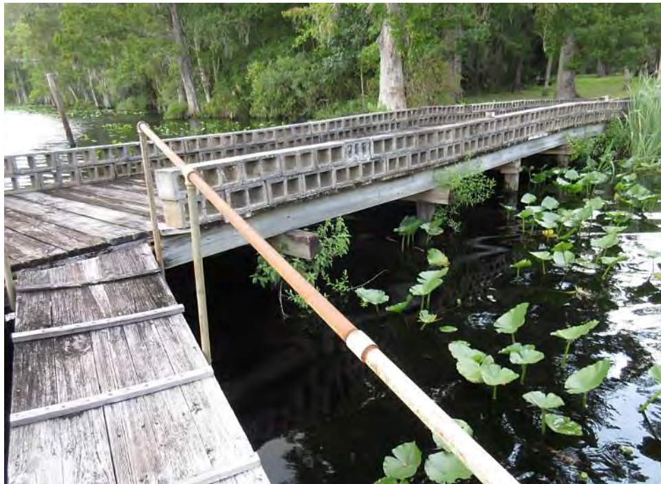
View east from the floating dock toward the fixed finger of the Dock.
