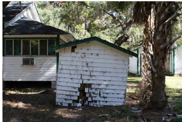
Woodshed for the Main House has lost shingles and is falling into the ground due to no foundation.
