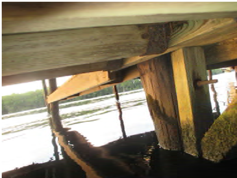
Photograph 8 Joist Hangers Deteriorated
