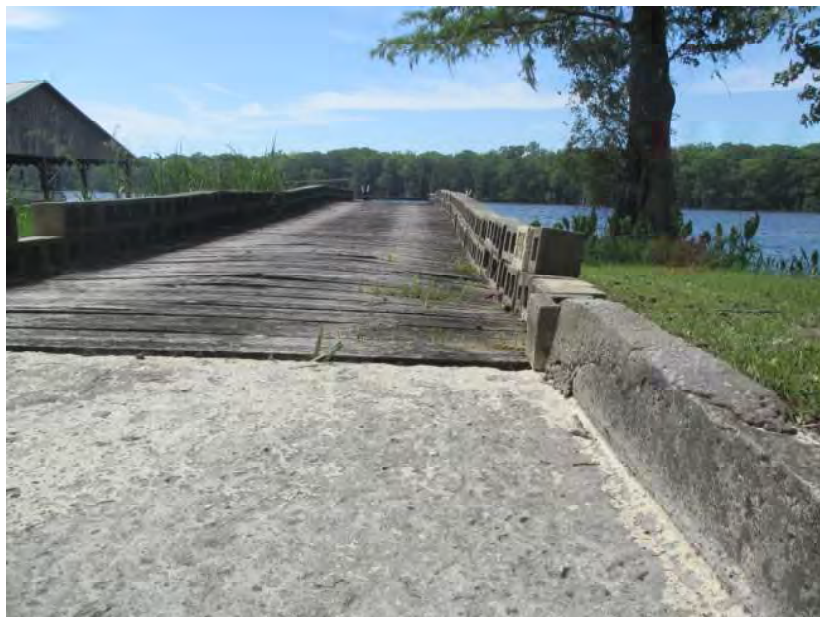
Photograph 6 Settlement of Dock Structure
