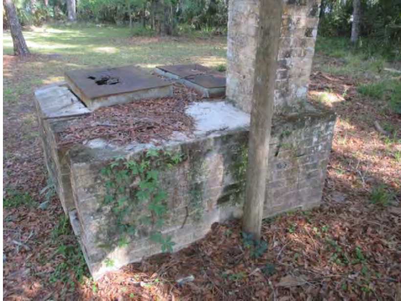
Photograph 2 Biological Growth and Vegetation on Outdoor Grill
