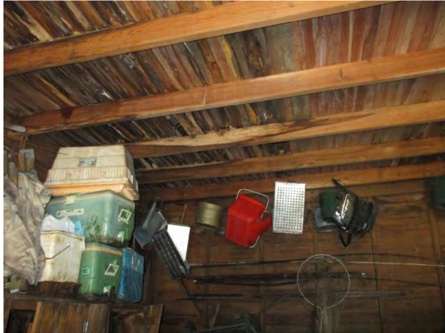
Photograph 5 Deteriorated Floor Framing and Decking
