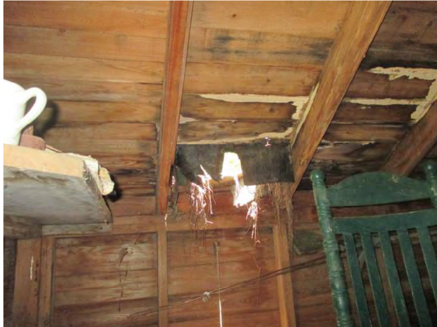
Photograph 3 Deteriorated Roof Framing and Sheathing
