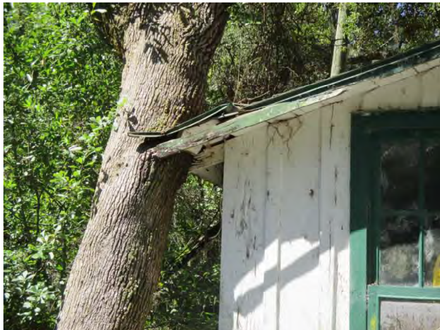
Photograph 3 Damaged Rear Corner Due to Tree
