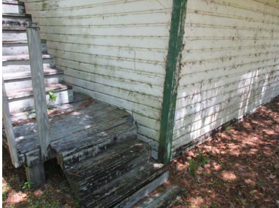
Photograph 15 Severely Deteriorated Attic Access Stair
