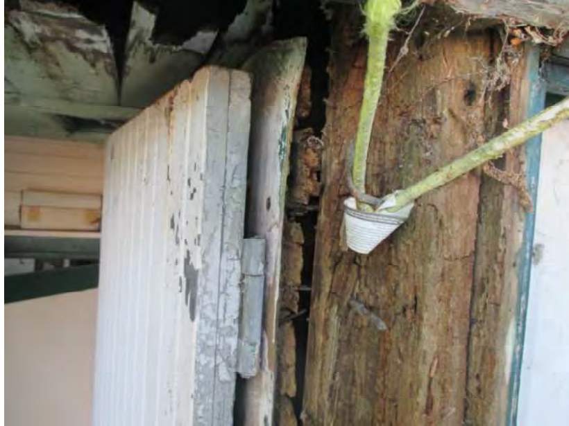
Photograph 4 North Wall and Roof Joists Severely Deteriorated
