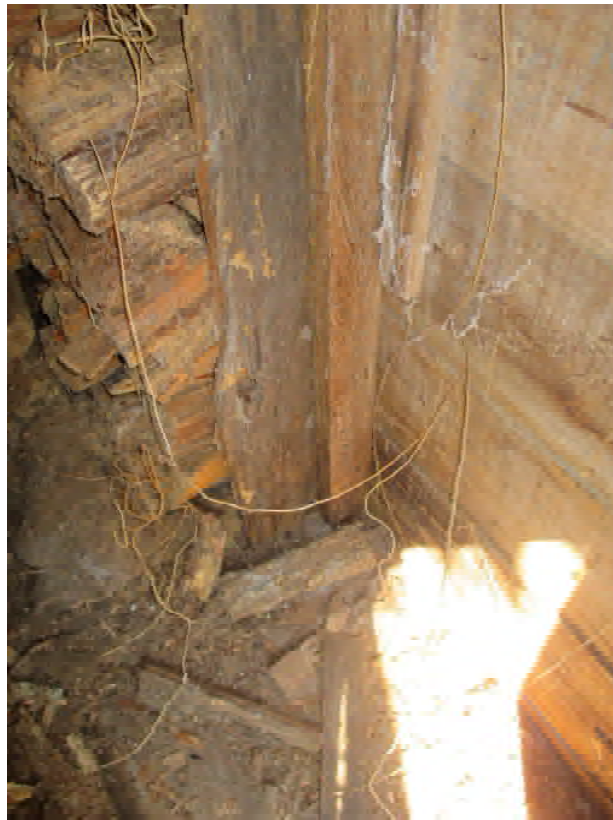
Photograph 4 Deteriorated Wall Framing and Sheathing
