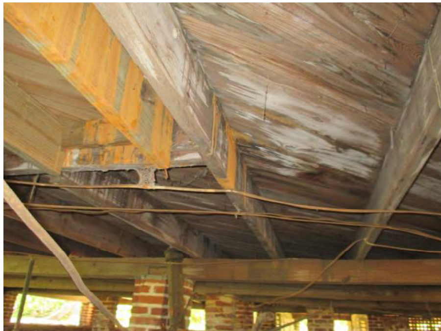
Photograph 13 Water Damaged Floor Decking
