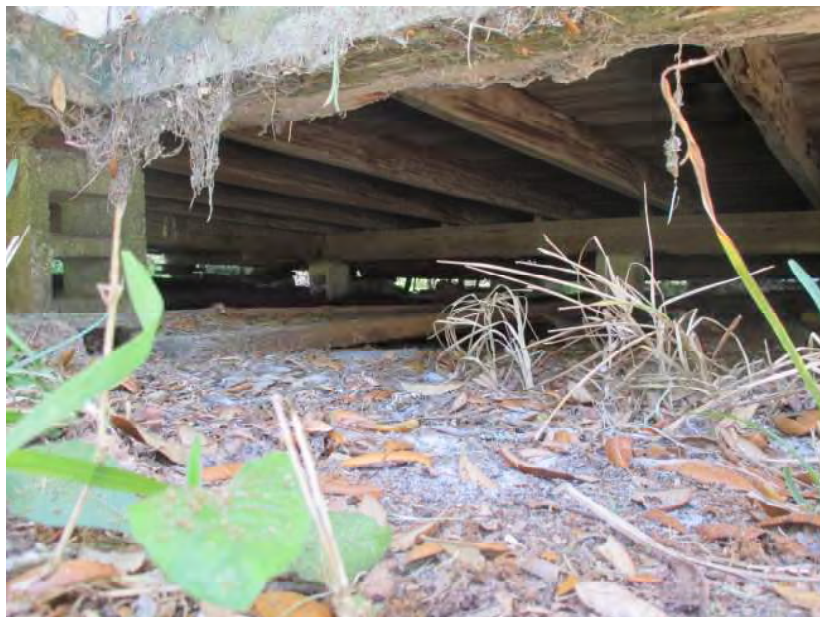
Photograph 5 Moisture or Termite Floor Framing Deteriorated
