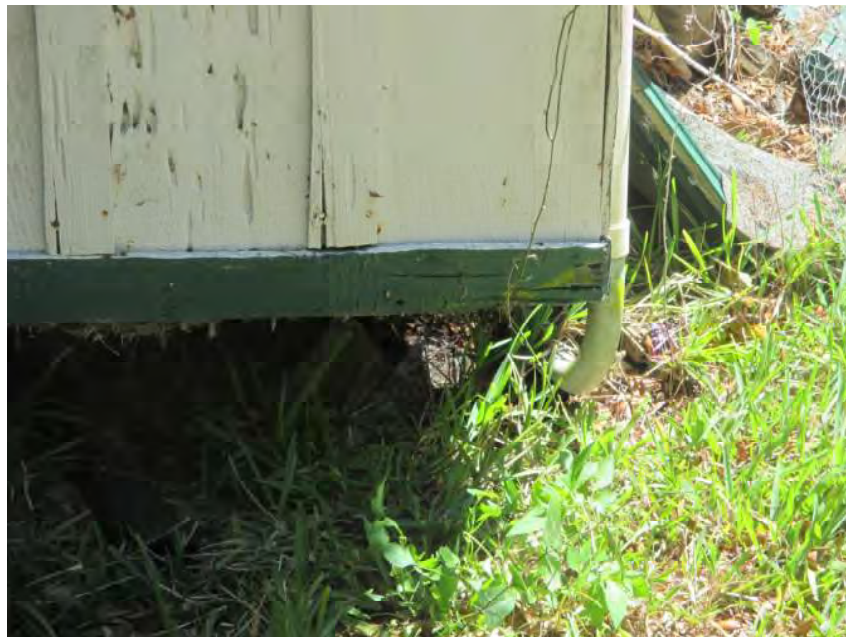
Photograph 13 Failed Corner Foundation
