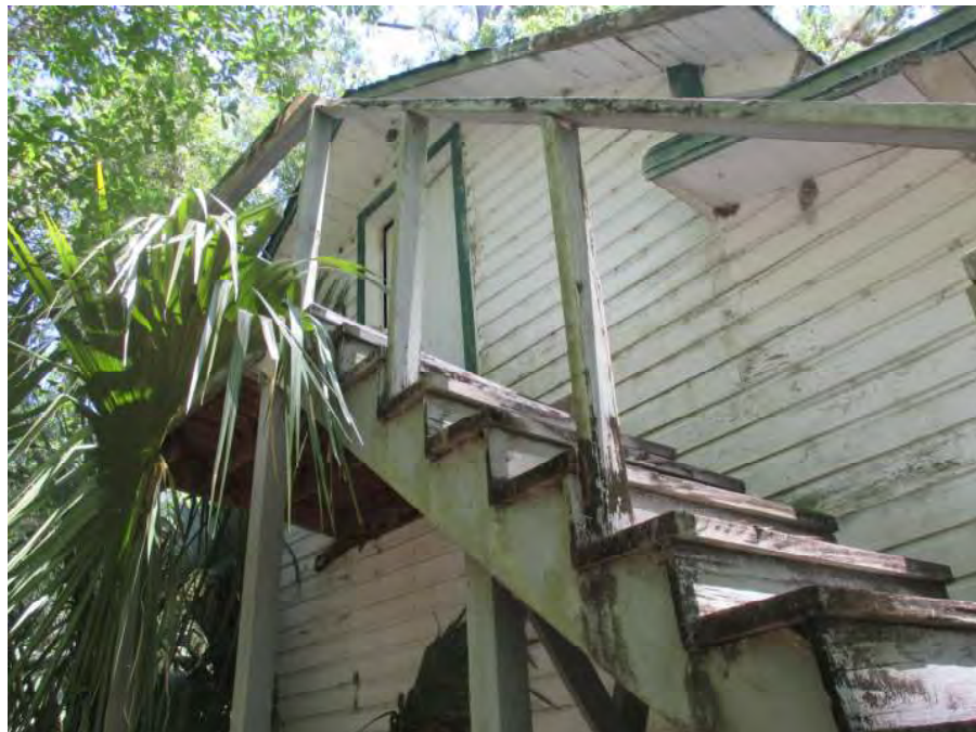
Photograph 16 Severely Deteriorated Attic Access Stair
