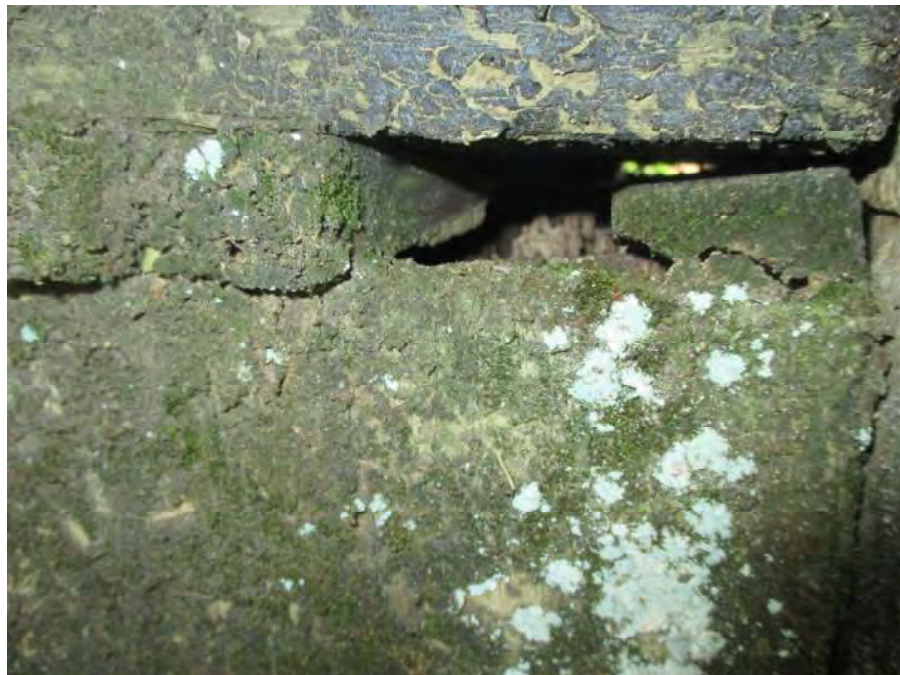
Photograph 16 Top of Houseboat Support Pile Deteriorated
