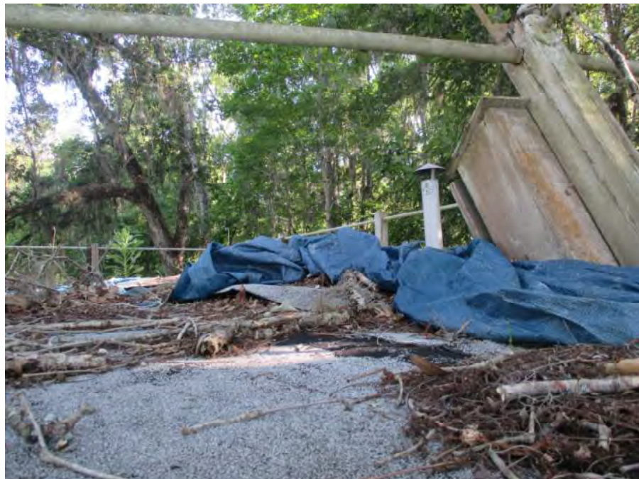
Photograph 2 Roof Tarp and Debris on Roof
