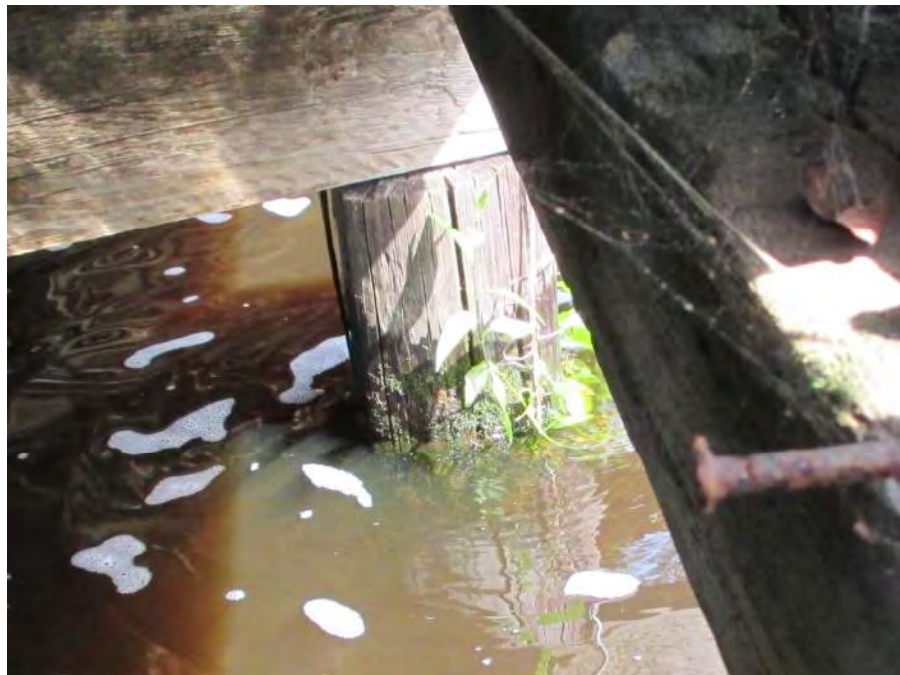
Photograph 8 Biological Growth and Weather Checking at Base of Timber Column
