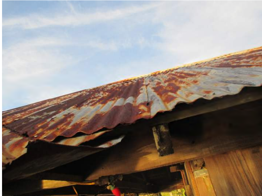
Photograph 3 Surfacial Rust on Metal V-Crimp Roofing
