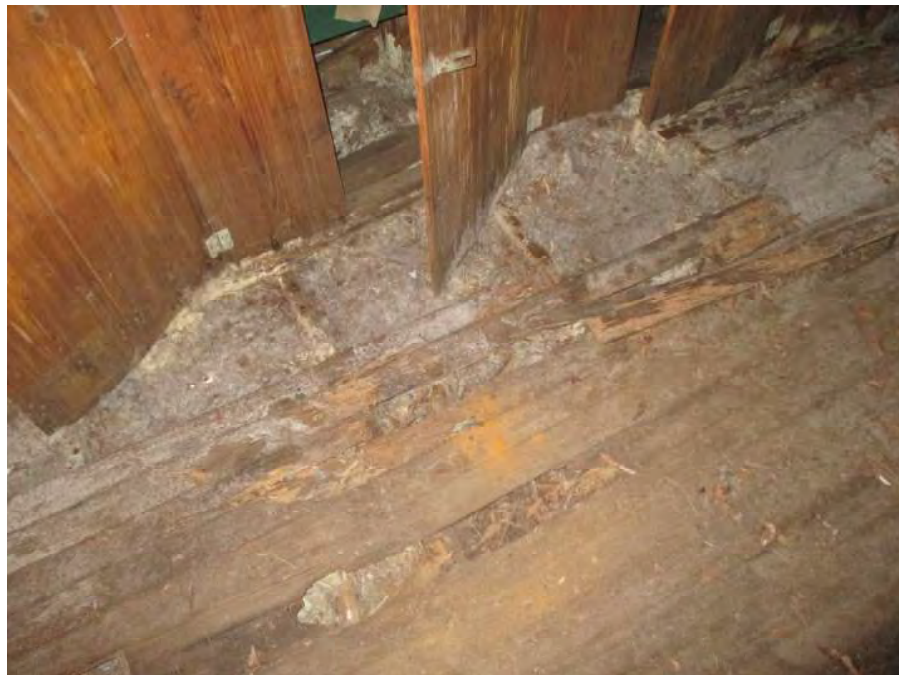
Photograph 8 Deteriorated Floor Decking and Framing Bearing on Grade
