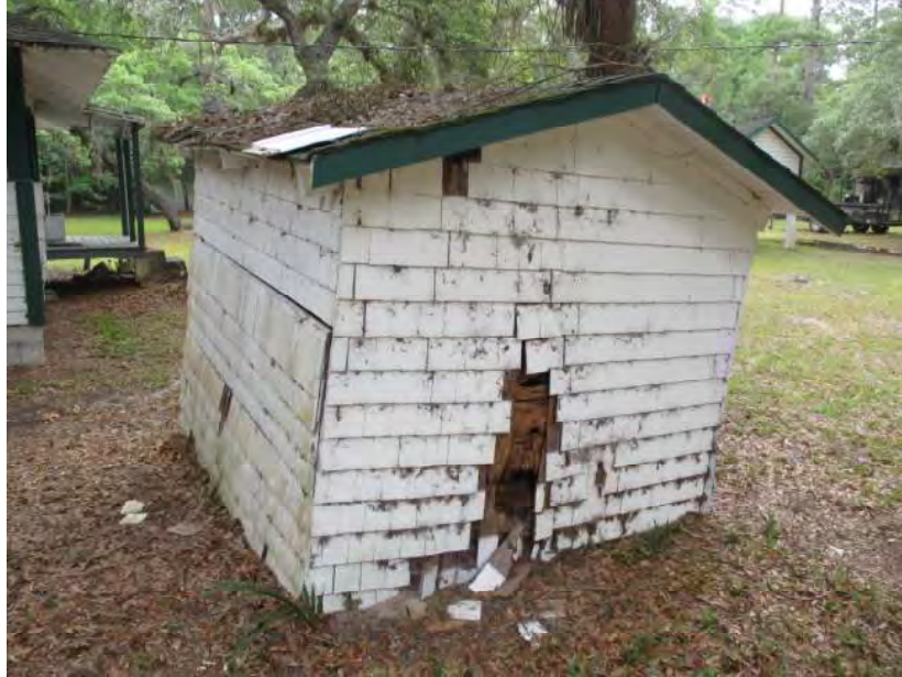
Photograph 3 Severely Deteriorated Wall Sheathing and Siding
