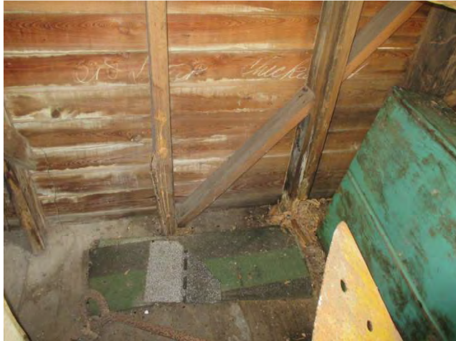
Photograph 11 Severely Deteriorated Wall Framing
