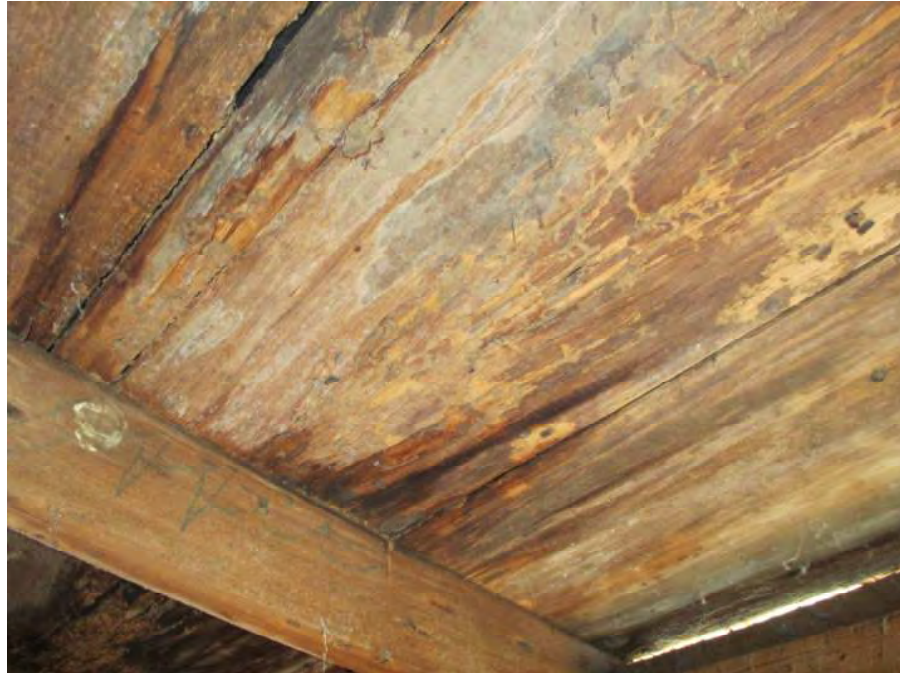
Photograph 5 Deteriorated Roof Sheathing
