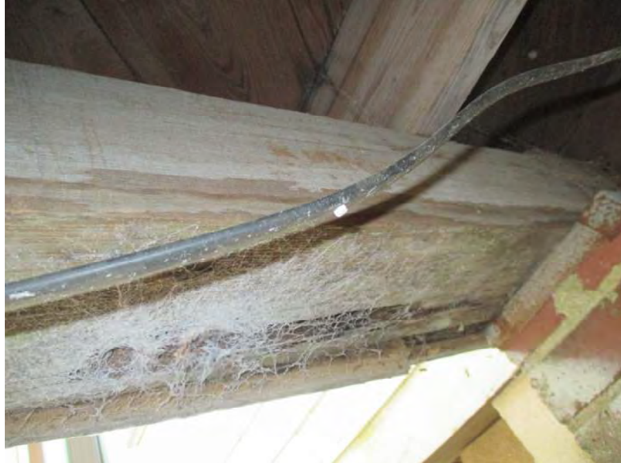
Photograph 10 Termite Damaged Floor Framing
