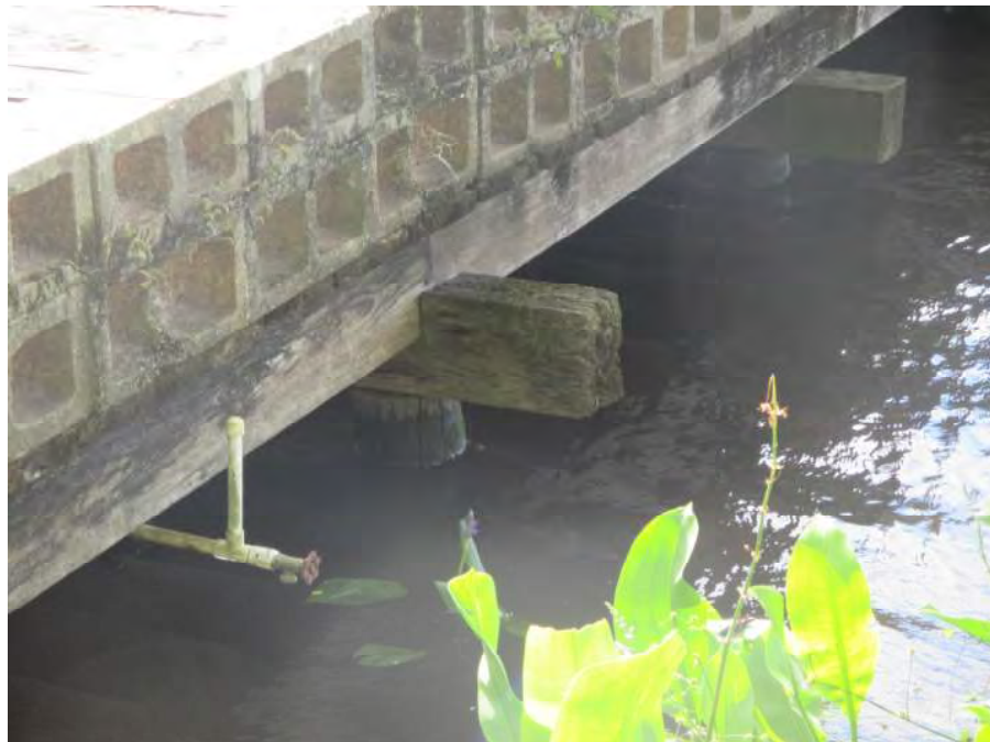
Photograph 2 Deteriorated Beam End Cantilevered Over Timber Pile
