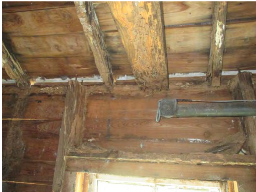
Photograph 6 Severely Deteriorated Wall and Roof Framing
