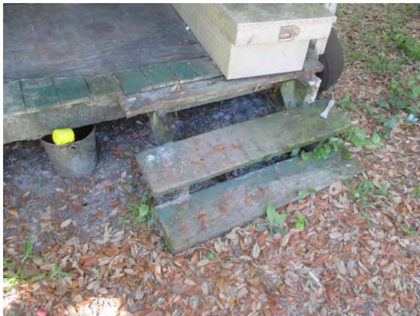
Photograph 15 Rotated and Deteriorated Main Entry Steps
