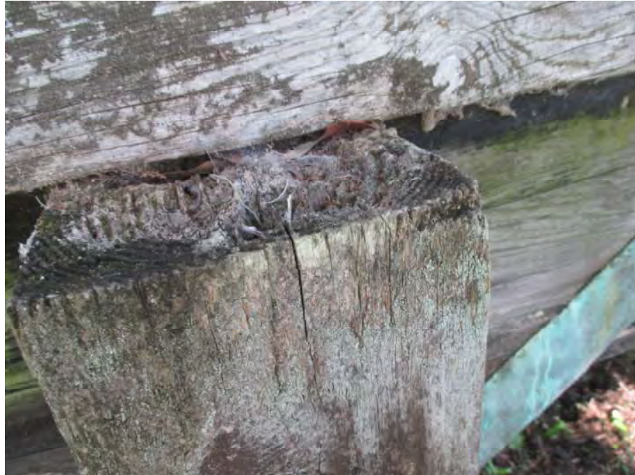
Photograph 15 Top of Houseboat Support Pile Deteriorated
