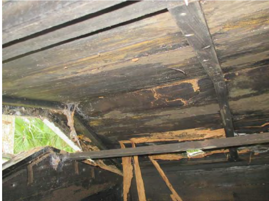
Photograph 3 Deteriorated Roof Sheathing and Framing
