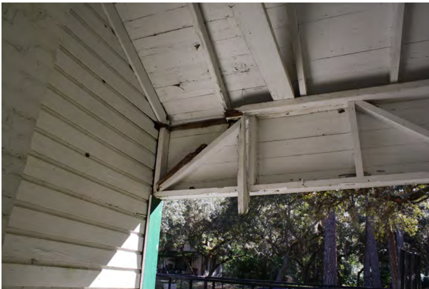
Fryer Shed plate deterioration.
