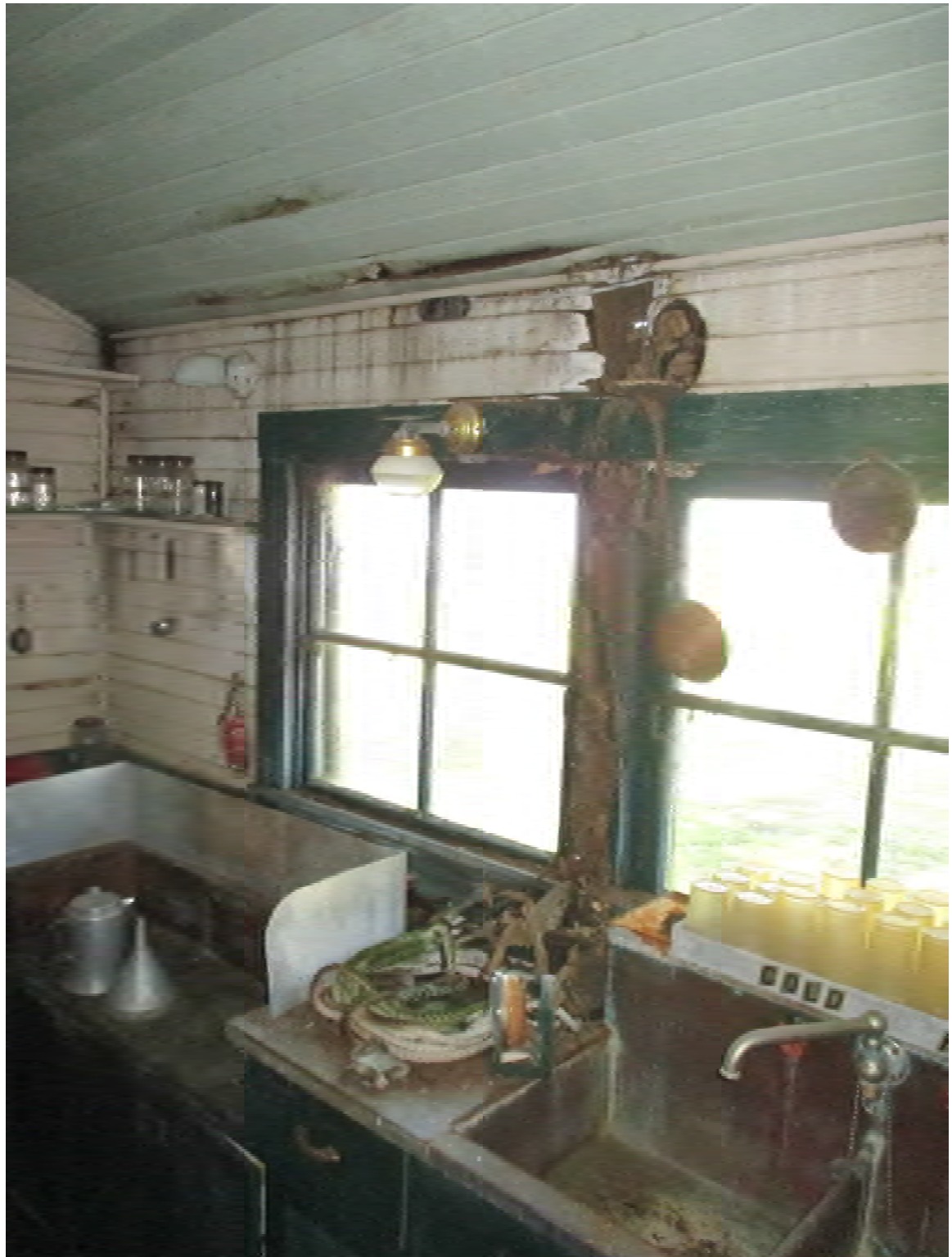
Photograph 7 Wall Framing and Siding Severely Deteriorated
