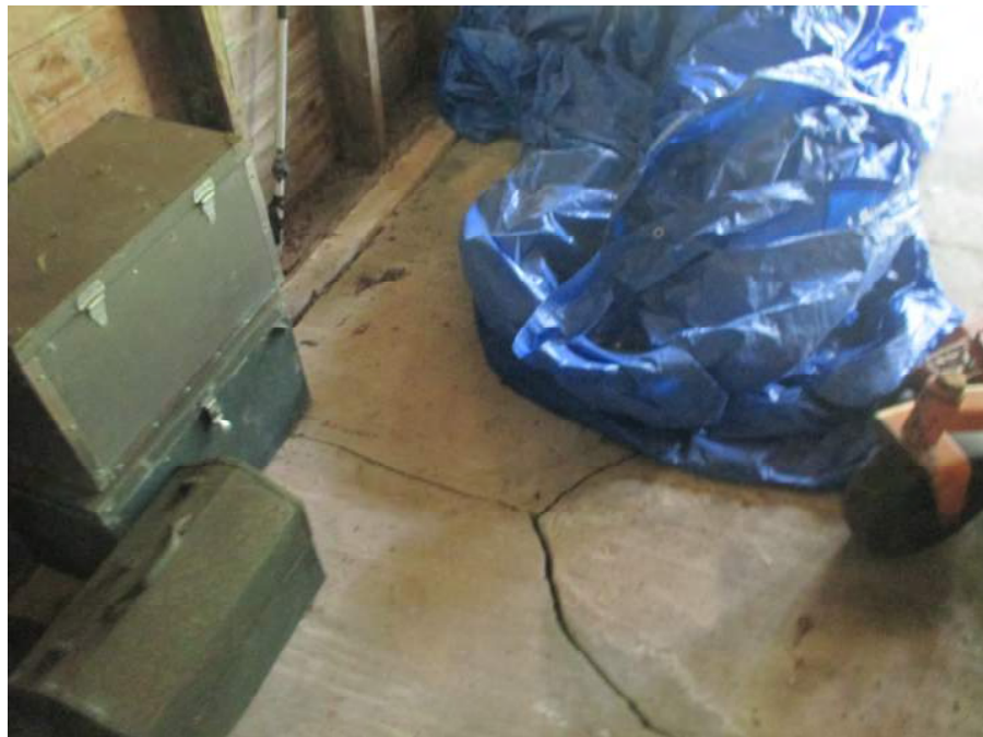
Photograph 7 Vertical and Horizontal Slab Displacement
