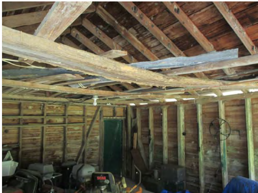
Photograph 3 Termite Damaged Framing
