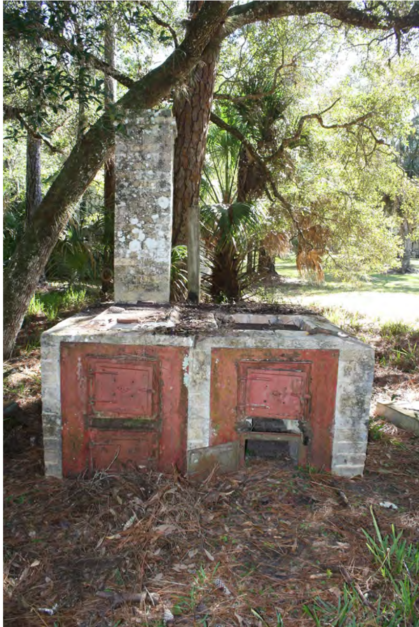
North side elevation of the grill. Note that some components will need restoration, including the concrete top.
