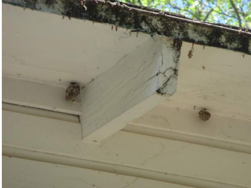
Photograph 4 Deteriorated Rafter Tail
