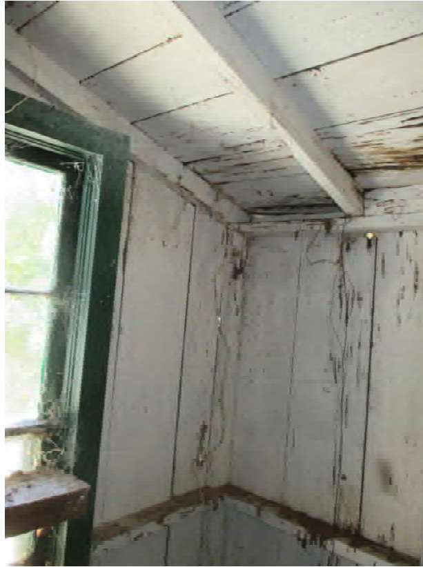
Photograph 4 Moisture Damaged Framing
