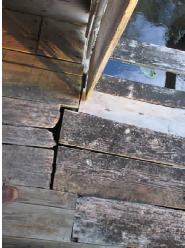
Photograph 7 Decking Deteriorated and Not Fastened
