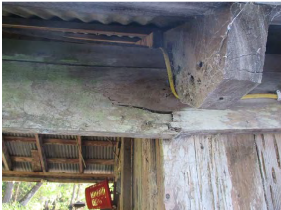
Photograph 6 Cracked Perimeter Beam
