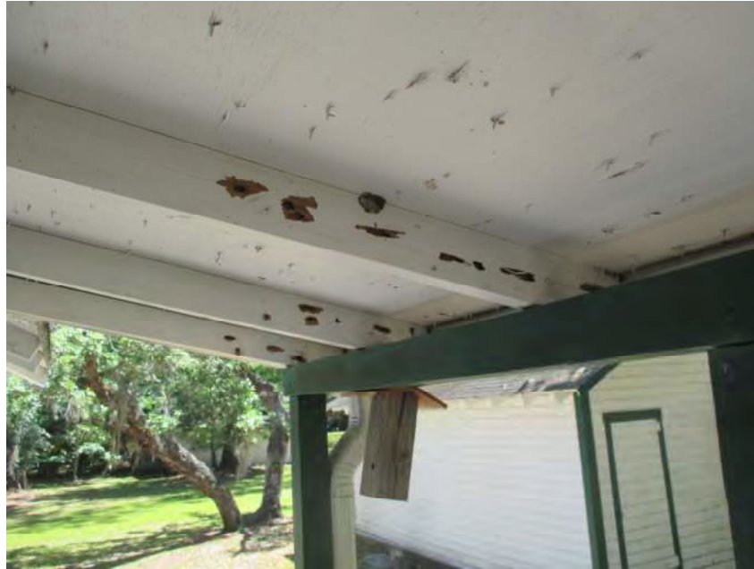
Photograph 6 Termite Damaged Rafter Tail at Rear Porch
