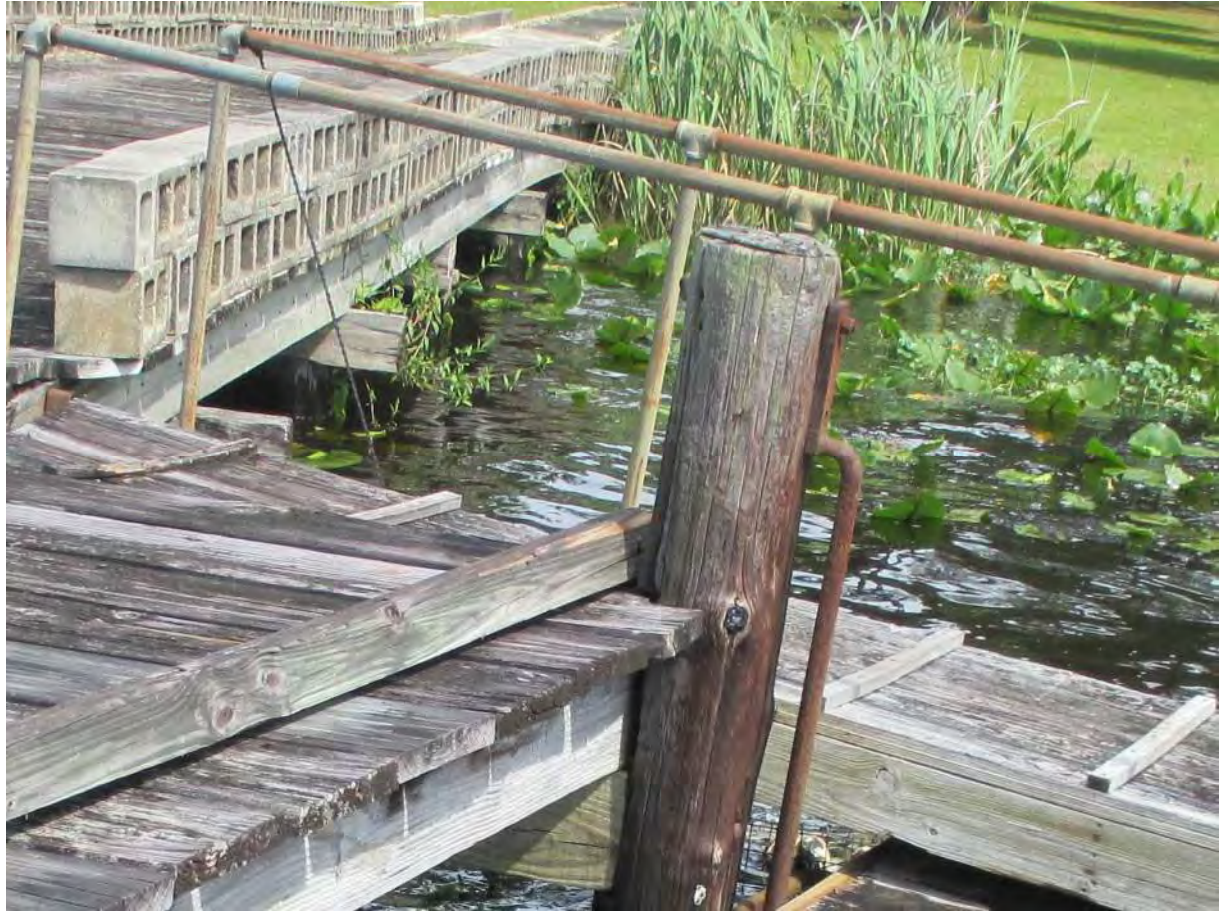
Photograph 11 Perimeter Timber Unattached
