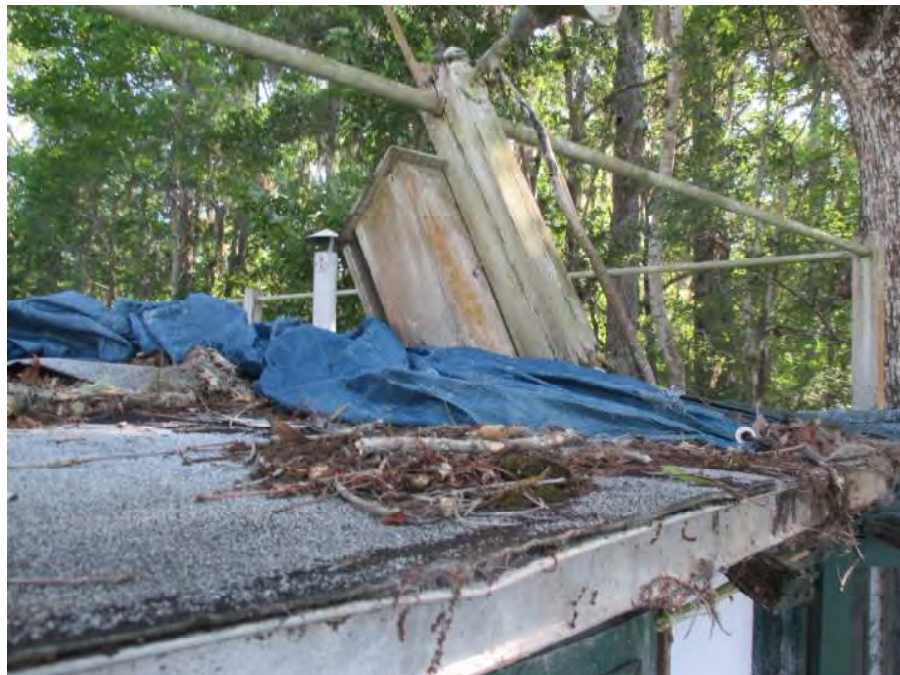
Photograph 12 Handrail Post Failed with Broken Handrail
