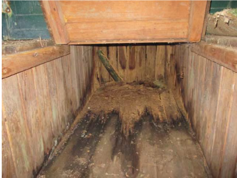
Photograph 8 Kitchen Floor Storage Well Moisture Damage
