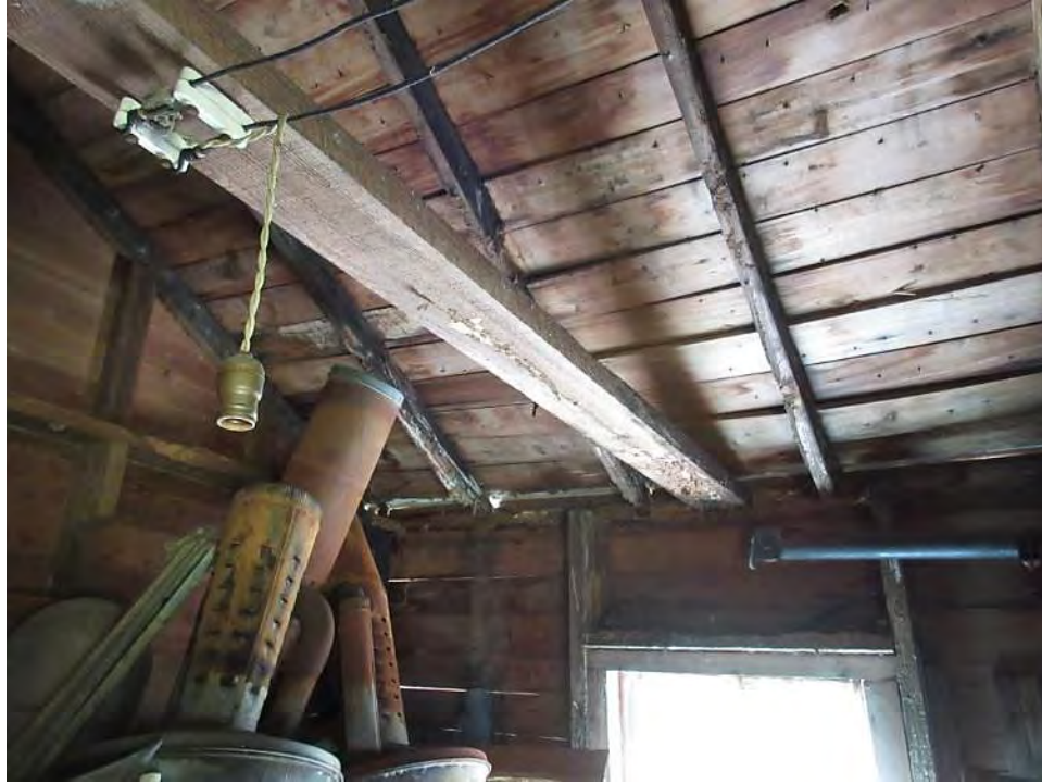
Detail of roof damage on the southern side of the interior storage area.
