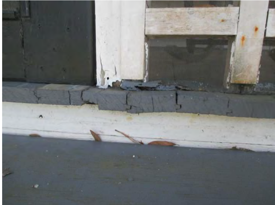
Photograph 14 Water Damaged Decking at Main Entry Porch
