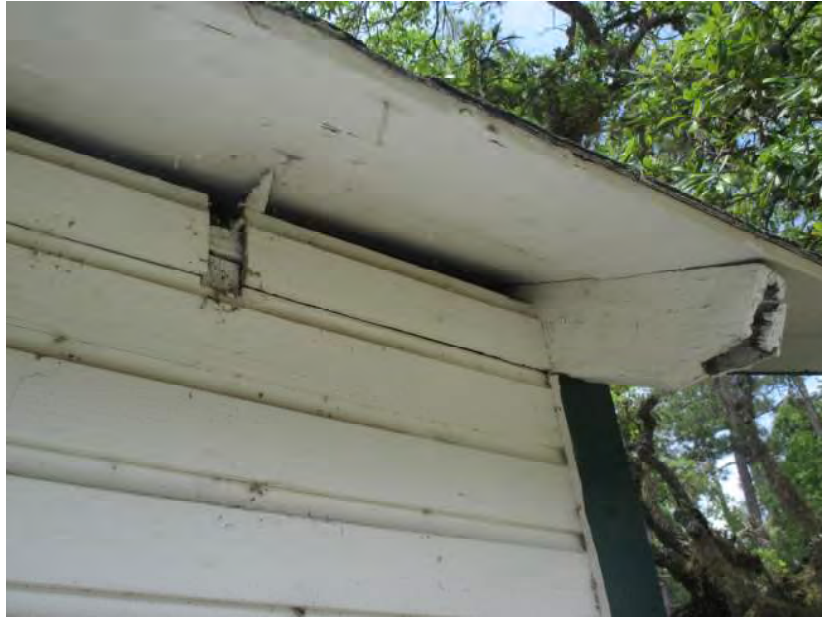
Photograph 4 Deteriorated Rafter Tails
