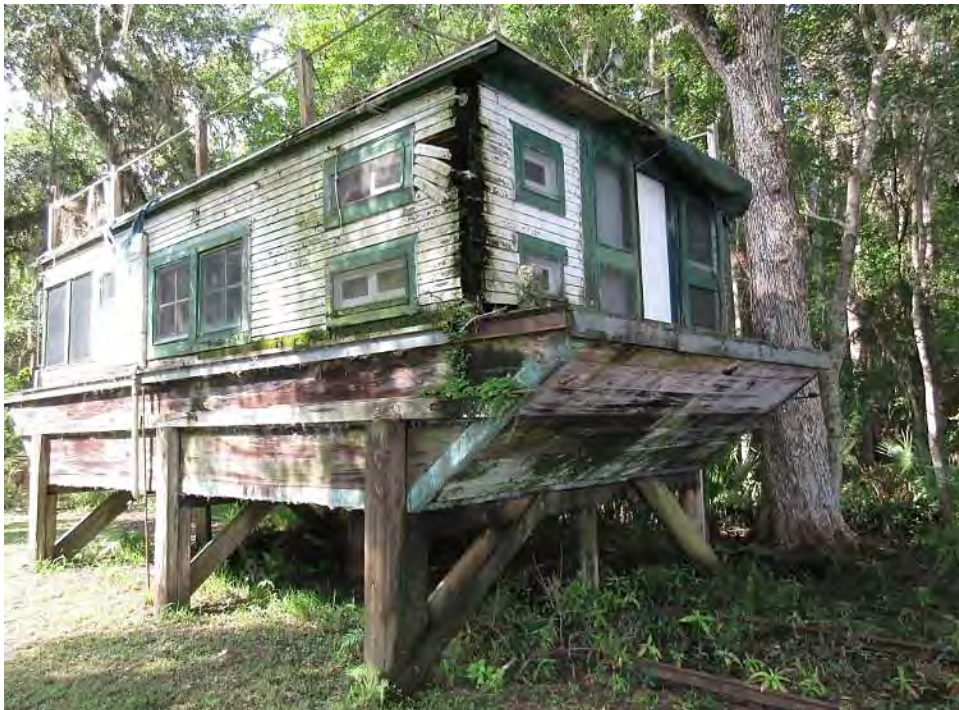
East and north sides of the Houseboat. Note wood rot damage at the northeast corner.
