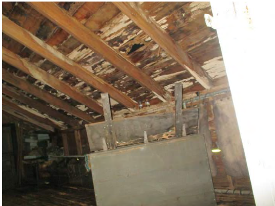
Photograph 4 Deteriorated Roof Sheathing and Framing
