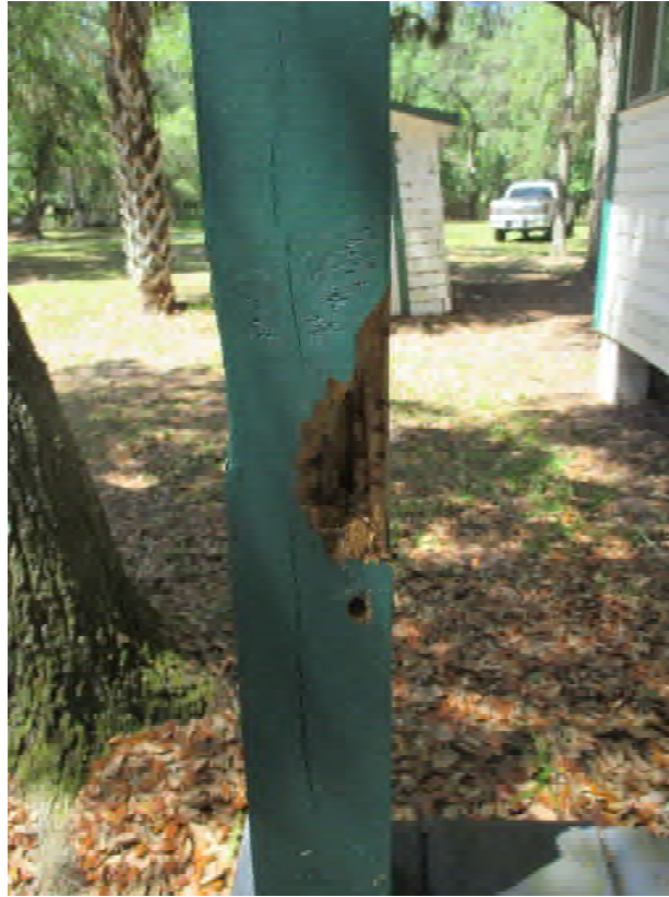
Photograph 8 Termite Damaged Porch Column
