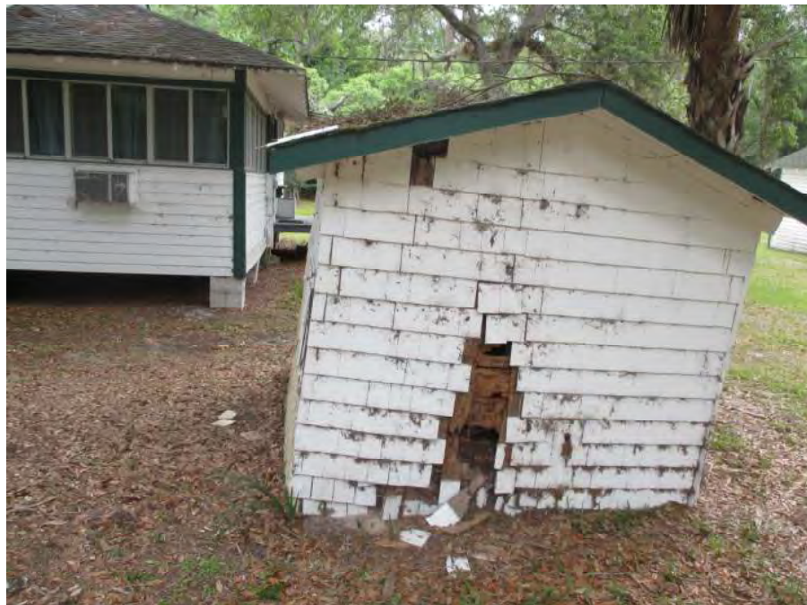
Photograph 6 Settled and Racked Structure
