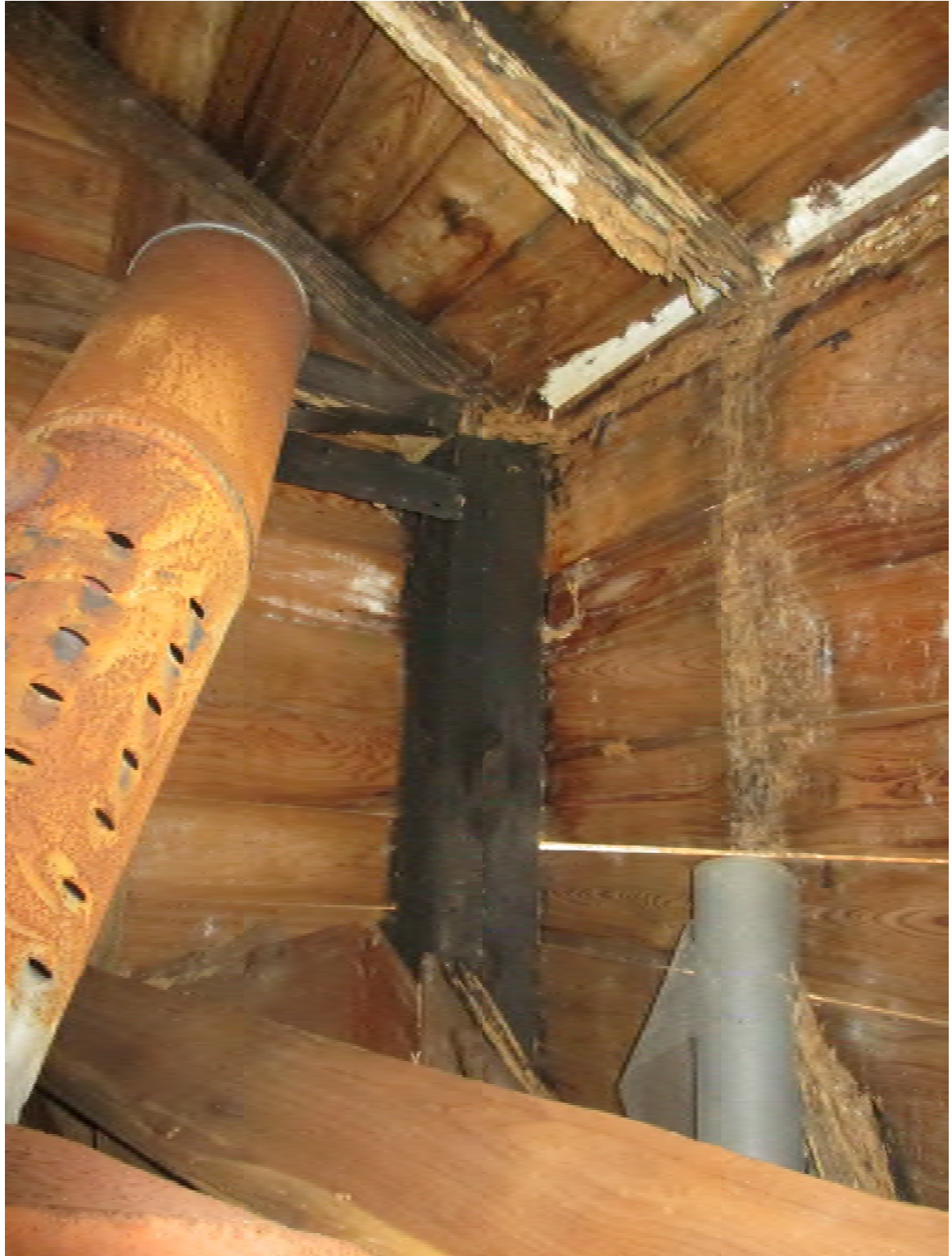
Photograph 8 Severely Deteriorated Wall and Roof Framing
