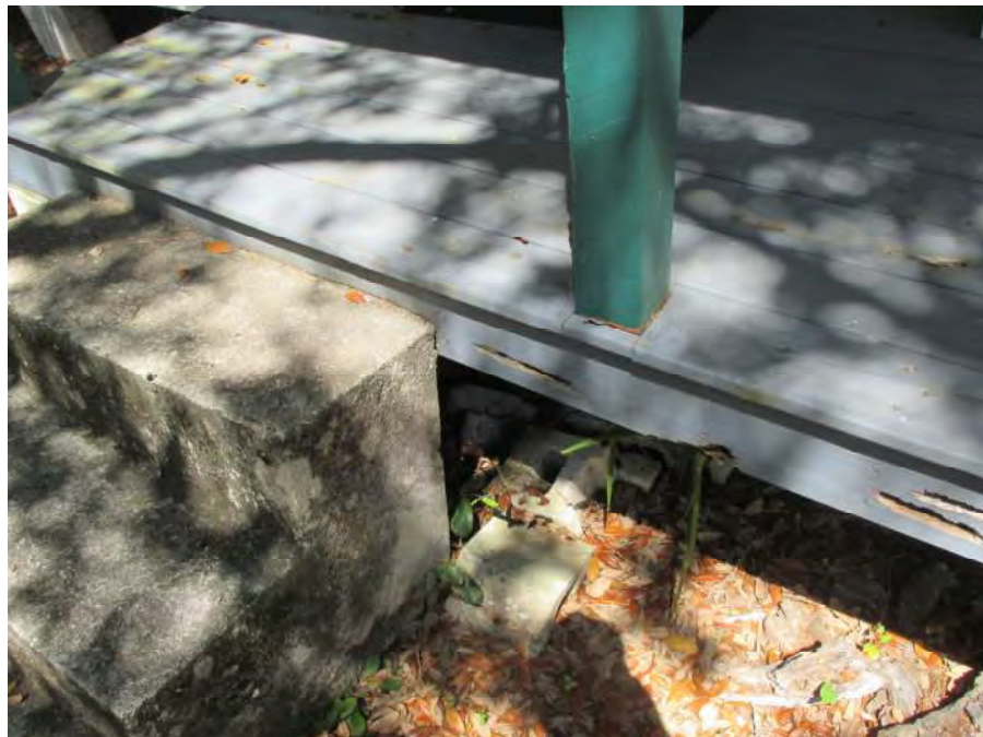
Photograph 19 Collapsed CMU Pier
