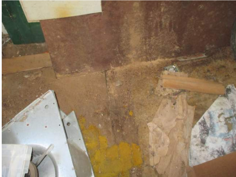
Photograph 8 Deteriorated Floor Decking at Rear Porch
