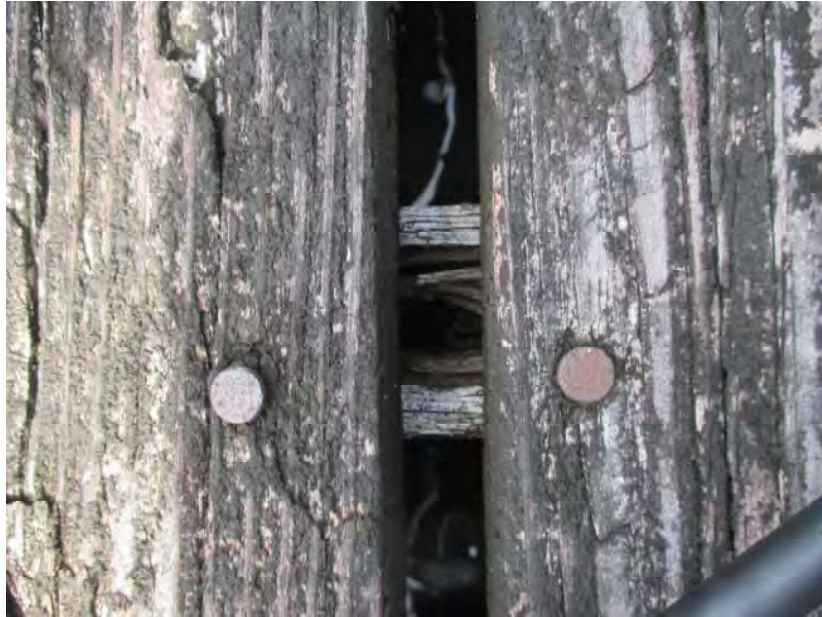
Photograph 3 Deteriorated 2x Stringer
