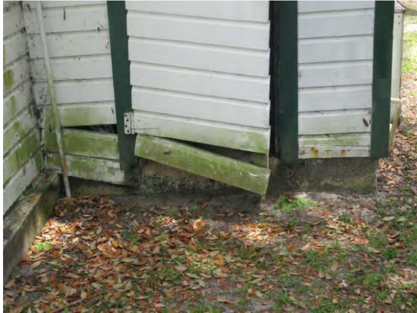
Photograph 10 Deteriorated Shed Siding
