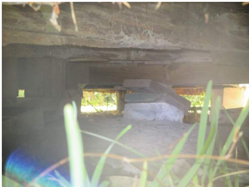
Photograph 11 Rotated and Loose Foundation
