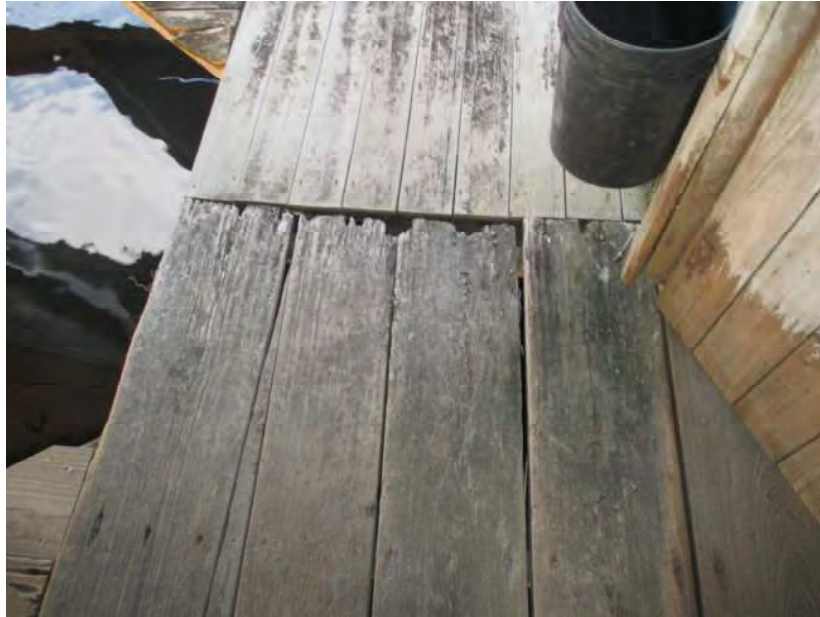
Photograph 9 Decking Deteriorated and Not Fastened
