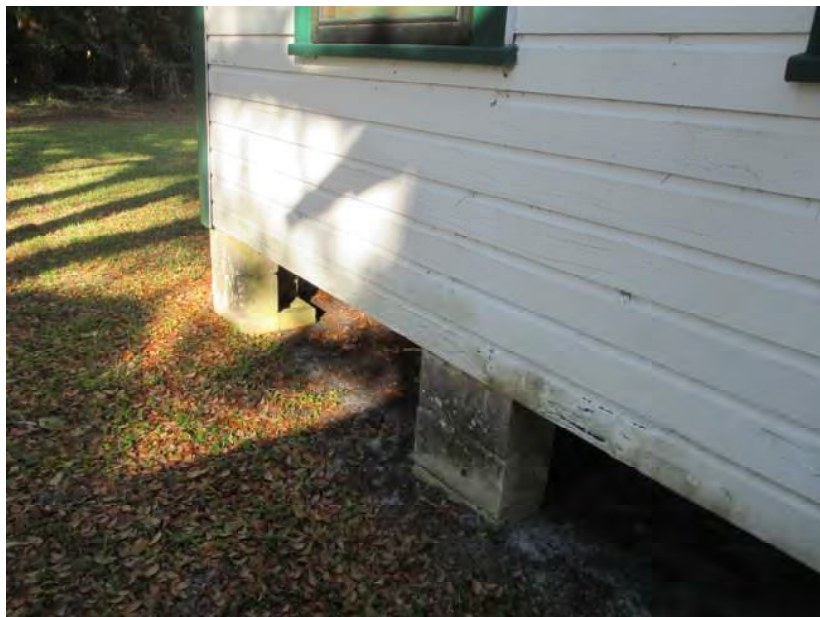
Photograph 9 Weathered Siding and Trim
