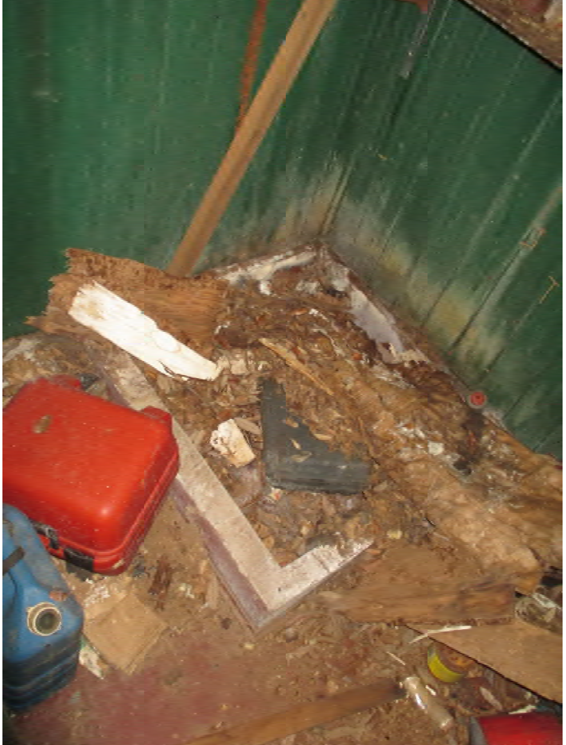
Photograph 7 Deteriorated Floor Decking at Addition
