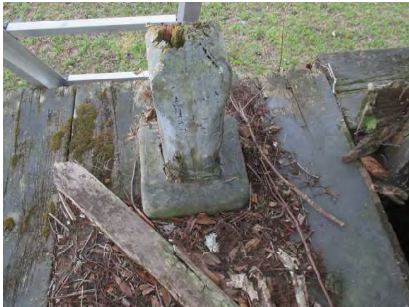
Photograph 9 Mooring Davit Deteriorated
