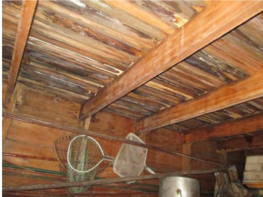
Photograph 7 Deteriorated Wall to Second-Floor Intersection
