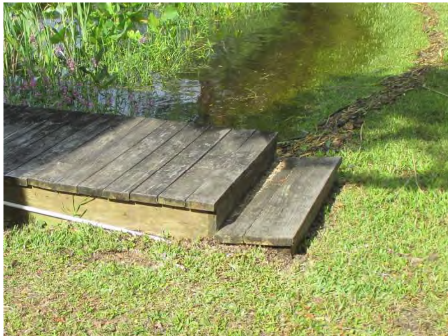
Photograph 14 Settled Entry Step
