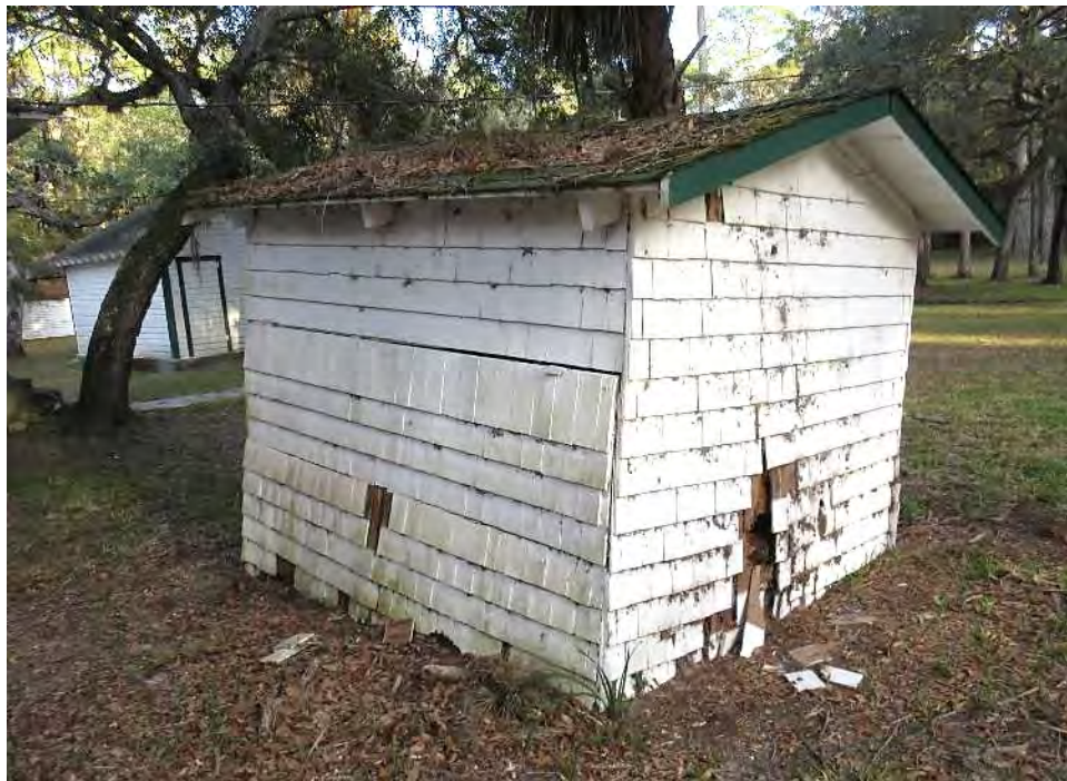
Detail view showing the access panel along the north façade, as well as the termite damage at the rear.
