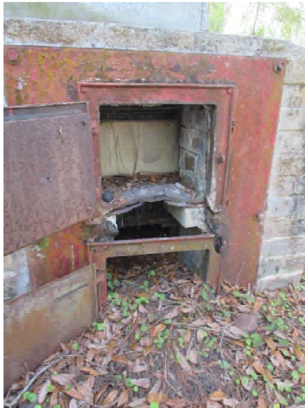
Photograph 5 Deteriorated Access Doors and Settled Corner
