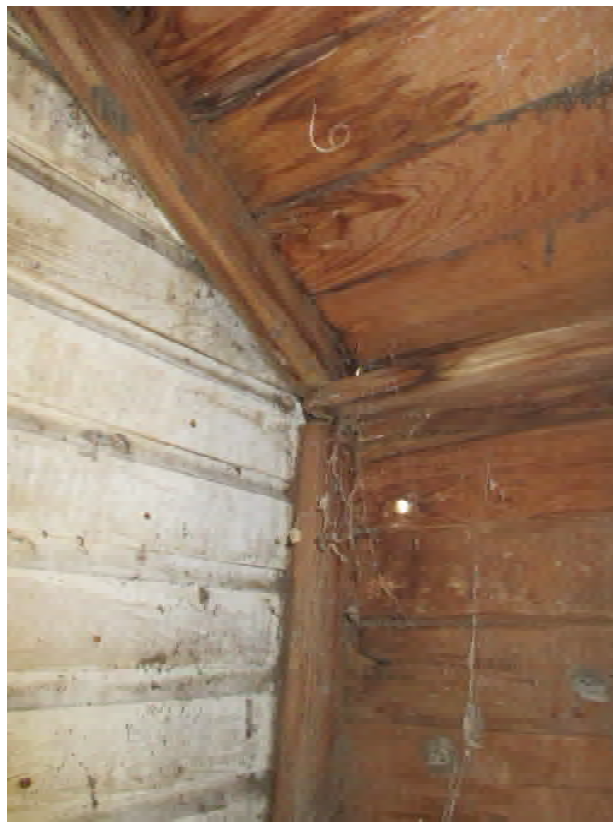
Photograph 9 Deteriorated Rear Shed Wall Framing
