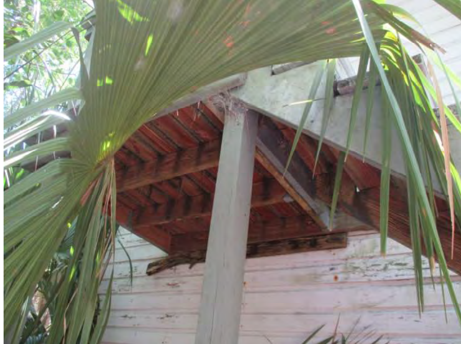
Photograph 13 Stair Ledger Severely Deteriorated
