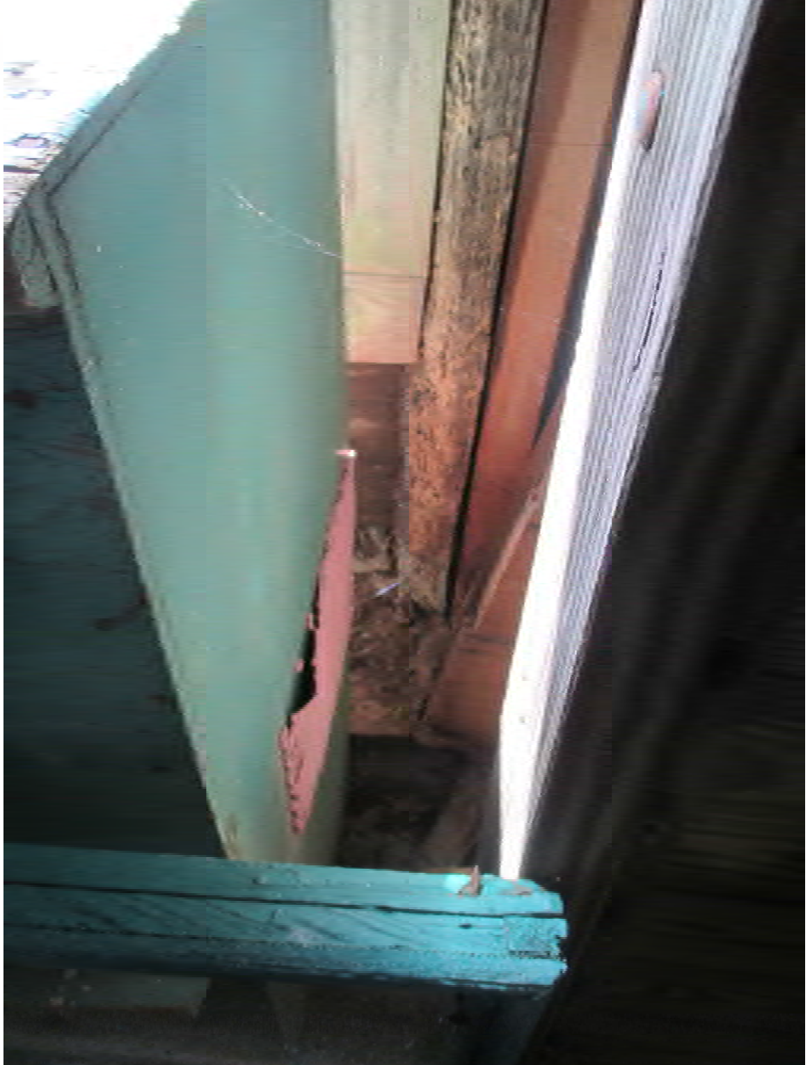
Photograph 7 Severely Deteriorated Wall Framing
