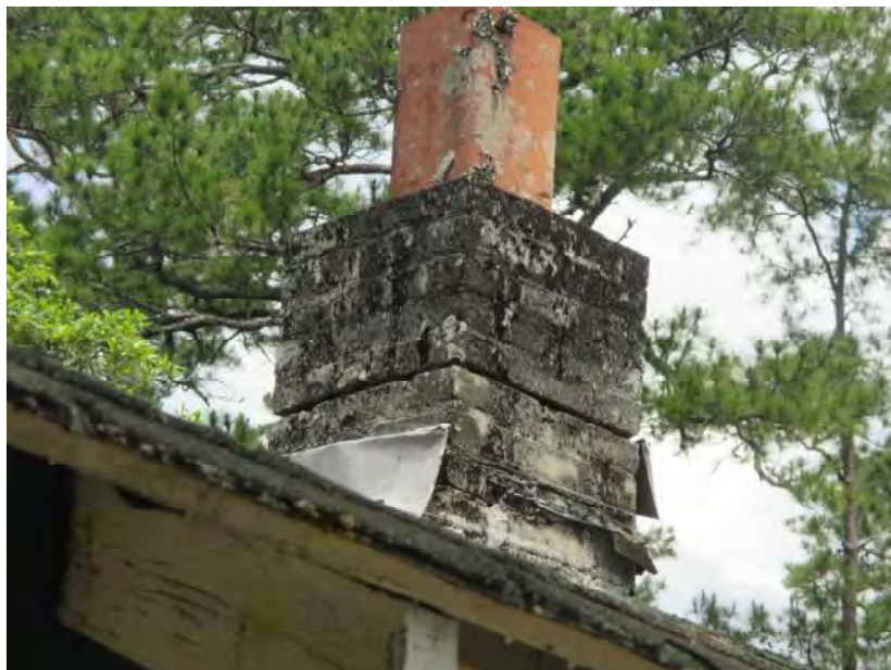
Photograph 4 Masonry Repointing Required at Chimney Cap
