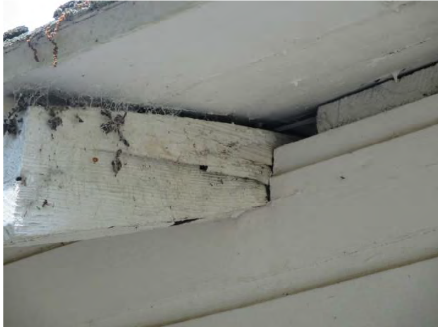
Photograph 13 Deteriorated Roof Joist
