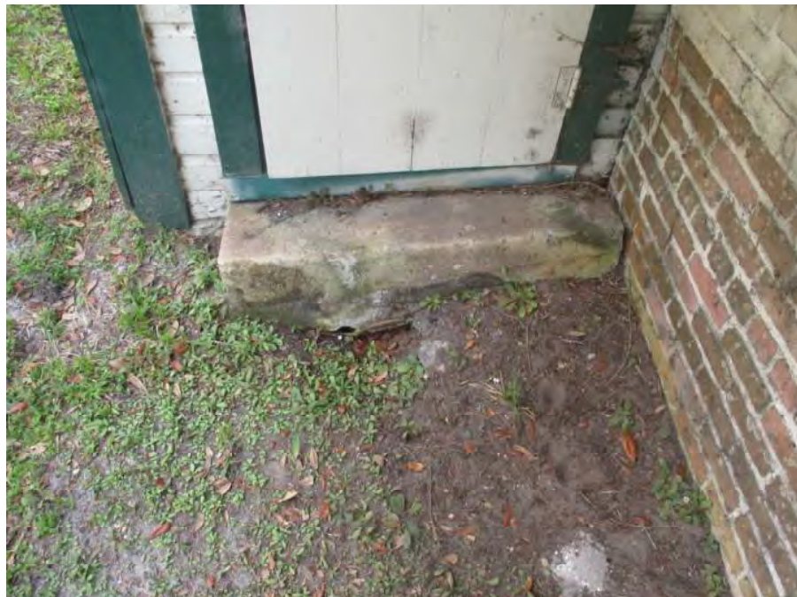
Photograph 16 Settled Entry Step
