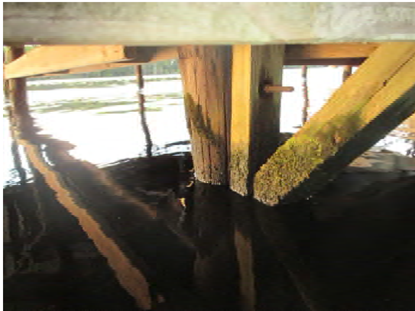
Photograph 10 Biological Growth at Waterline and Weather Checking
