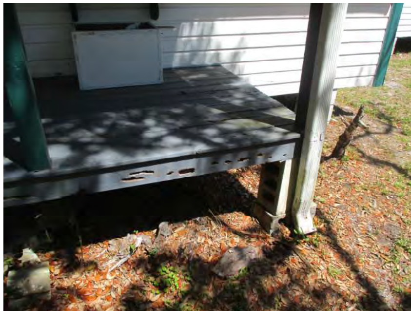
Photograph 7 Termite Damaged Rear Porch Entry Framing
