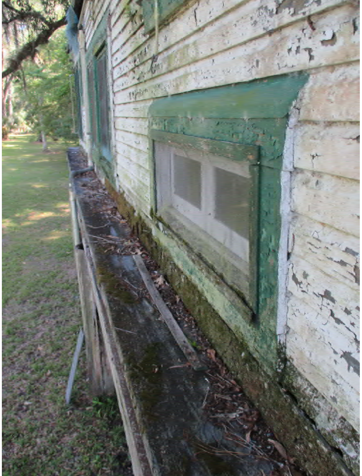
Photograph 10 Siding, Trim, Decking, and Wall Framing Severely Deteriorated
