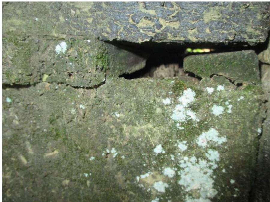
Photograph 16 Top of Houseboat Support Pile Deteriorated
