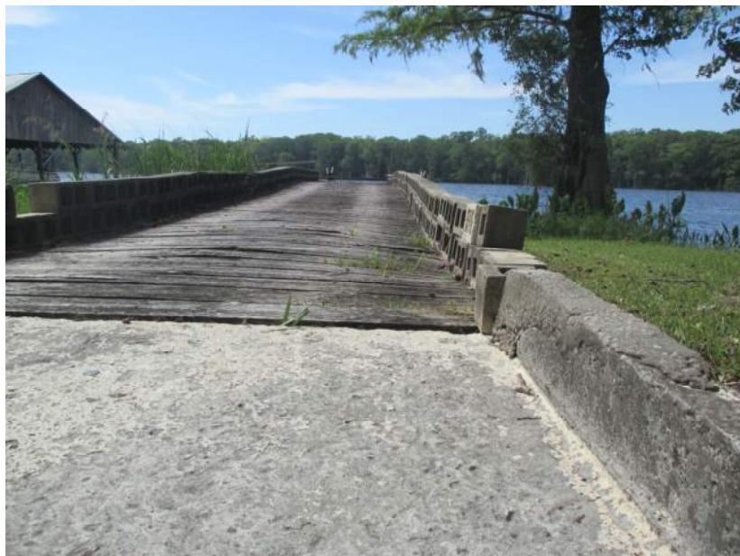
Photograph 6 Settlement of Dock Structure
