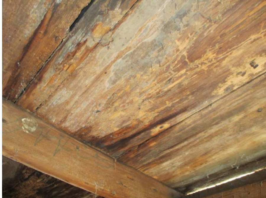
Photograph 5 Deteriorated Roof Sheathing
