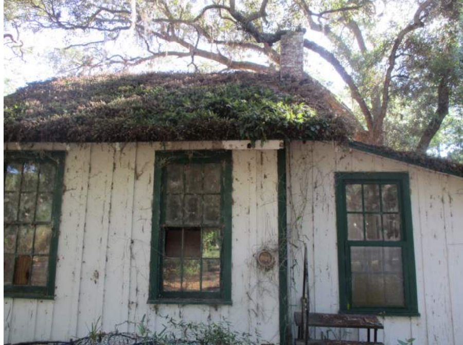
Photograph 2 Biological Growth on the Roof
