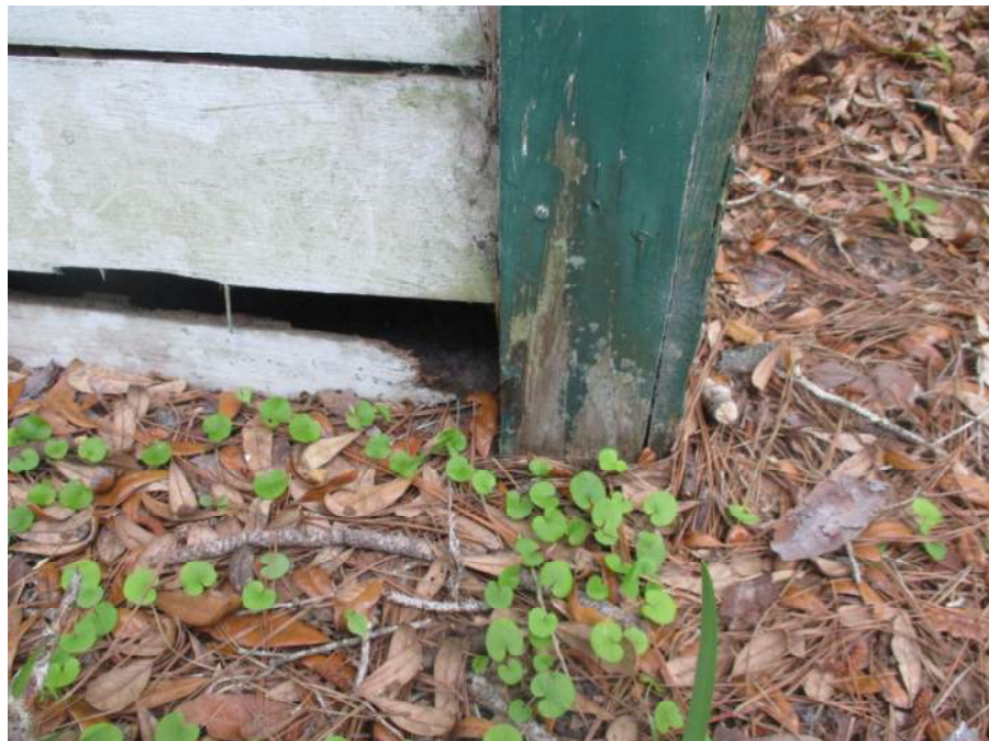
Photograph 4 Deteriorated Trim and Siding
