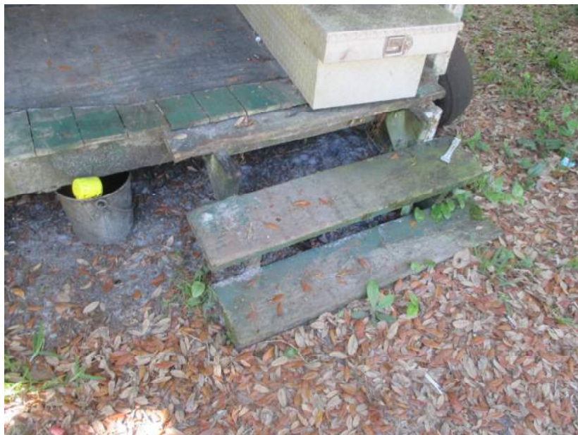
Photograph 15 Rotated and Deteriorated Main Entry Steps
