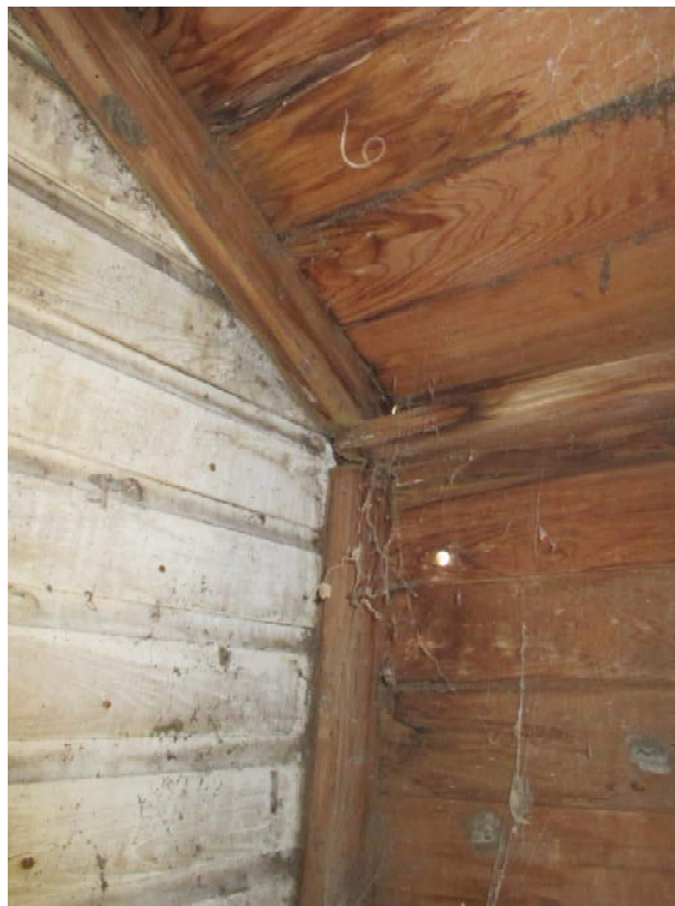
Photograph 9 Deteriorated Rear Shed Wall Framing
