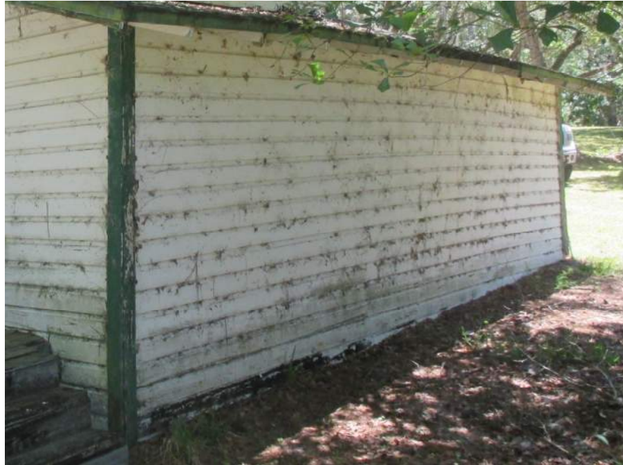
Photograph 11 Perimeter Vegetation Buildup
