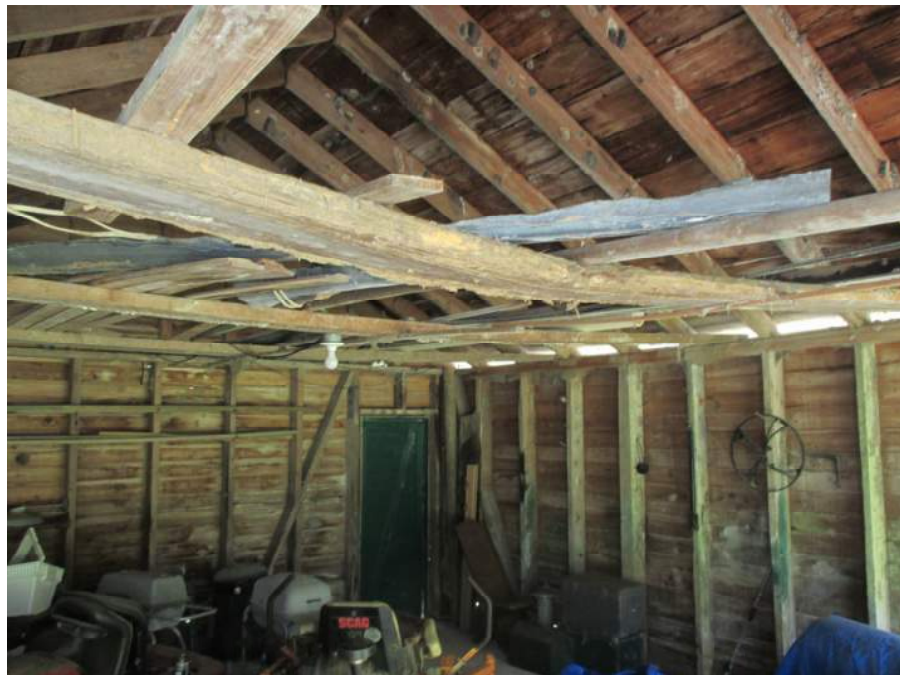
Photograph 3 Termite Damaged Framing
