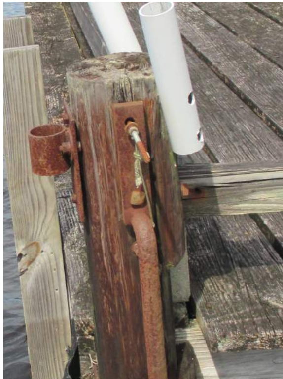
Photograph 10 Corroded and Missing Hardware
