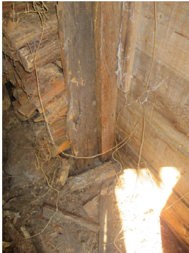
Photograph 4 Deteriorated Wall Framing and Sheathing
