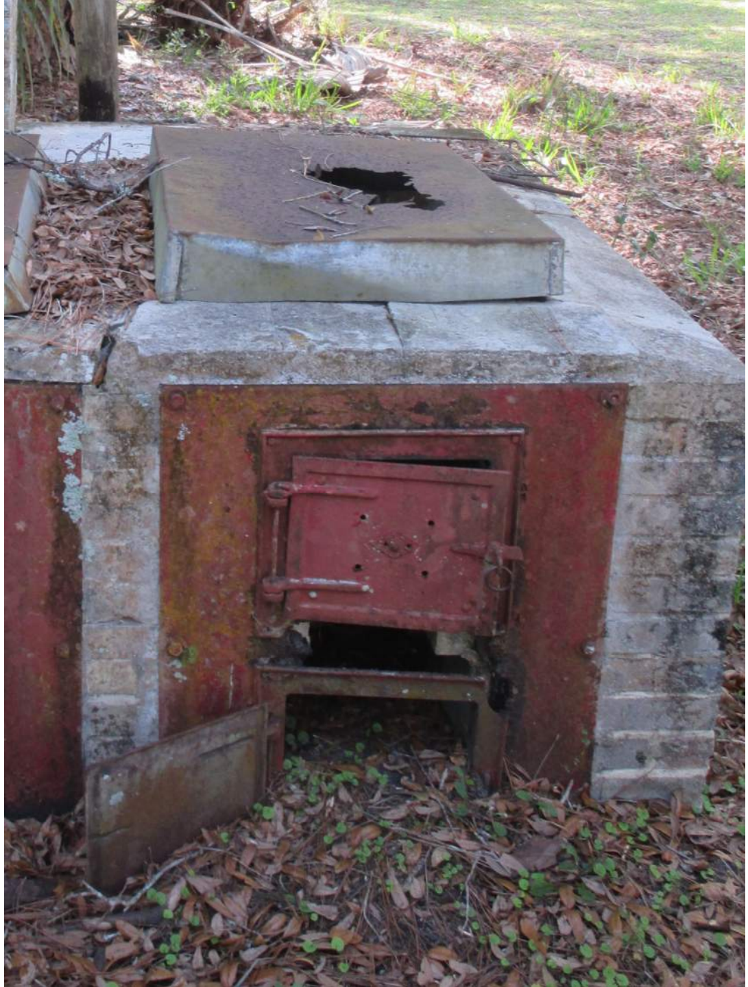
Photograph 6 Deteriorated Access Doors and Settled Corner
