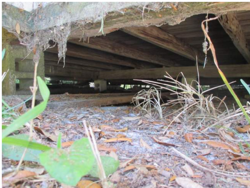
Photograph 5 Moisture or Termite Floor Framing Deteriorated
