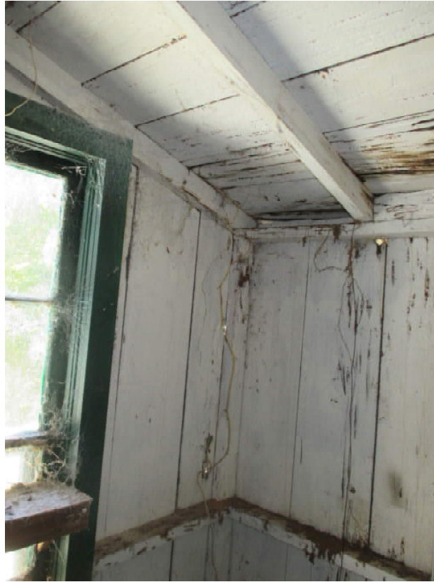
Photograph 4 Moisture Damaged Framing
