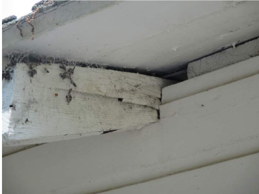
Photograph 13 Deteriorated Roof Joist
