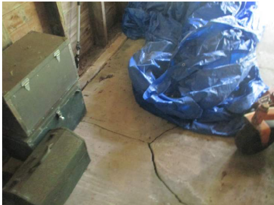
Photograph 7 Vertical and Horizontal Slab Displacement
