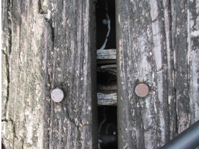
Photograph 3 Deteriorated 2x Stringer
