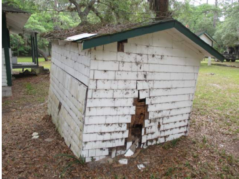
Photograph 3 Severely Deteriorated Wall Sheathing and Siding
