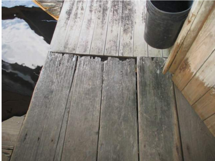
Photograph 9 Decking Deteriorated and Not Fastened
