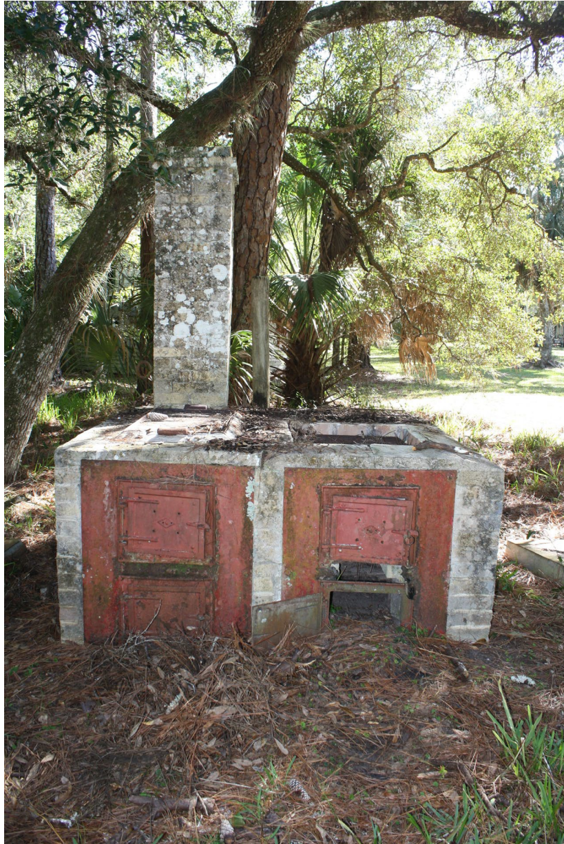
North side elevation of the grill. Note that some components will need restoration, including the concrete top.
