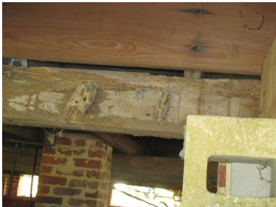
Photograph 11 Weathered Floor Framing
