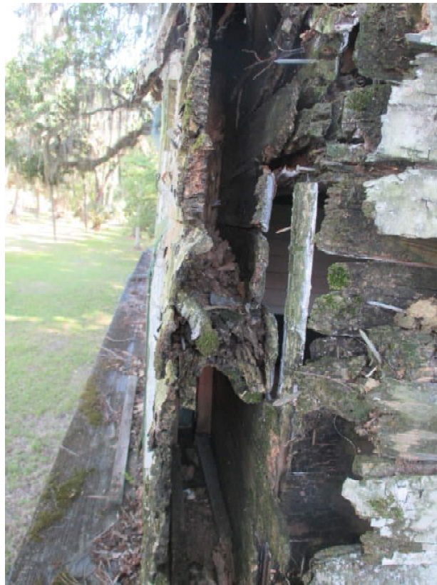
Photograph 5 Wall Studs, Siding, Blocking, and Decking Severely Deteriorated
