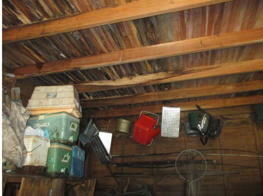
Photograph 5 Deteriorated Floor Framing and Decking
