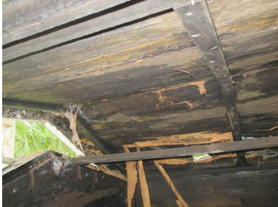
Photograph 3 Deteriorated Roof Sheathing and Framing
