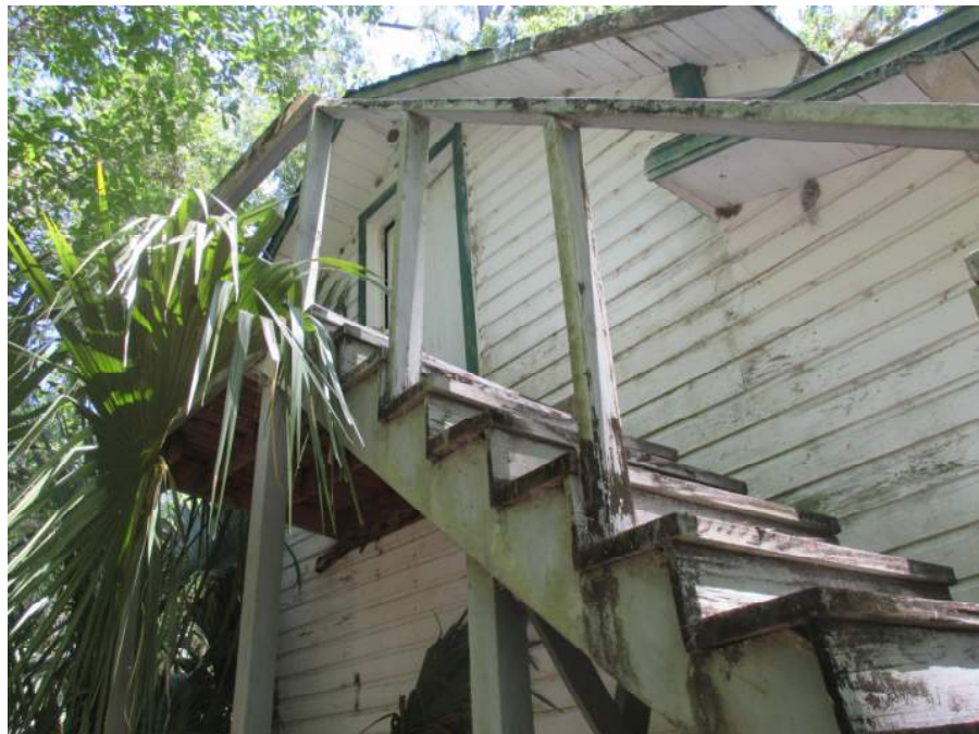
Photograph 16 Severely Deteriorated Attic Access Stair
