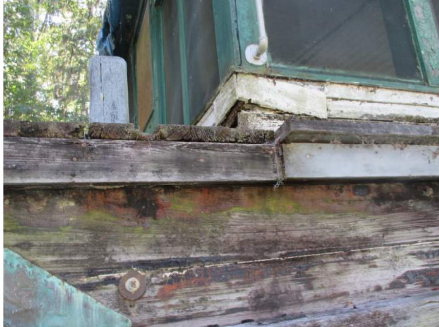
Photograph 11 Decking and Trim Deteriorated with Corroded Fasteners
