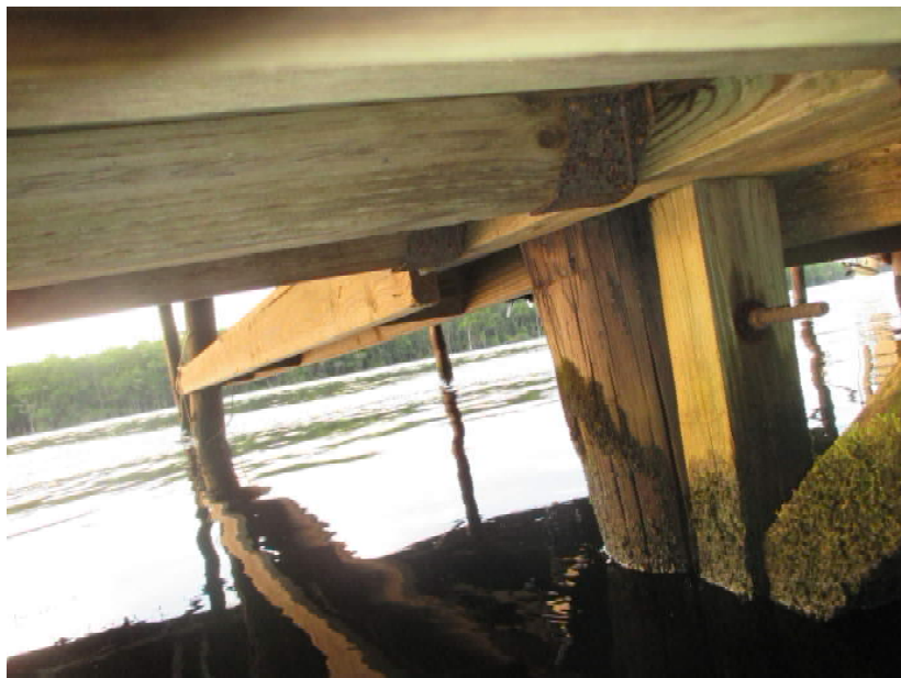
Photograph 8 Joist Hangers Deteriorated
