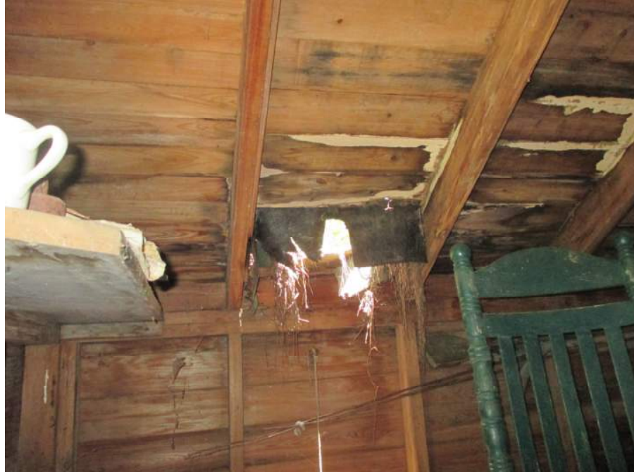
Photograph 3 Deteriorated Roof Framing and Sheathing
