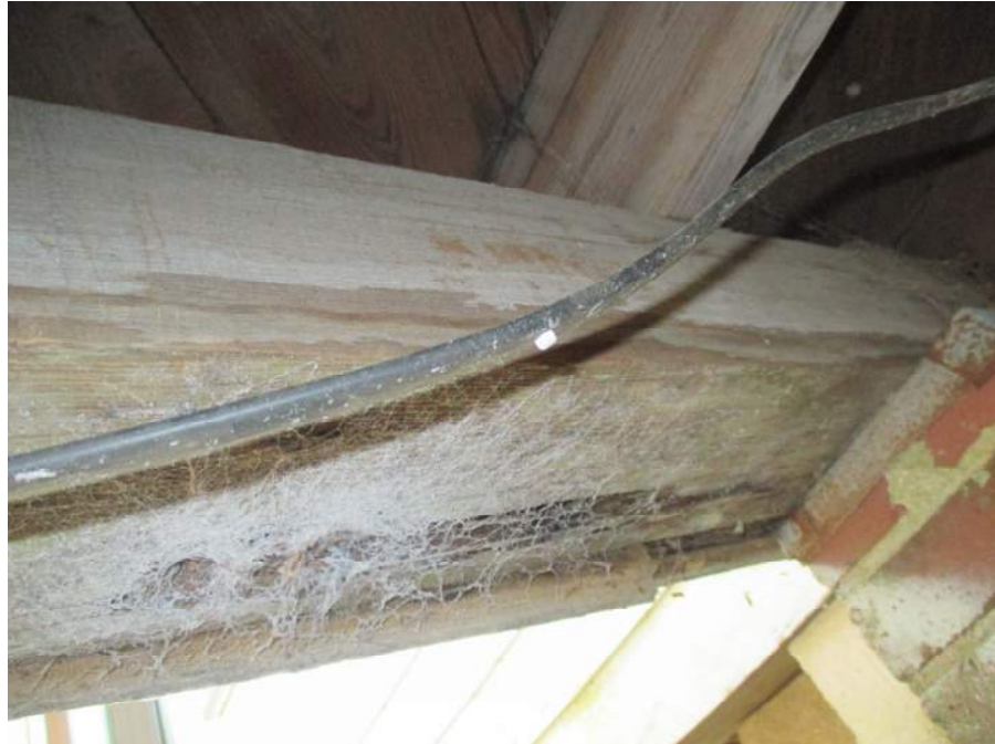
Photograph 10 Termite Damaged Floor Framing
