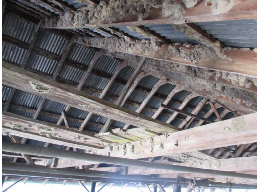
Photograph 5 Roof Rafters Covered in Mud Dauber Nests
