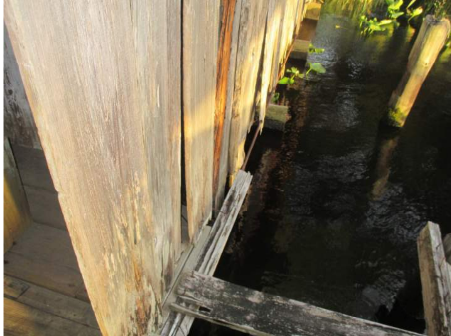
Photograph 13 Deterioration at Base of Siding and Missing Deteriorated Framing
