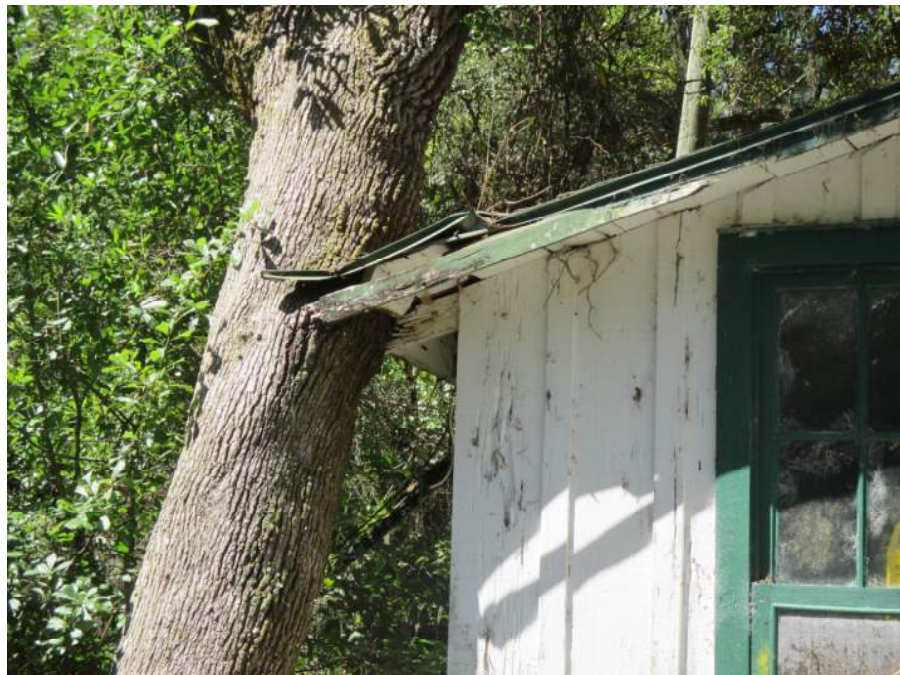
Photograph 3 Damaged Rear Corner Due to Tree
