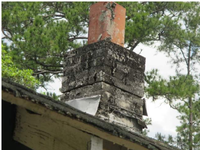
Photograph 4 Masonry Repointing Required at Chimney Cap
