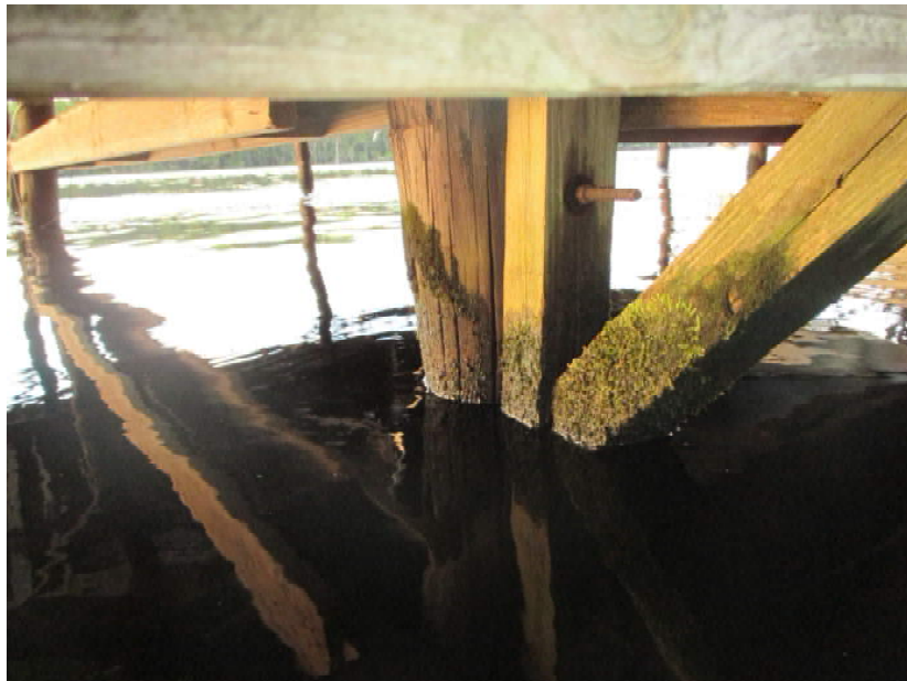
Photograph 10 Biological Growth at Waterline and Weather Checking
