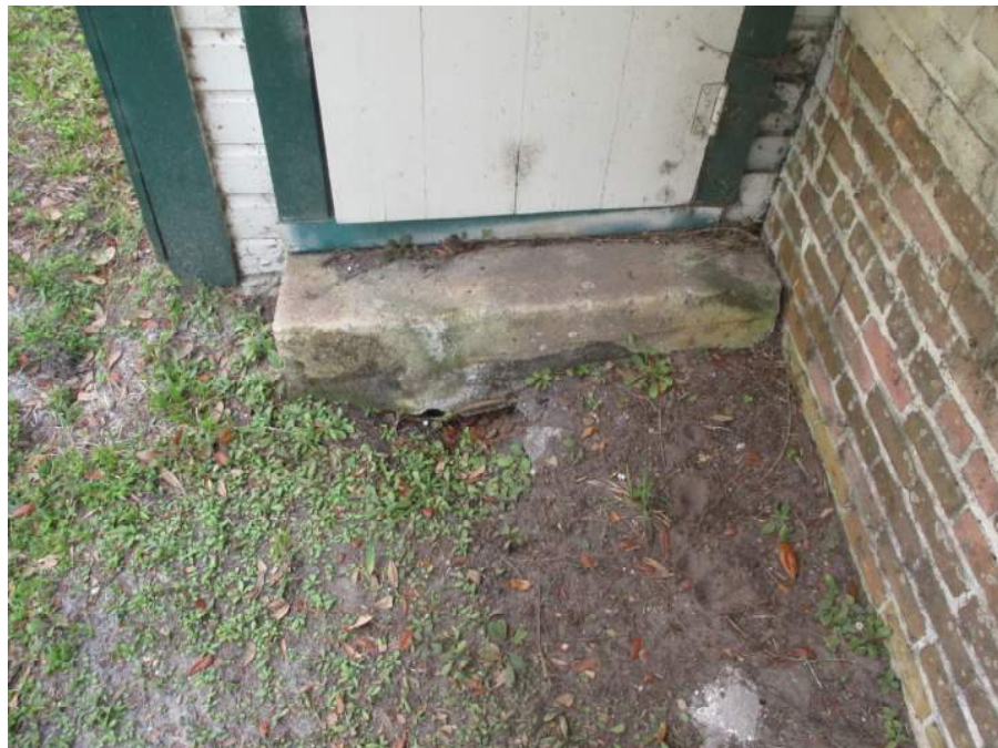
Photograph 16 Settled Entry Step
