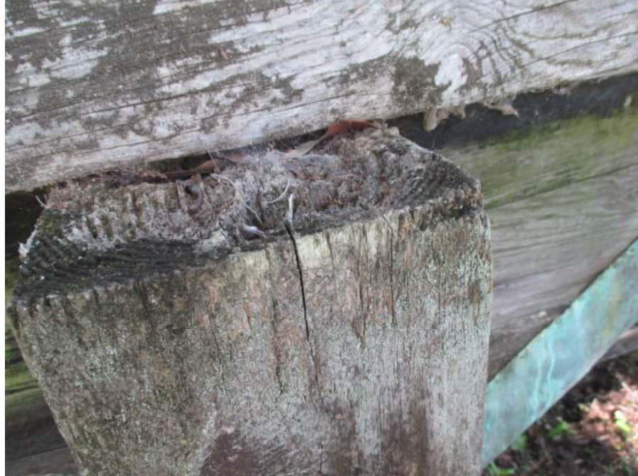
Photograph 15 Top of Houseboat Support Pile Deteriorated
