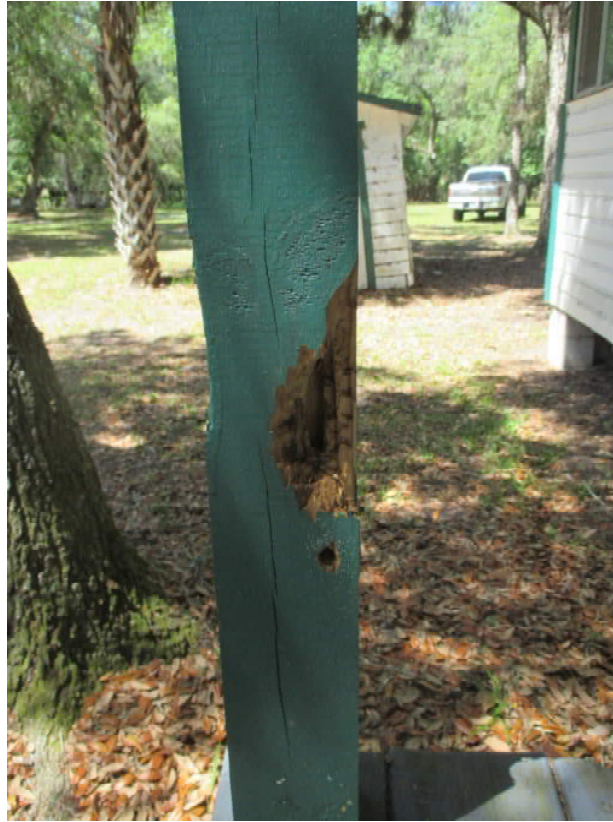
Photograph 8 Termite Damaged Porch Column
