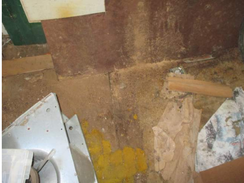
Photograph 8 Deteriorated Floor Decking at Rear Porch
