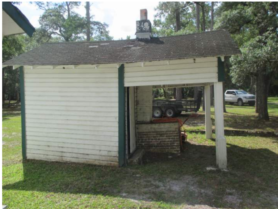
Photograph 2 Settled and Hinging Structural Framing
