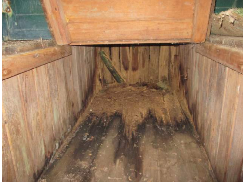
Photograph 8 Kitchen Floor Storage Well Moisture Damage
