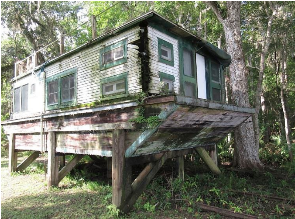
East and north sides of the Houseboat. Note wood rot damage at the northeast corner.
