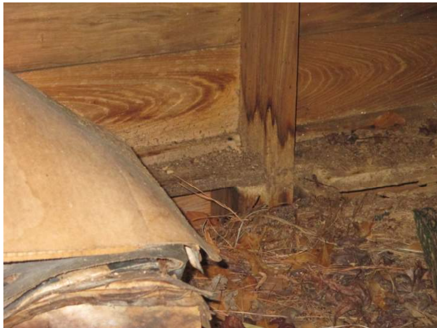
Photograph 6 Deteriorated Wall to Second-Floor Intersection
