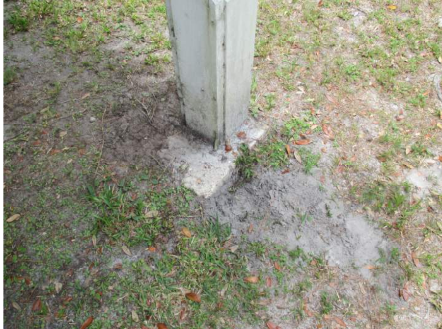
Photograph 15 Settled Column Foundation
