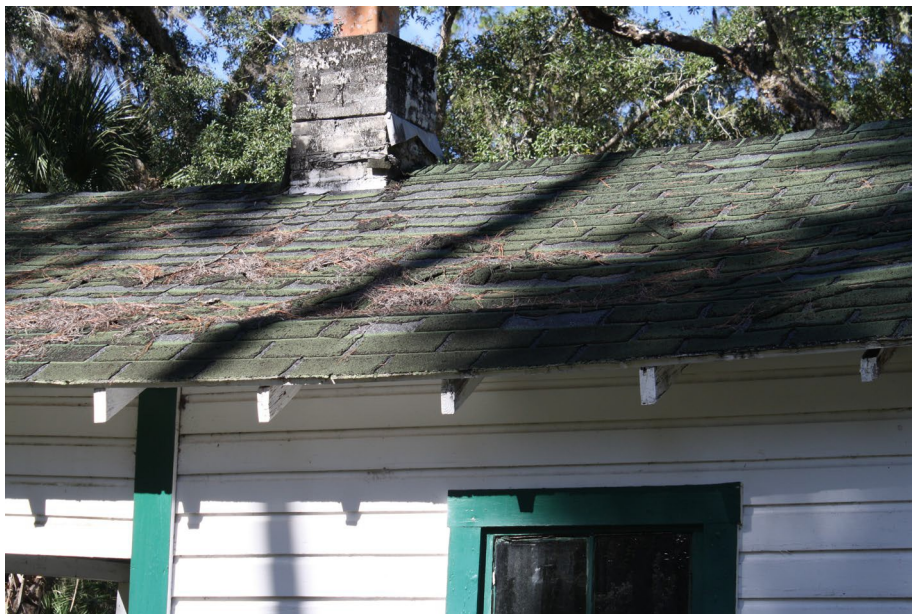
Fryer Shed chimney. Deteriorated and needs restoration.
