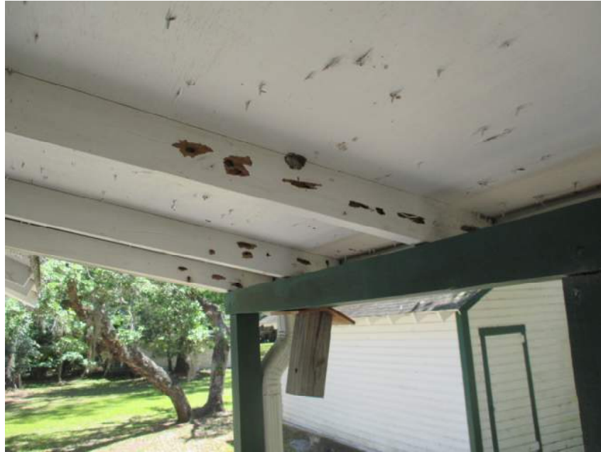
Photograph 6 Termite Damaged Rafter Tail at Rear Porch
