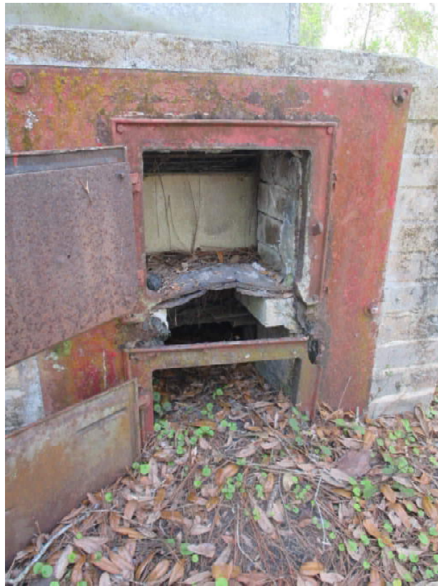
Photograph 5 Deteriorated Access Doors and Settled Corner
