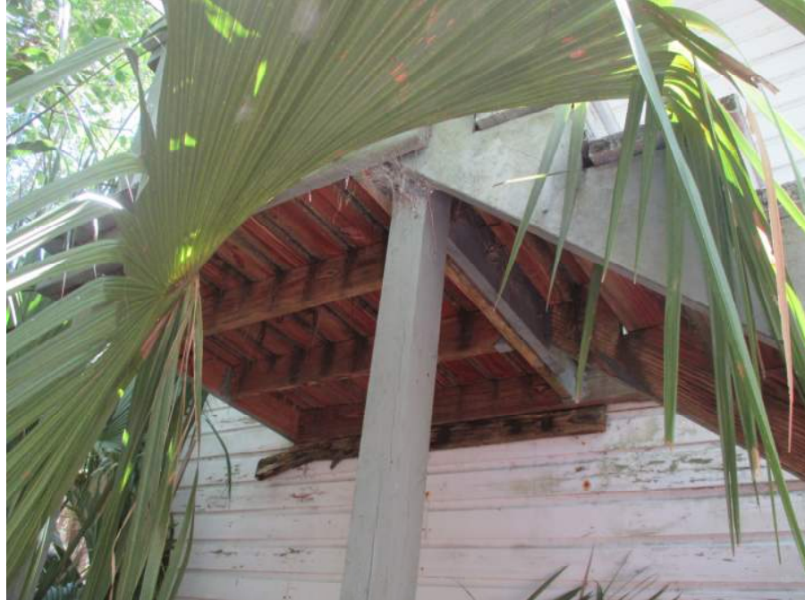
Photograph 13 Stair Ledger Severely Deteriorated
