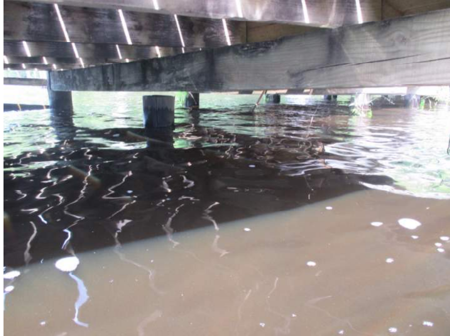
Photograph 7 Timber Pile Settled and Not in Contact with Framing
