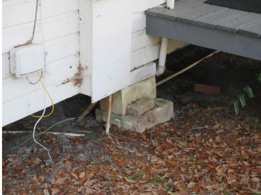
Photograph 18 Dry-Stacked and Unstable CMU Pier
