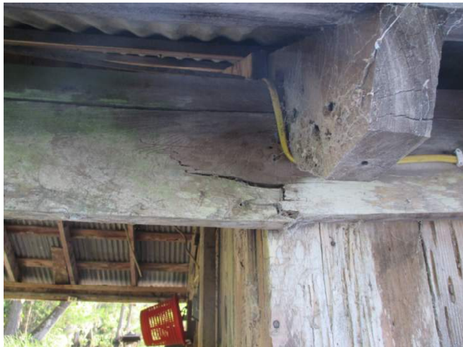
Photograph 6 Cracked Perimeter Beam
