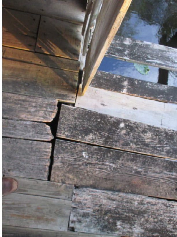
Photograph 7 Decking Deteriorated and Not Fastened
