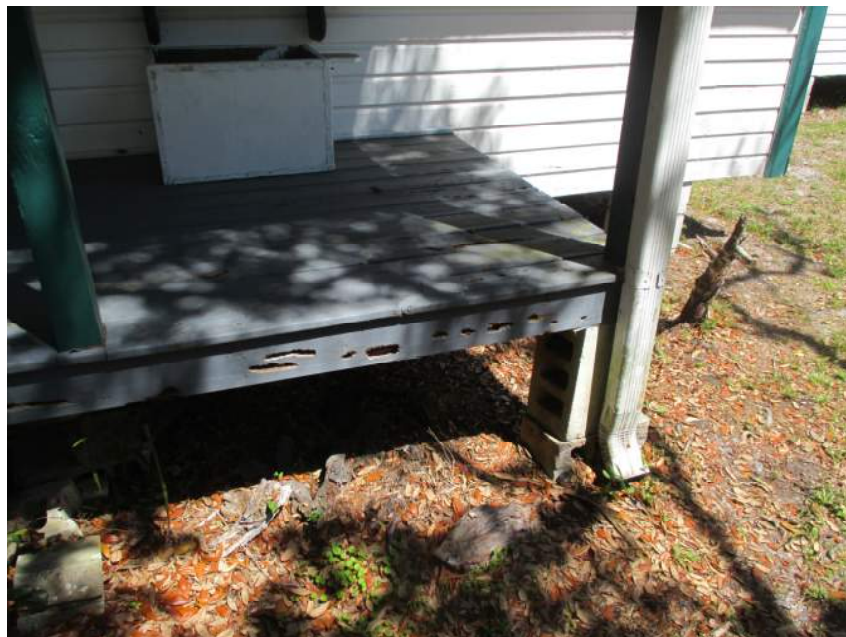
Photograph 7 Termite Damaged Rear Porch Entry Framing
