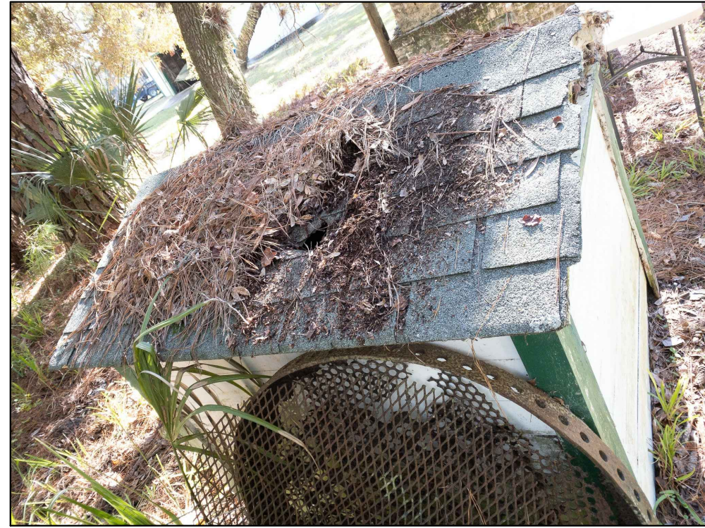
2 SMOKER ROOF DAMAGE (OYSTER GRILL IN FOREGROUND) SCALE: N. T. S.
