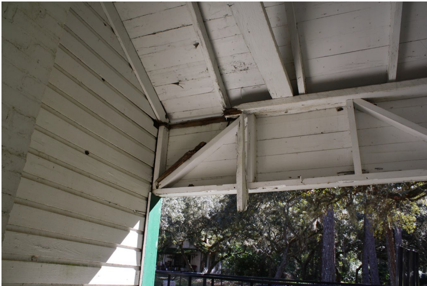
Fryer Shed plate deterioration.
