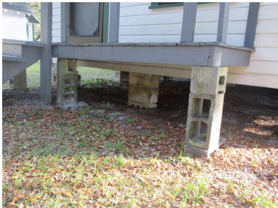
Photograph 17 Dry-Stacked and Unstable CMU Piers
