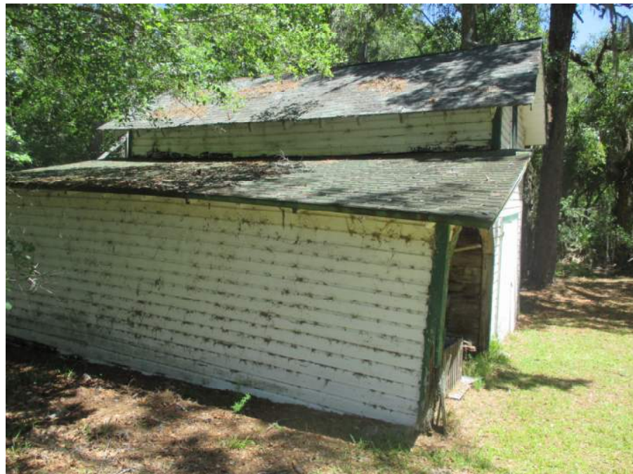
Photograph 12 Corner Racked and Settled
