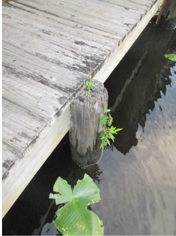
Photograph 11 Deterioration at Top of Timber Pile
