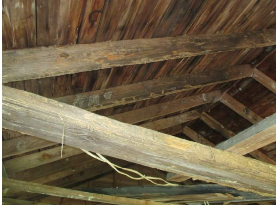
Photograph 2 Deteriorated Roof Rafters
