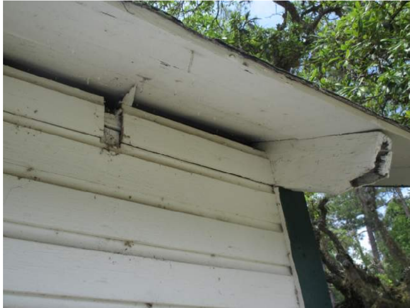
Photograph 4 Deteriorated Rafter Tails
