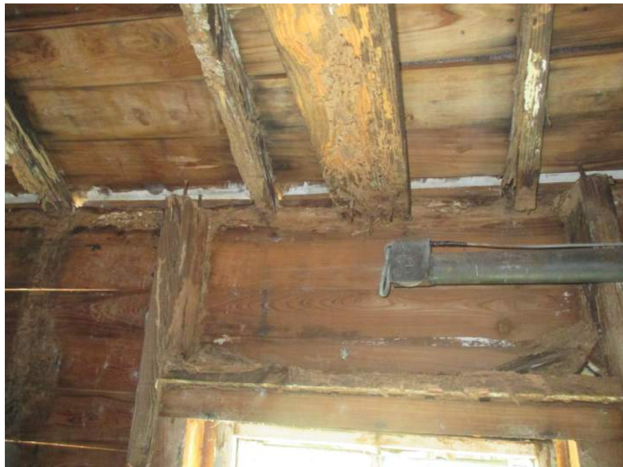
Photograph 6 Severely Deteriorated Wall and Roof Framing
