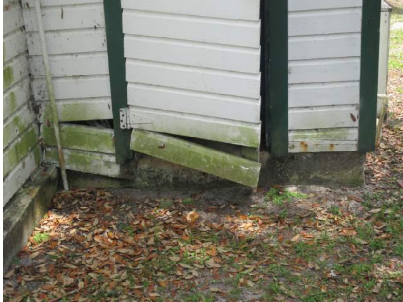
Photograph 10 Deteriorated Shed Siding
