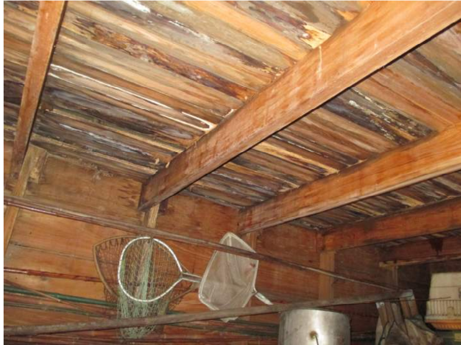
Photograph 7 Deteriorated Wall to Second-Floor Intersection
