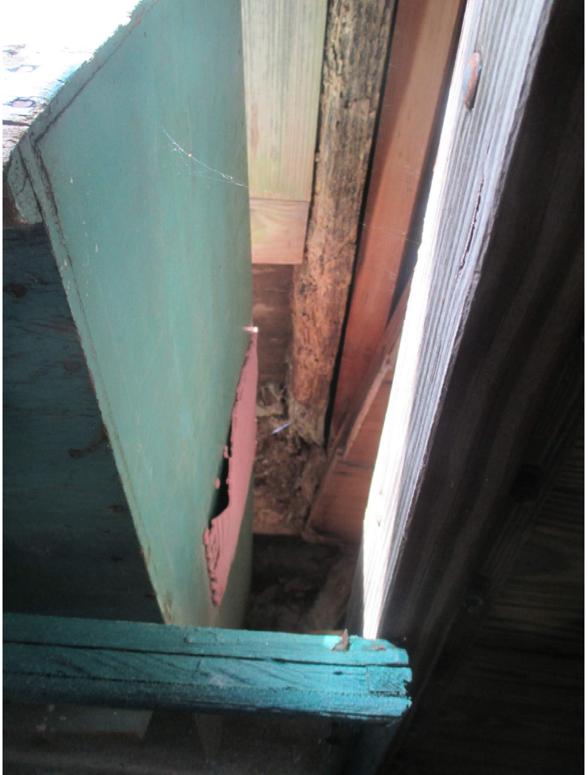
Photograph 7 Severely Deteriorated Wall Framing
