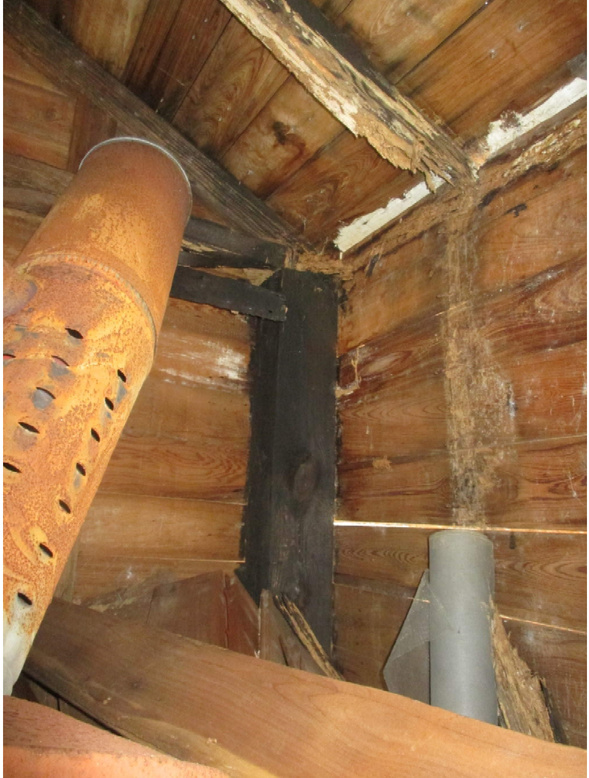
Photograph 8 Severely Deteriorated Wall and Roof Framing
