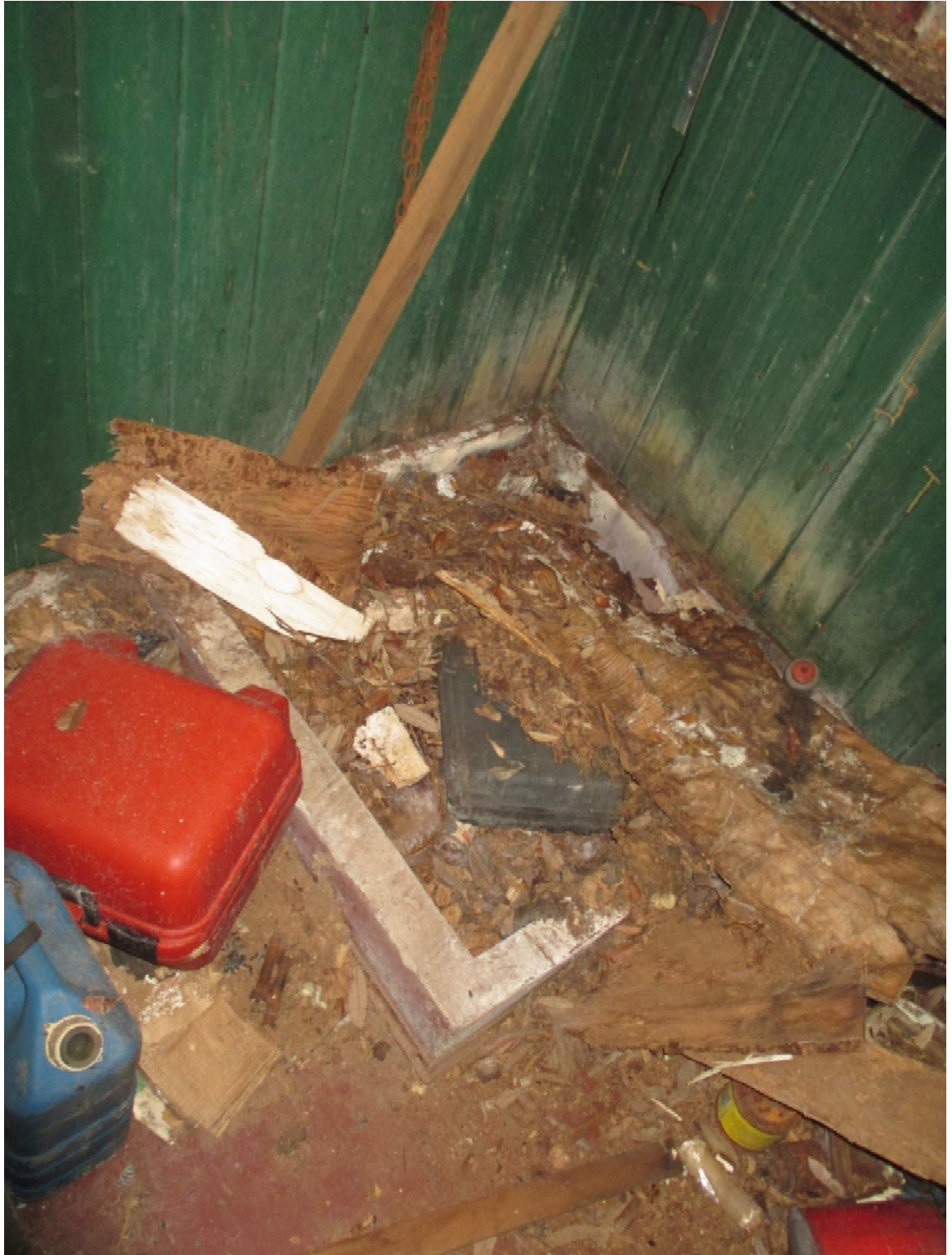
Photograph 7 Deteriorated Floor Decking at Addition
