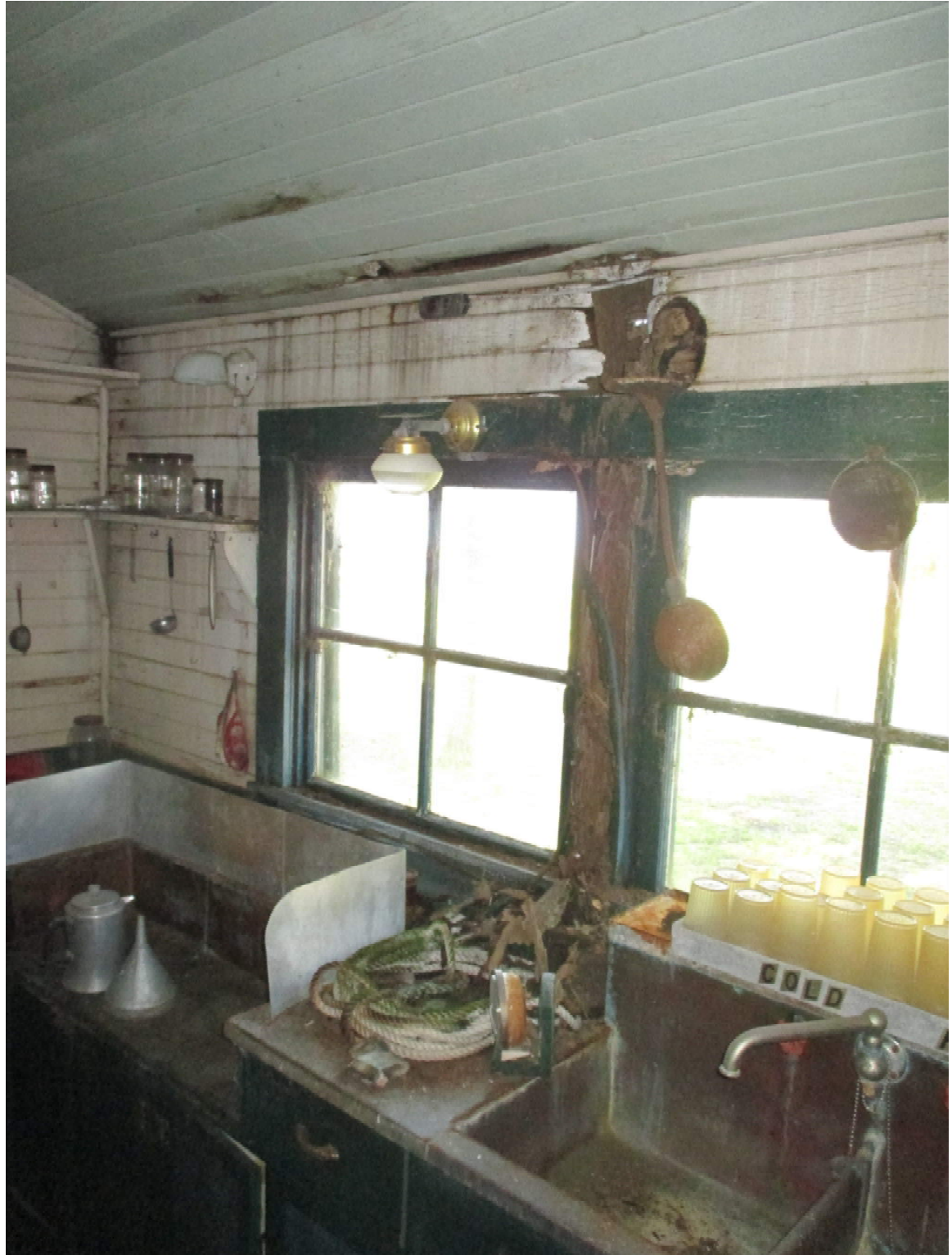
Photograph 7 Wall Framing and Siding Severely Deteriorated
