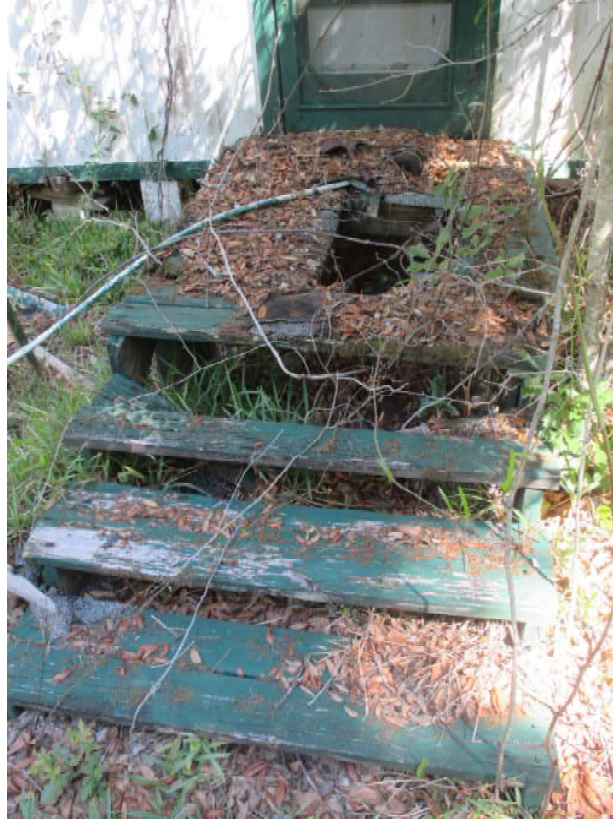
Photograph 14 Failed Rear Porch Entry Steps
