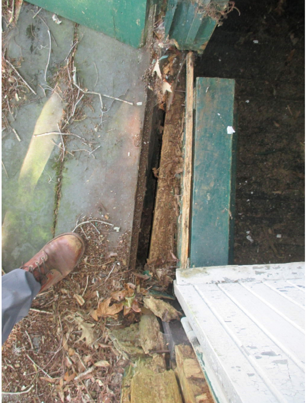
Photograph 6 Decking, Entry Step, and Wall Framing Severely Deteriorated
