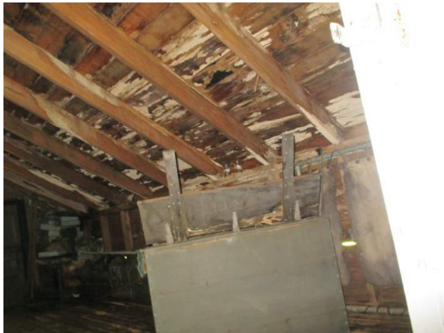
Photograph 4 Deteriorated Roof Sheathing and Framing
