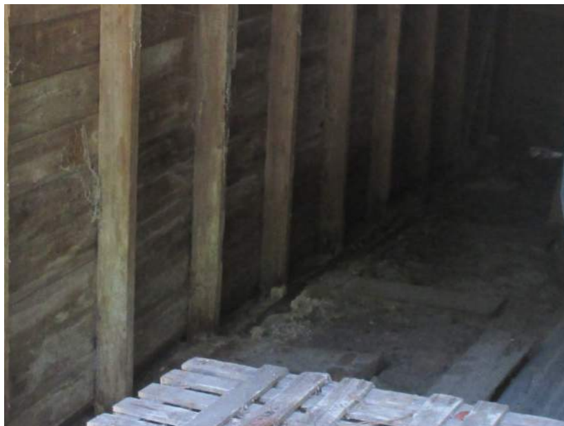
Photograph 10 Base of Wall Studs Deteriorated
