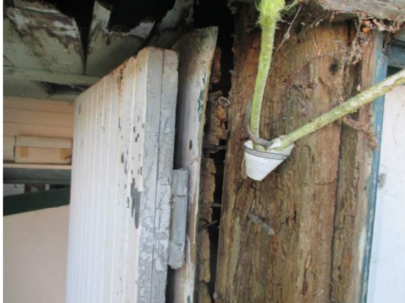
Photograph 4 North Wall and Roof Joists Severely Deteriorated
