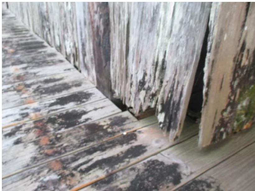
Photograph 12 Deterioration at Base of Siding
