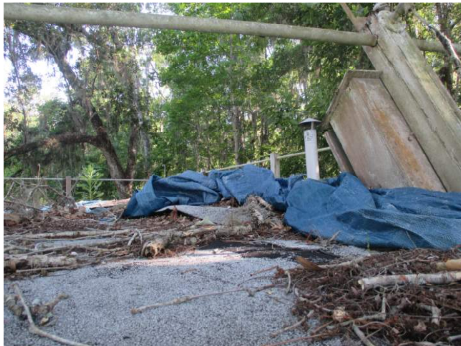
Photograph 2 Roof Tarp and Debris on Roof
