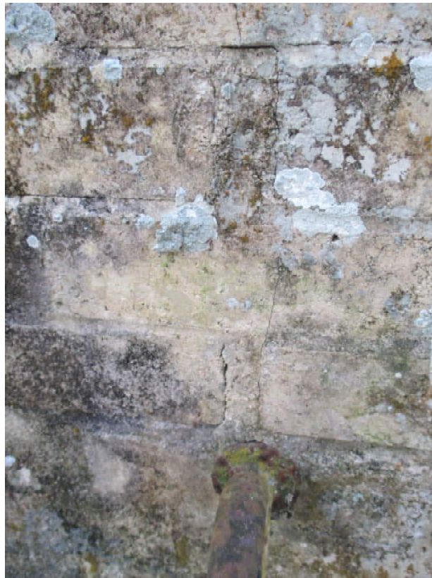
Photograph 3 Vertical Crack in Clay Brick
