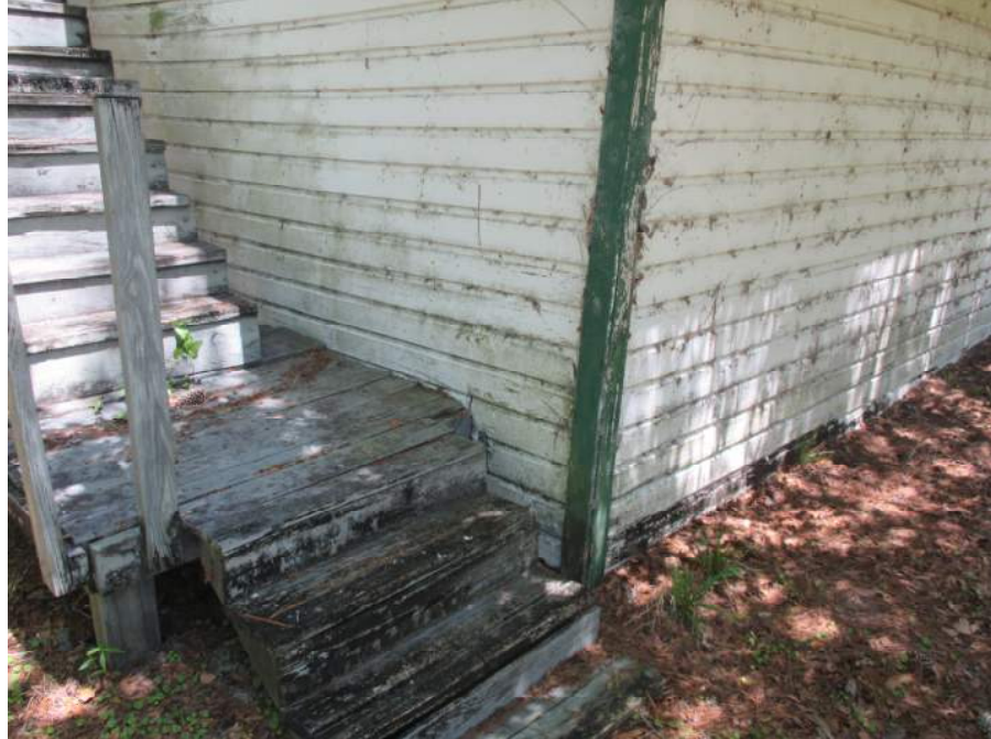
Photograph 15 Severely Deteriorated Attic Access Stair
