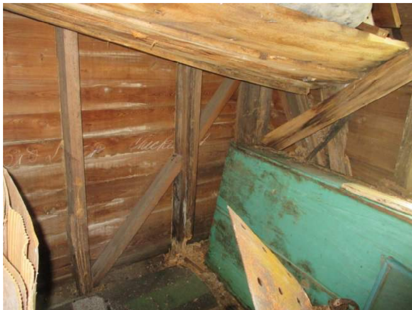
Photograph 10 Failed Storage Shelf
