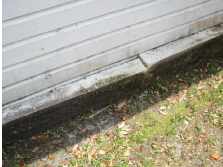
Photograph 6 Vertical and Horizontal Foundation Displacement
