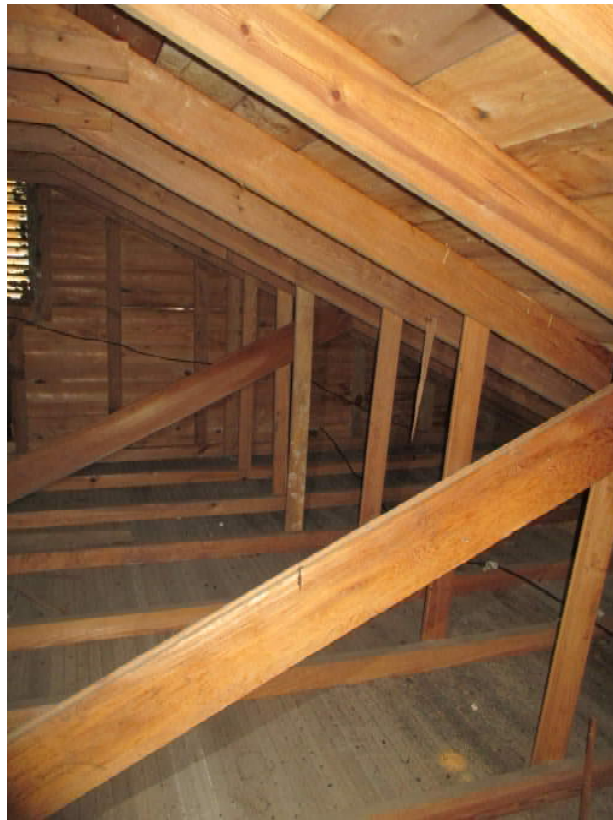
Photograph 5 Missing Diagonals within Attic
