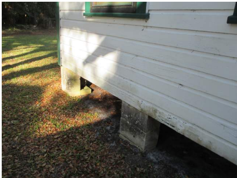
Photograph 9 Weathered Siding and Trim
