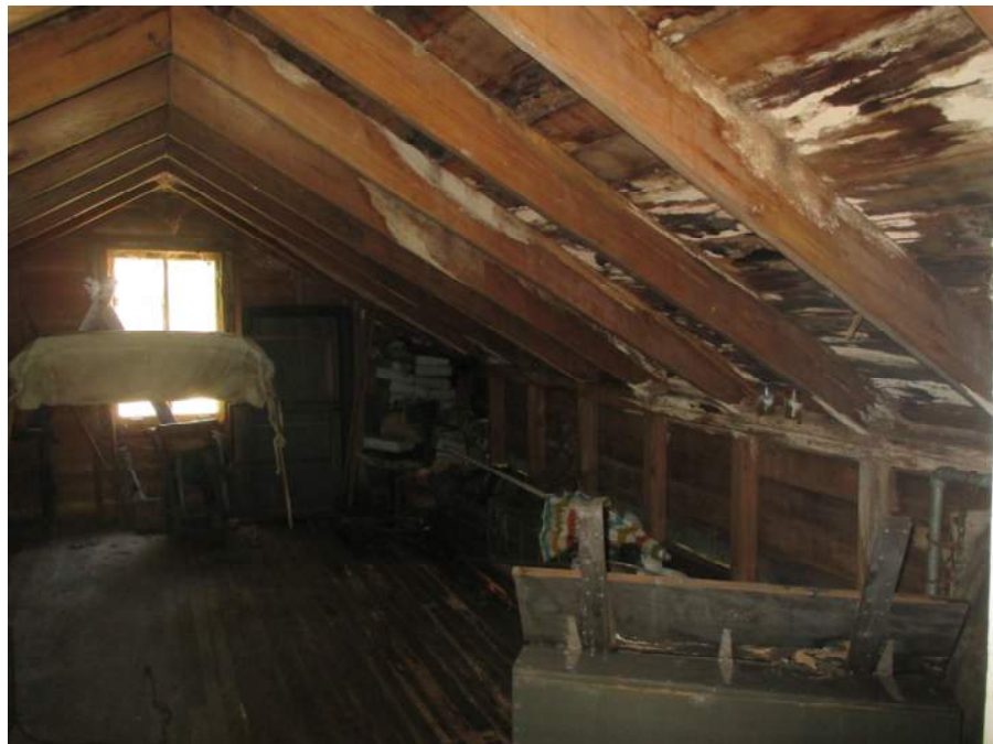
Photograph 2 Deteriorated Roof and Wall Framing
