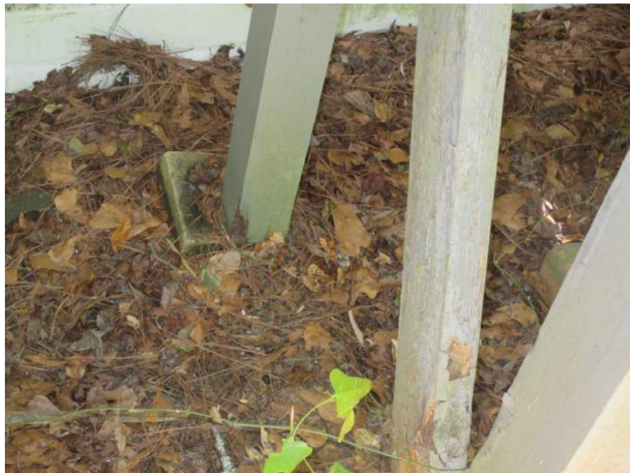
Photograph 14 Stair Column Not on Stable Foundation
