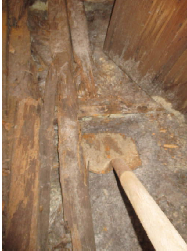
Photograph 9 Deteriorated Floor Decking and Framing Bearing on Grade
