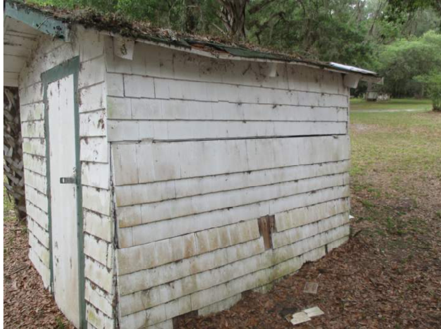
Photograph 1 Vertically Hinged Woodshed Access Door
