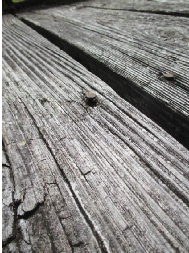
Photograph 5 Raised Nail Heads
