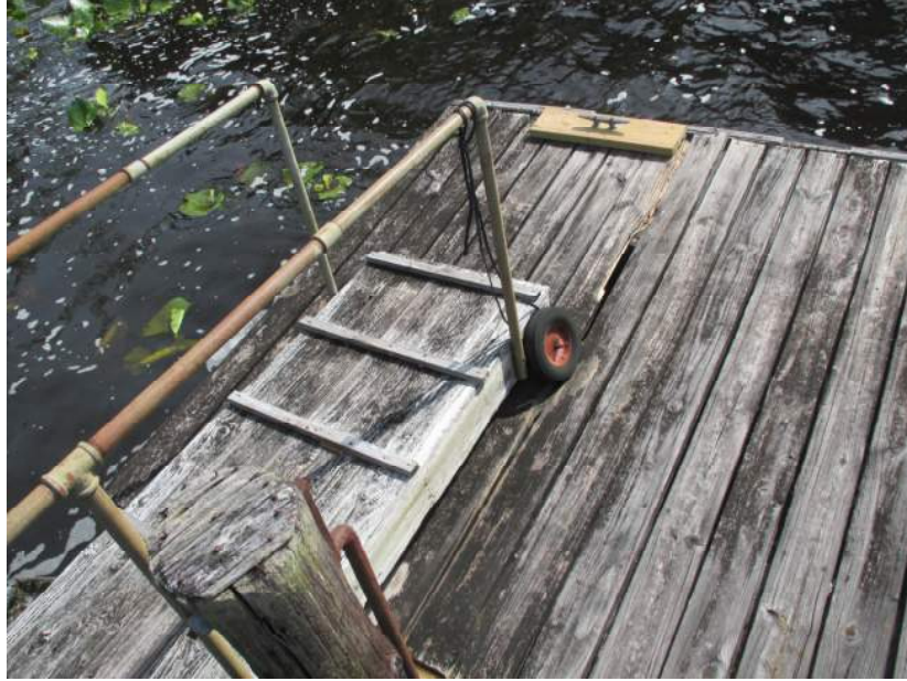
Photograph 9 Deteriorated Decking at Pivot Ramp
