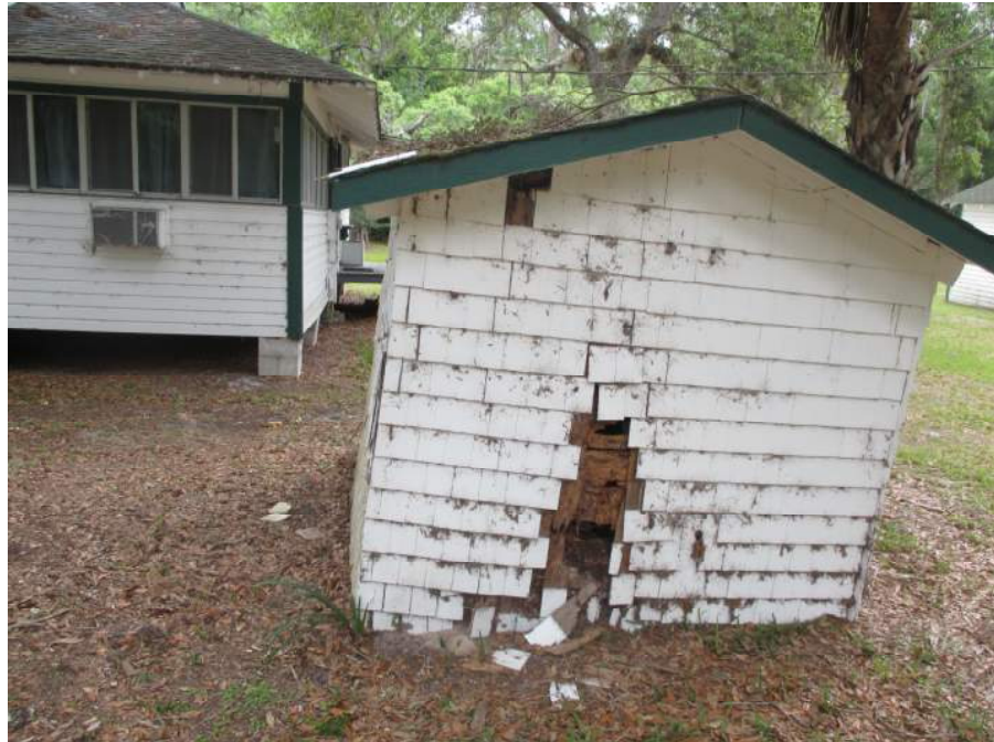
Photograph 6 Settled and Racked Structure
