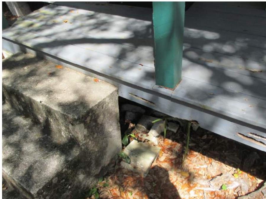
Photograph 19 Collapsed CMU Pier
