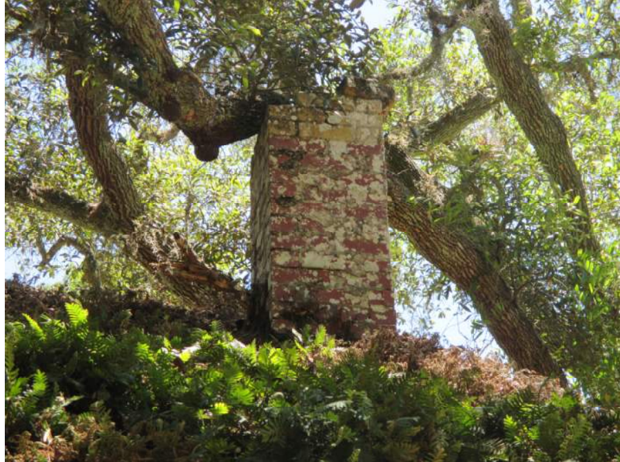
Photograph 12 Tree Bearing on Brick Chimney with Loose Debris
