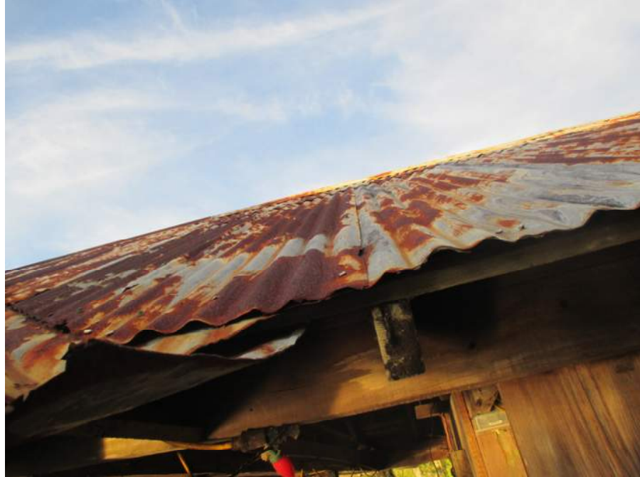
Photograph 3 Surfacial Rust on Metal V-Crimp Roofing
