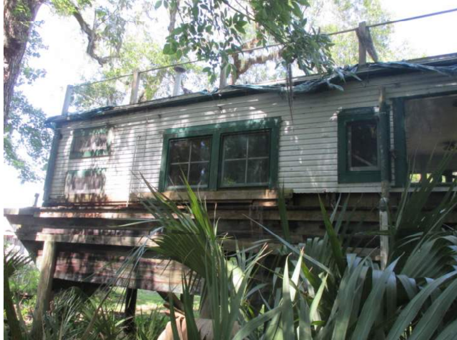
Photograph 13 Missing and Severely Deteriorated Siding
