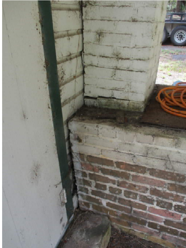
Photograph 3 Chimney to Brick Oven Hinging Masonry
