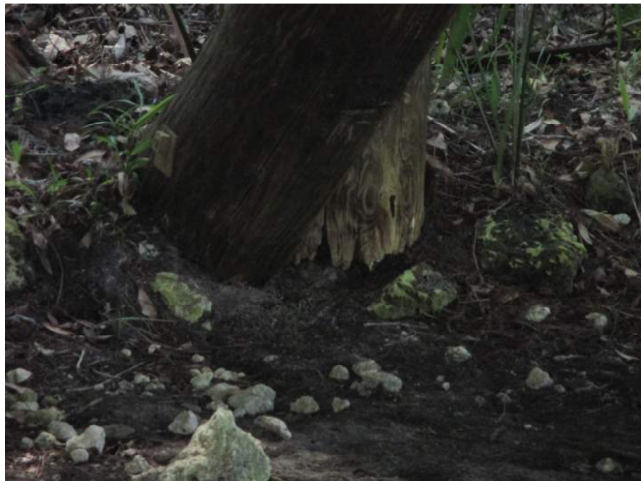
Photograph 14 Base of Houseboat Supports Deteriorated
