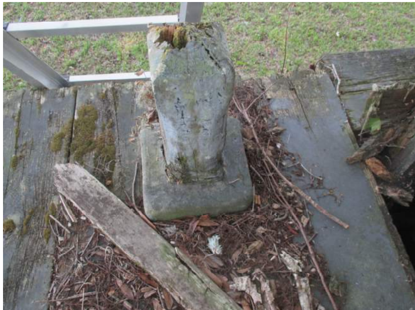
Photograph 9 Mooring Davit Deteriorated
