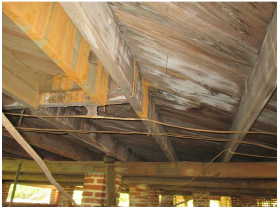
Photograph 13 Water Damaged Floor Decking
