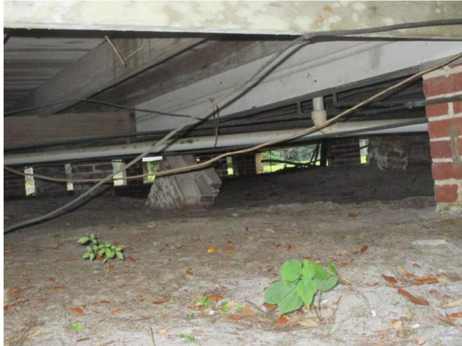
Photograph 16 Rotated and Settled Foundation Piers
