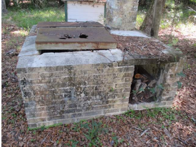
Photograph 4 Settling of Northwest Corner
