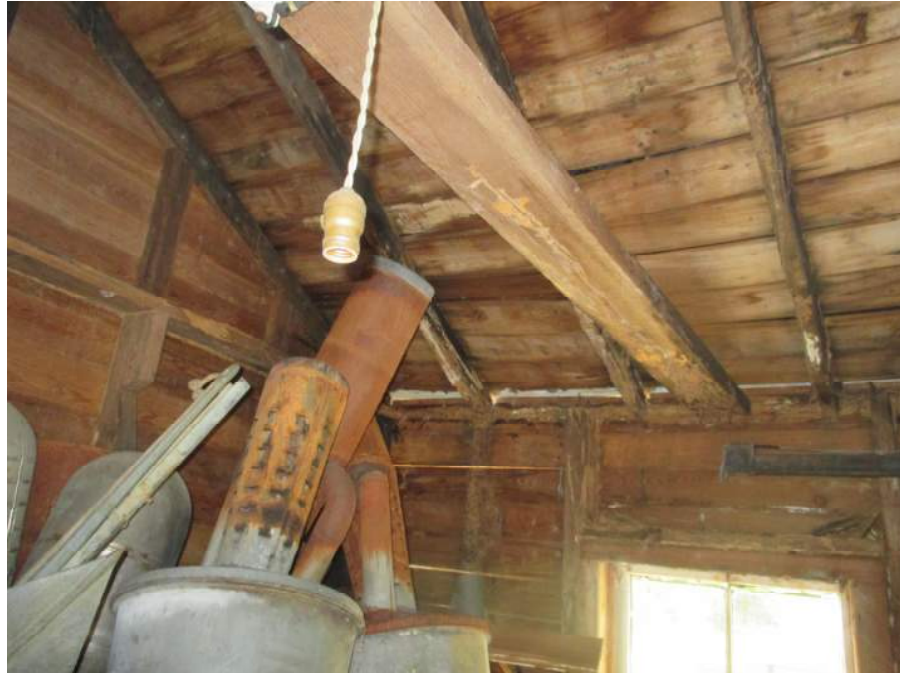
Photograph 5 Severely Deteriorated Wall and Roof Framing
