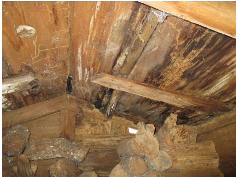
Photograph 2 Severely Deteriorated Roof Framing, Roof and Wall Sheathing
