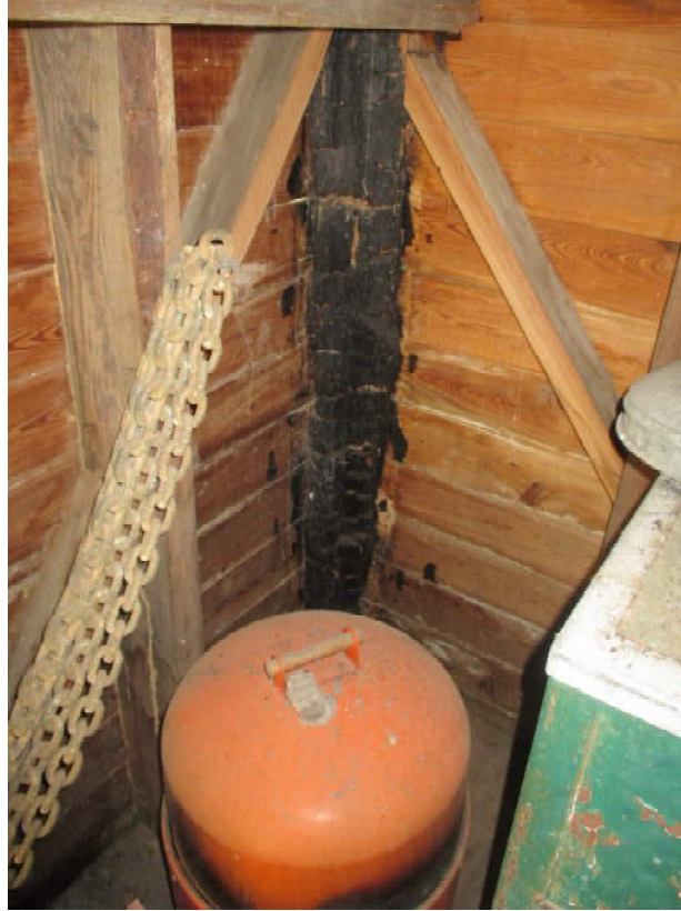
Photograph 9 Charred and Termite Damaged Column
