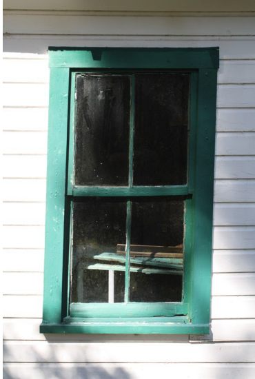
Fryer Shed window with deterioration.
