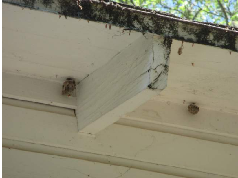
Photograph 4 Deteriorated Rafter Tail
