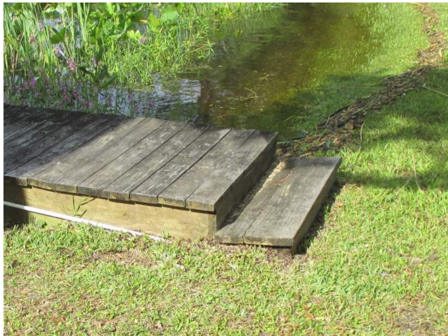
Photograph 14 Settled Entry Step
