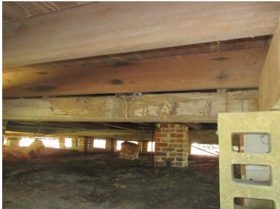
Photograph 15 Rotated and Settled Foundation Piers
