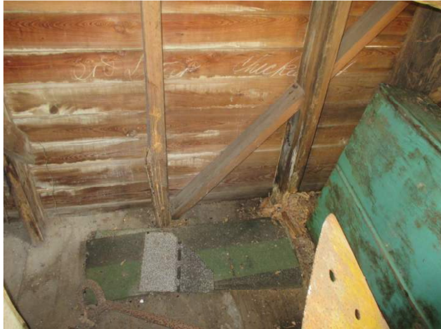
Photograph 11 Severely Deteriorated Wall Framing
