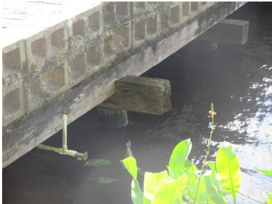
Photograph 2 Deteriorated Beam End Cantilevered Over Timber Pile
