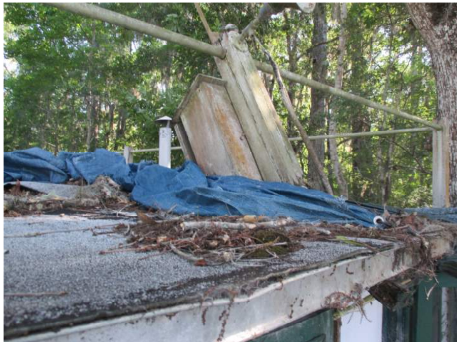
Photograph 12 Handrail Post Failed with Broken Handrail
