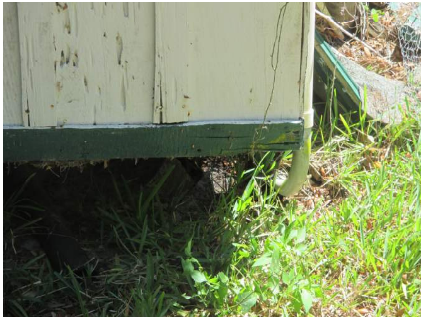
Photograph 13 Failed Corner Foundation
