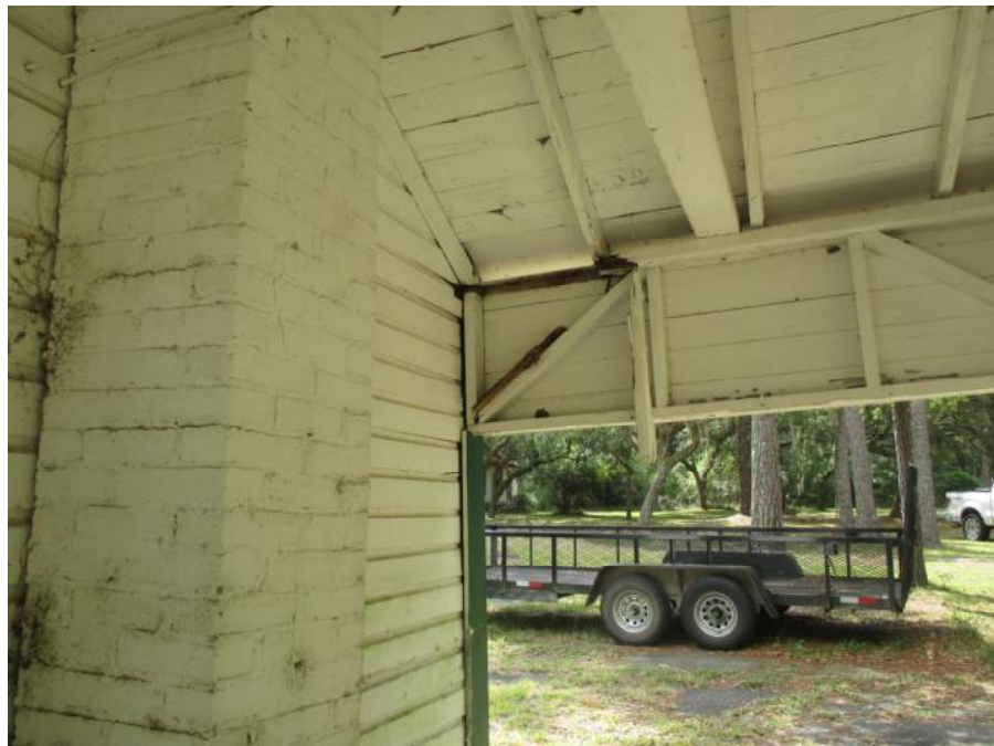
Photograph 14 Deteriorated Porch Framing
