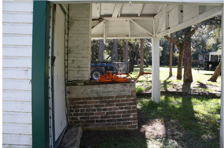
Fryer Shed base has dropped at the building.
