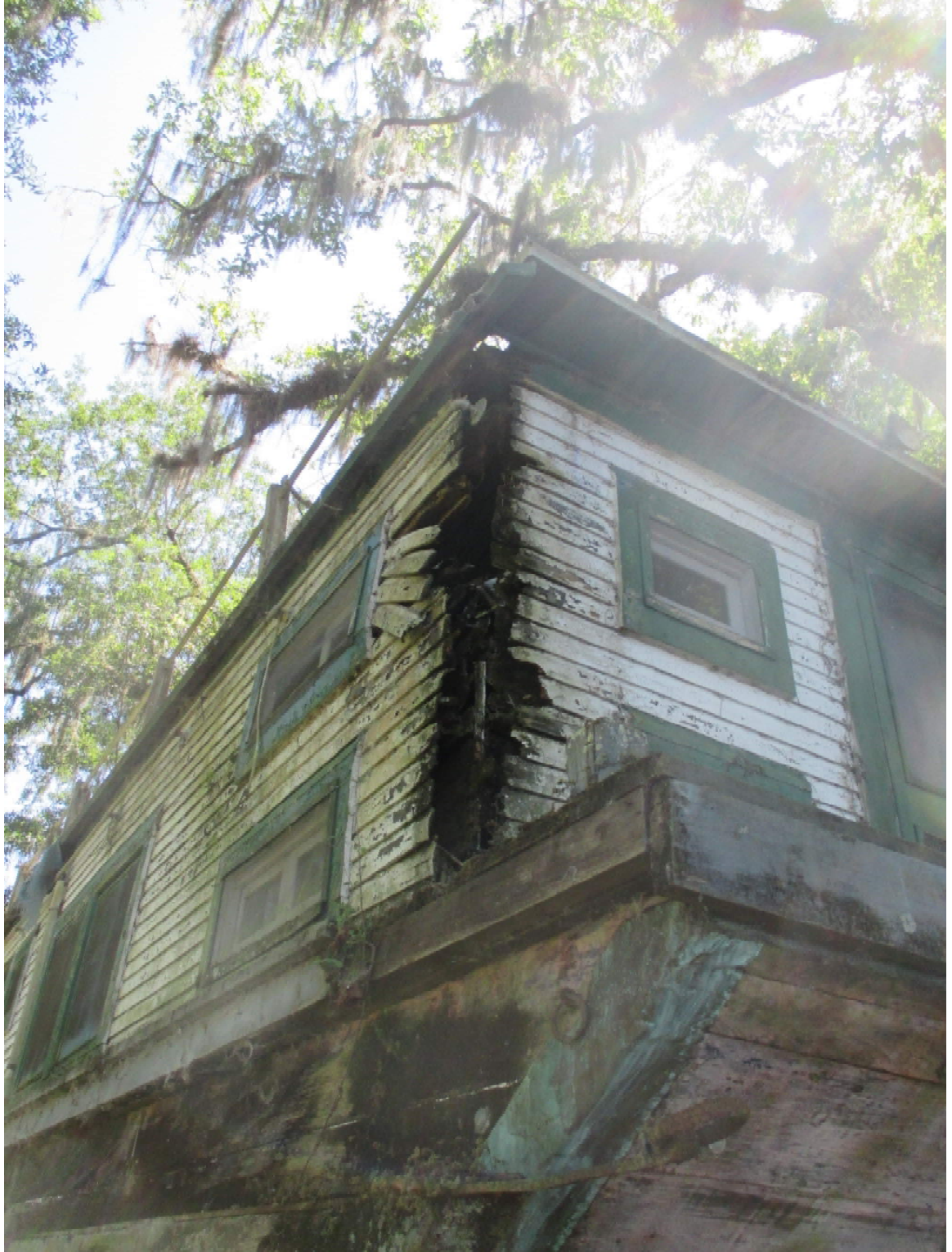
Photograph 3 Northwest Corner Severely Deteriorated
