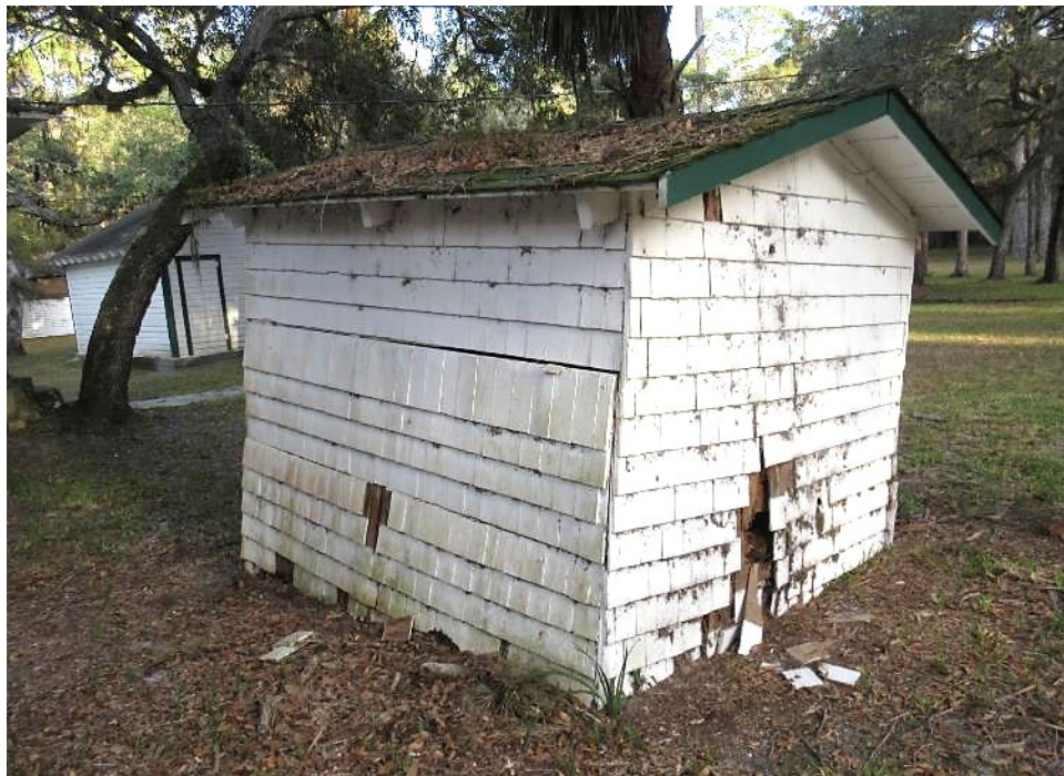
Detail view showing the access panel along the north façade, as well as the termite damage at the rear.
